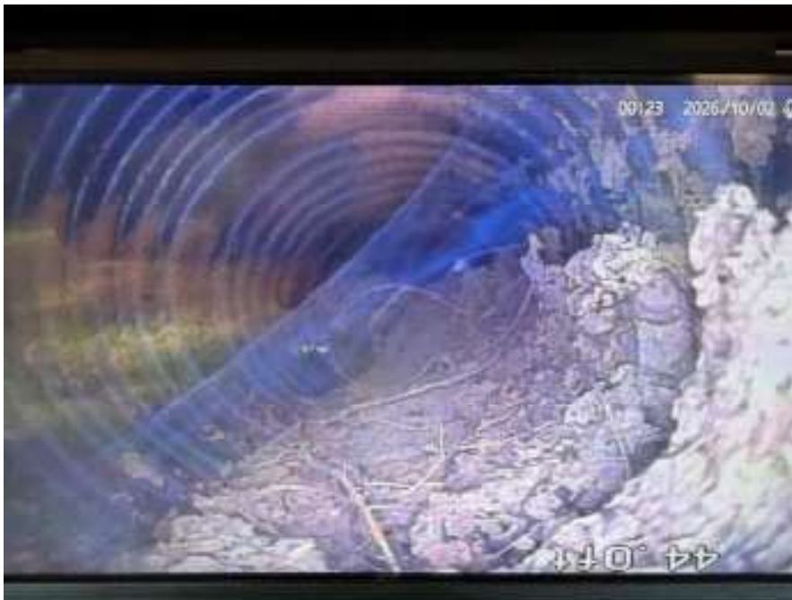
Debris noted inside disposal lines
