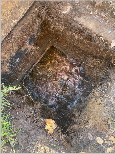
Inlet side of tank.
