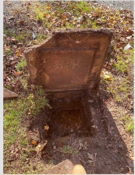
Inlet side of tank showing broken riser lid.
