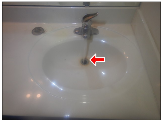
4.4 Item 8(Picture) Missing drain pop-up
