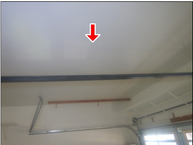
8.2 Item 2(Picture) Loose drywall tape
