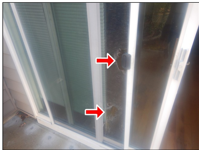
2.1 Item 1(Picture) Holes in screen
