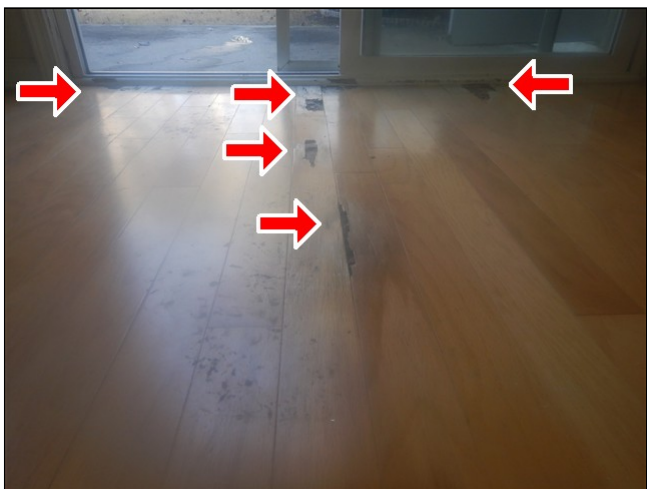
8.3 Item 2(Picture) Close up of damaged hardwood flooring
