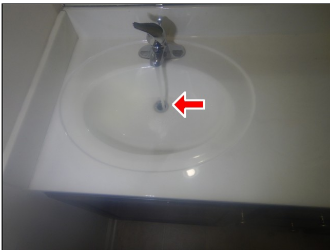
4.4 Item 7(Picture) Missing drain pop-up
