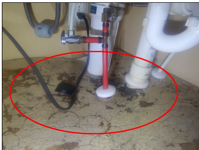
8.4 Item 1(Picture) Sagged and damaged base of cabinet
