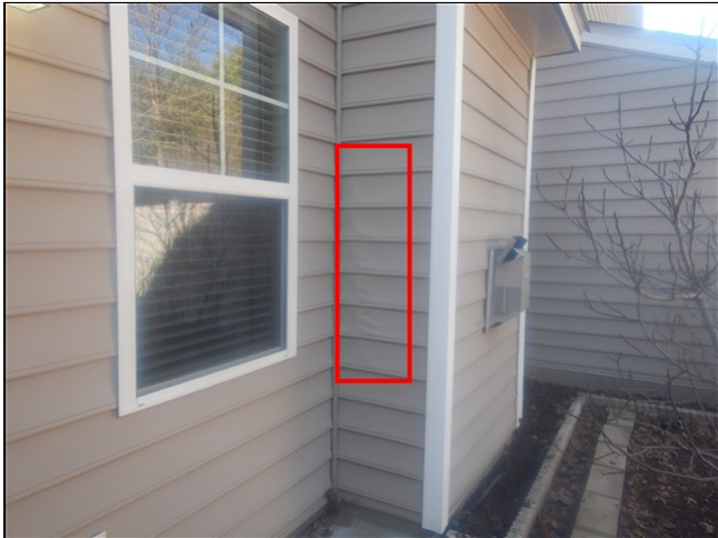
2.0 Item 1(Picture) Deformed vinyl siding
