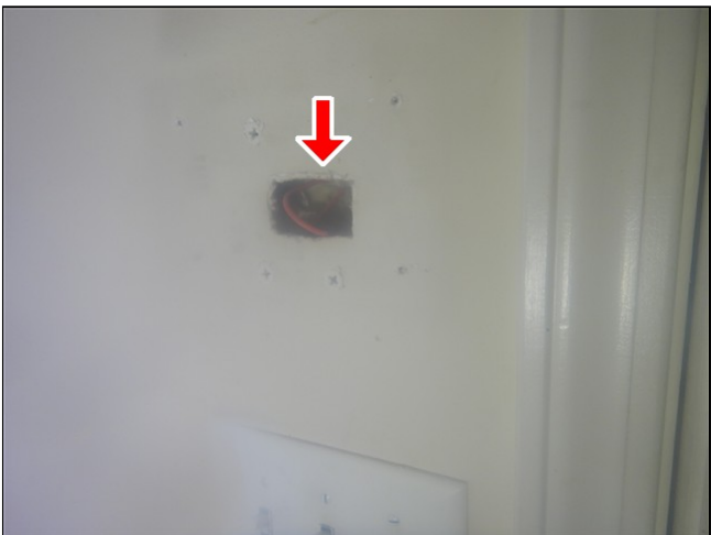
8.1 Item 4(Picture) Close up of hole in drywall
