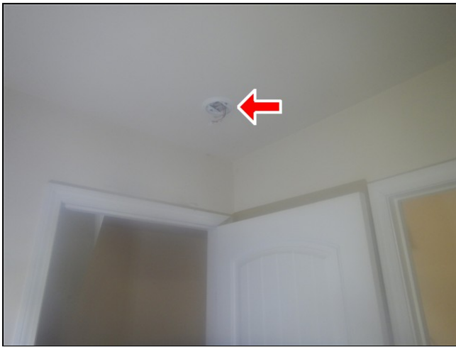
5.6 Item 1(Picture) Missing cartridge
