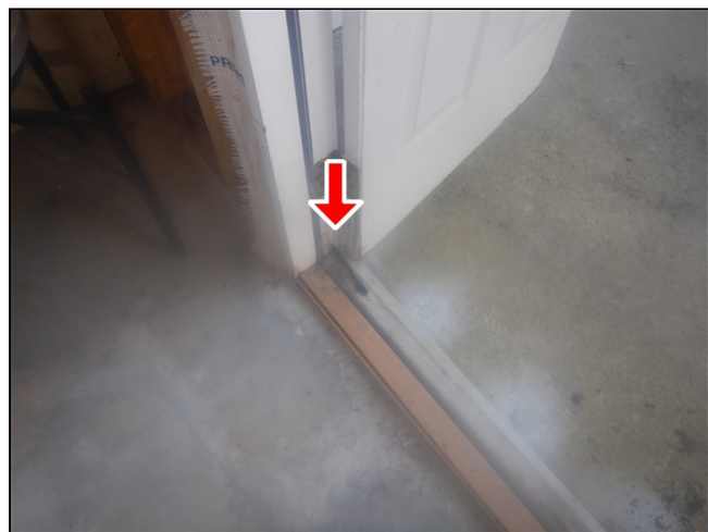
2.1 Item 2(Picture) Water damaged wood
