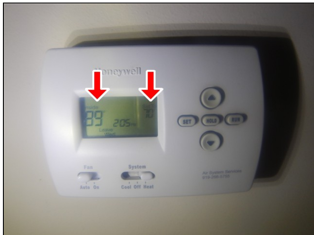
6.1 Item 1(Picture) 2nd floor thermostat in heat mode with interior temperature of 89 degrees and requested temperature of 70 degrees
