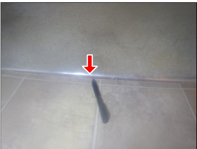
8.3 Item 6(Picture) Close up of vinyl flooring not extending to threshold
