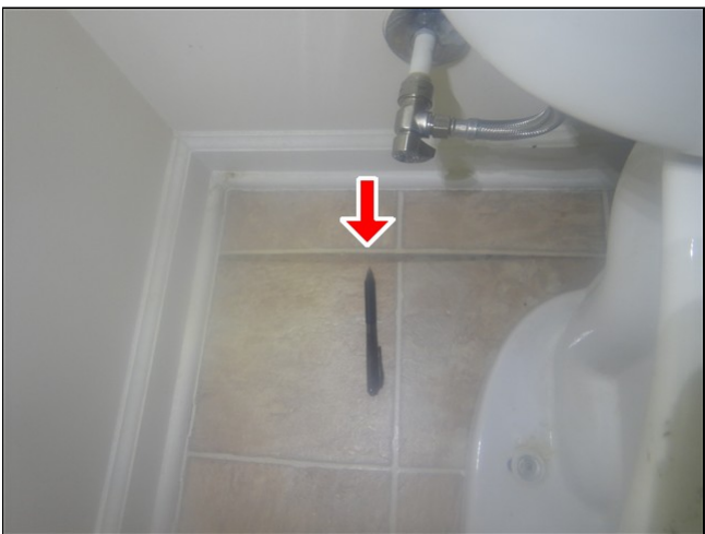
8.3 Item 8(Picture) Close up of separated vinyl flooring
