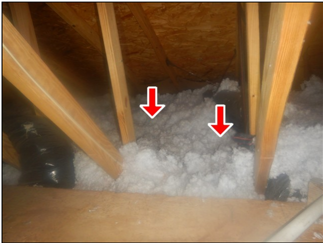
9.0 Item 1(Picture) Low spots in insulation
