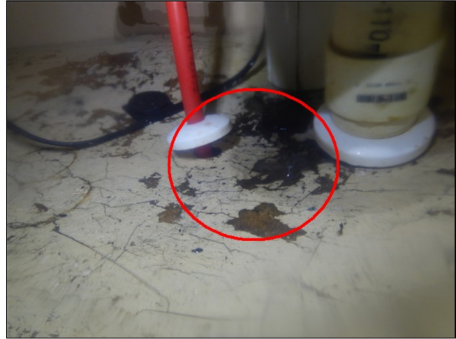
4.4 Item 4(Picture) Puddled water
