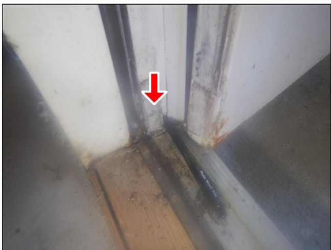
2.1 Item 3(Picture) Close up of water damaged wood
