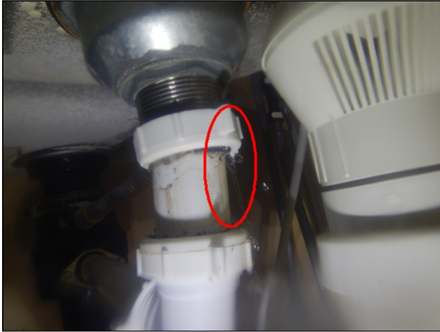
4.4 Item 3(Picture) Leak at rear half of kitchen sink
