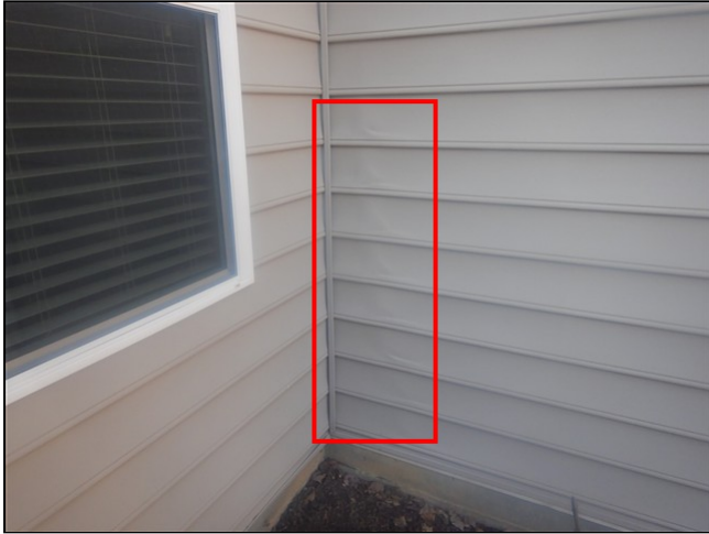
2.0 Item 3(Picture) Deformed vinyl siding
