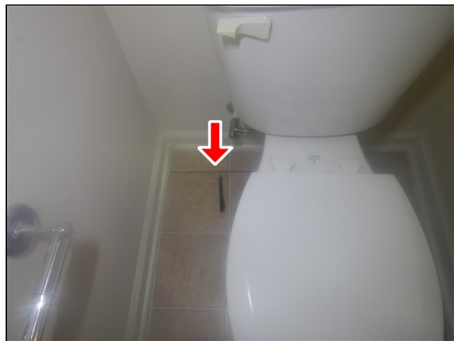
8.3 Item 7(Picture) Separated vinyl flooring
