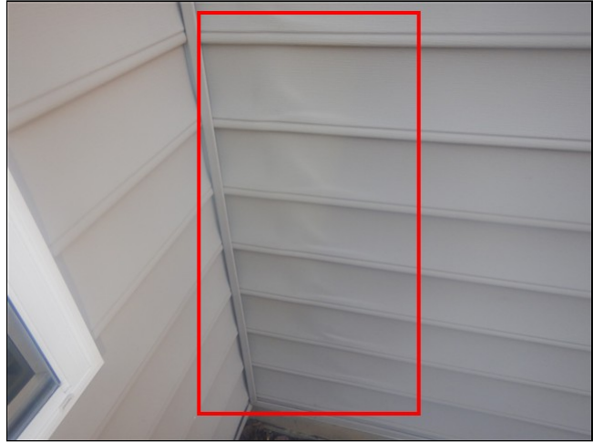
2.0 Item 4(Picture) Close up of deformed vinyl siding
