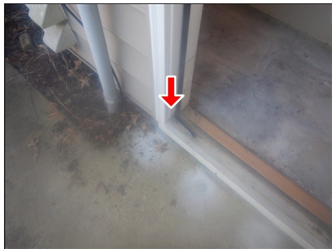
2.1 Item 4(Picture) Water damaged wood
