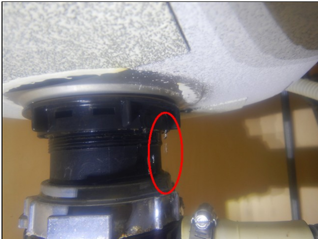
4.4 Item 1(Picture) Leak at disposal side of kitchen sink
