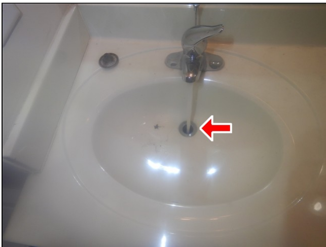
4.4 Item 5(Picture) Missing drain pop-up
