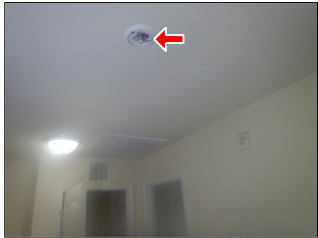
5.6 Item 2(Picture) Missing cartridge
