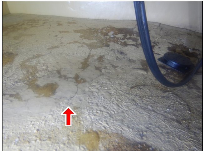
4.4 Item 2(Picture) Puddled water
