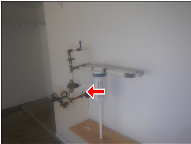
4.2 Item 1(Picture) Main water shut off valve
