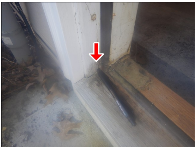
2.1 Item 5(Picture) Close up of water damaged wood
