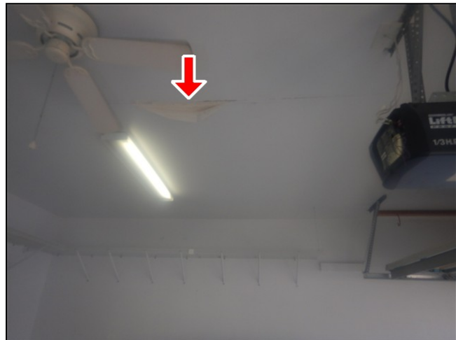
8.2 Item 1(Picture) Loose drywall tape
