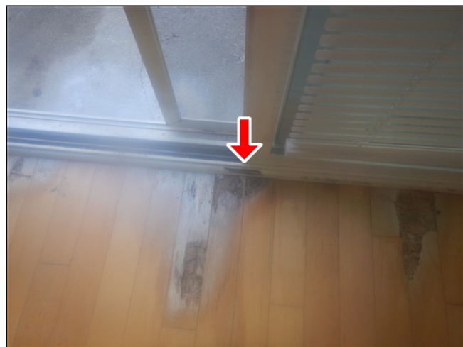
8.3 Item 3(Picture) Damaged quarter round molding
