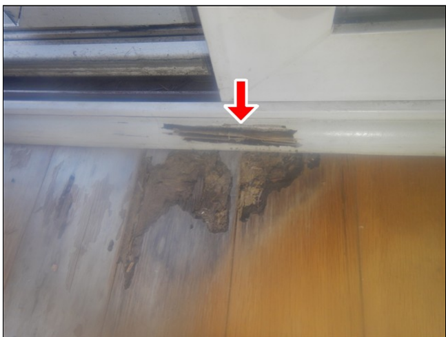
8.3 Item 4(Picture) Close up of damaged quarter round molding
