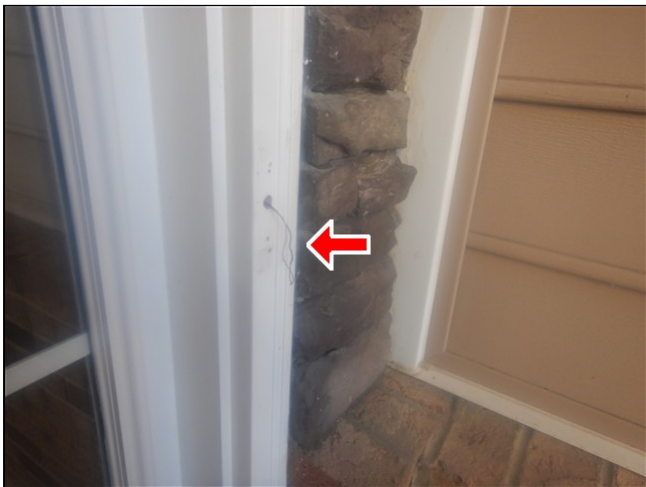
5.3 Item 1(Picture) Missing doorbell
