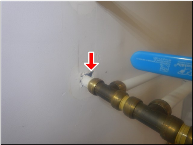
8.1 Item 2(Picture) Close up of hole in garage drywall
