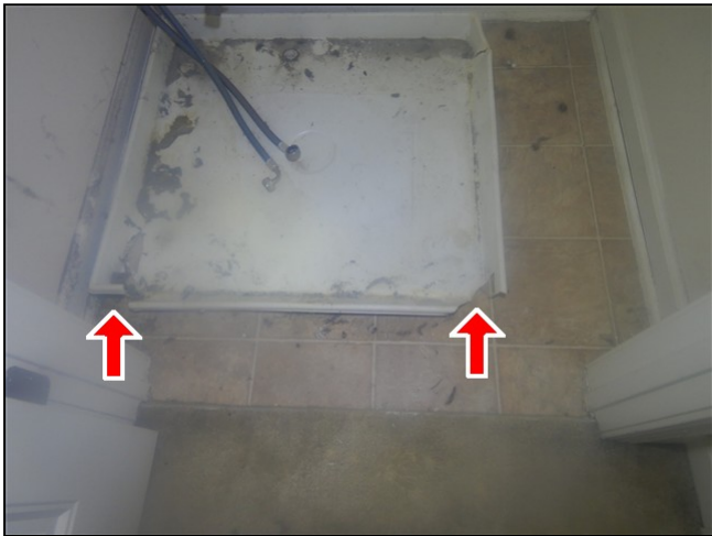
4.0 Item 1(Picture) Damaged overflow pan
