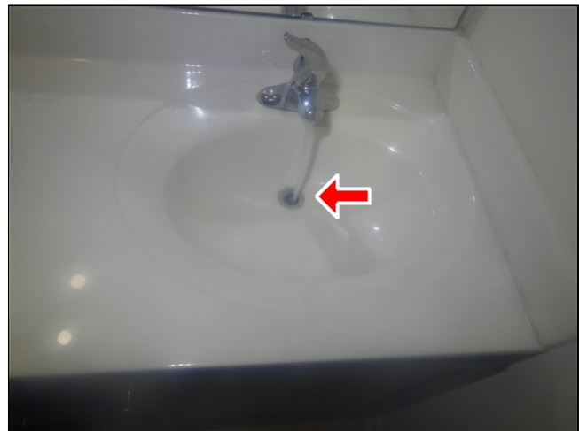
4.4 Item 6(Picture) Missing drain pop-up
