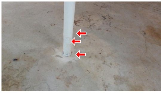
Rust damaged columns in the basement
