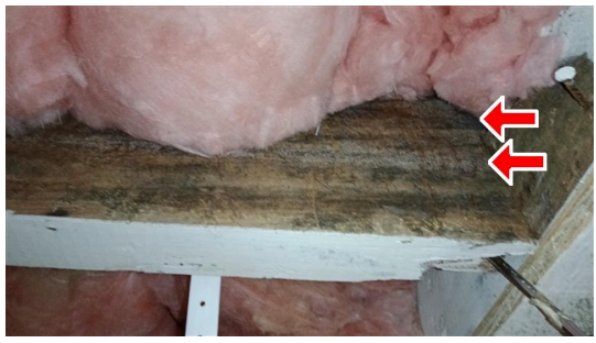
Fungal growth noted on the floor framing
