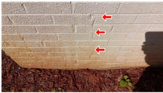
Cracking with repairs that has been painted
