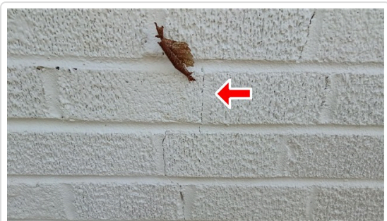
Cracking with repairs that has been painted
