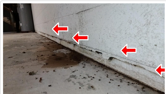
Straight mortar joint cracking where the blocks are pushed in and are hanging off the supporting blocks
