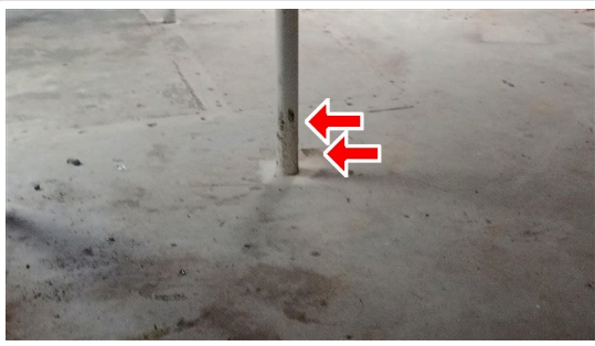
Rust damaged columns in the basement
