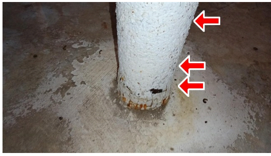
Rust damaged columns in the basement
