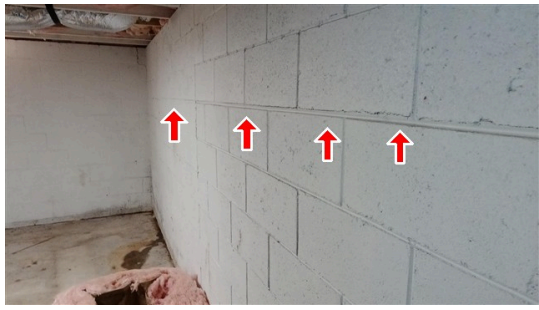
Hydrostatic pressure has caused the wall to bulge and crack
