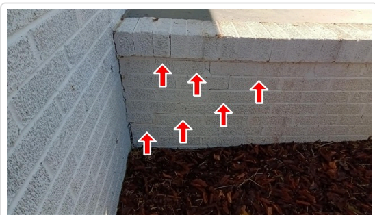
Stair step cracking in the front porch foundation
