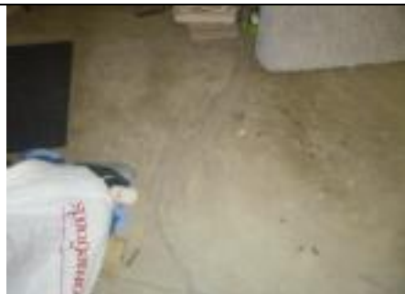
Previous Repairs to Garage Floor
