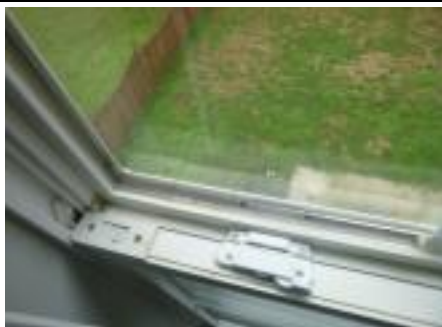
Failed Thermal Seal Window
