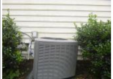
Exterior A/C Unit Out of Level
