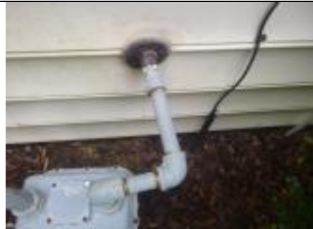
CSST Not Bonded at Gas Meter
