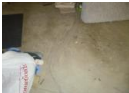
Previous Repairs to Garage Floor
