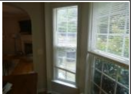
Failed Sash Balance at Bay Window
