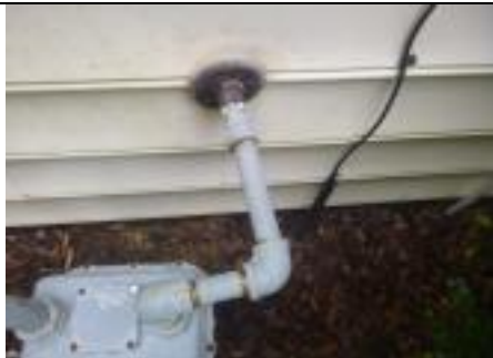
CSST Not Bonded at Gas Meter
