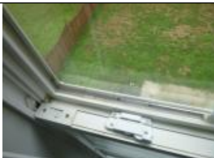
Failed Thermal Seal Window
