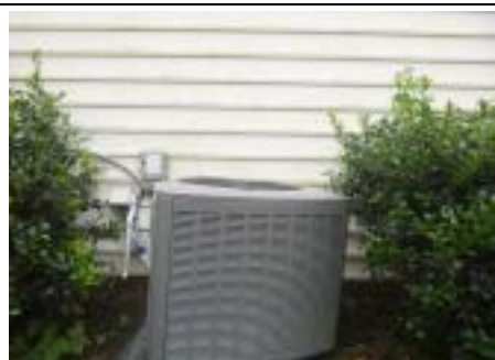
Exterior A/C Unit Out of Level
