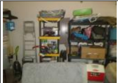
Main Panel Obstructed by Storage
