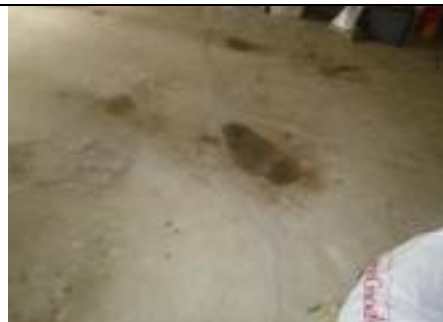
Previous Repairs to Garage Floor
