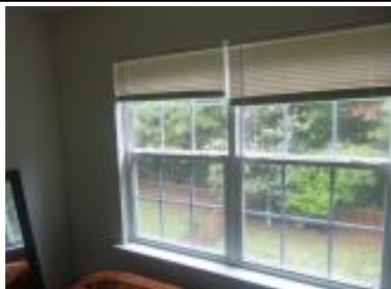
Failed Sash Balance at Bedroom
