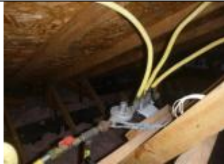
CSST Not Bonded at Gas Manifold
