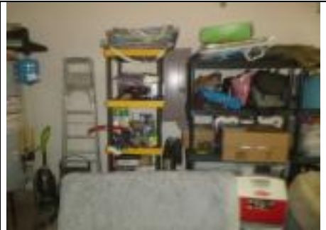
Main Panel Obstructed by Storage
