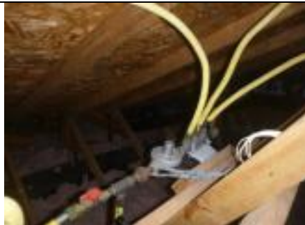
CSST Not Bonded at Gas Manifold
