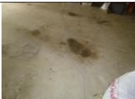
Previous Repairs to Garage Floor
