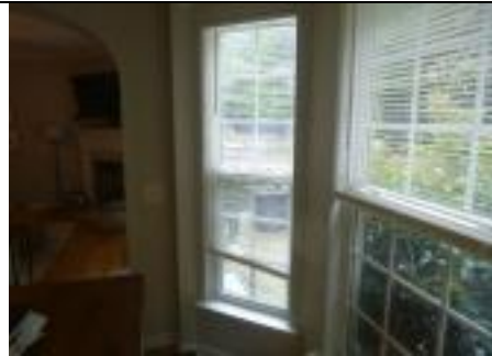
Failed Sash Balance at Bay Window
