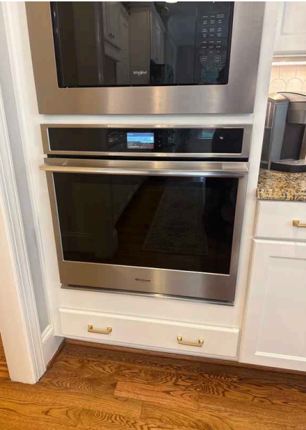
Range/Oven: Photo - Range/Oven Range/Oven: Photo - Oven Pre-Heated Range/Oven
