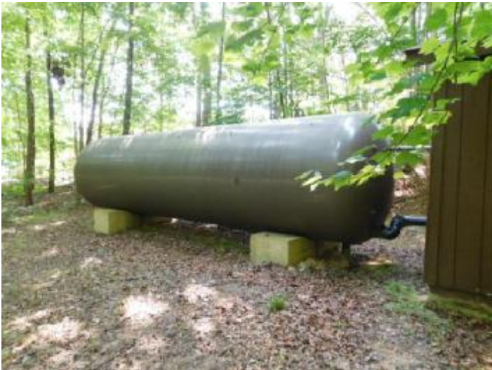
Community well tank
