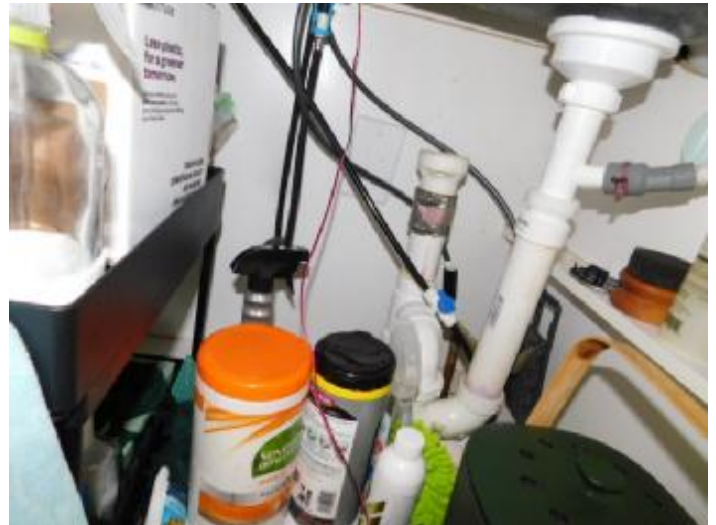
Below kitchen sink
