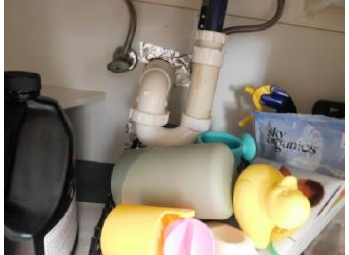
Example of below bathroom sinks
