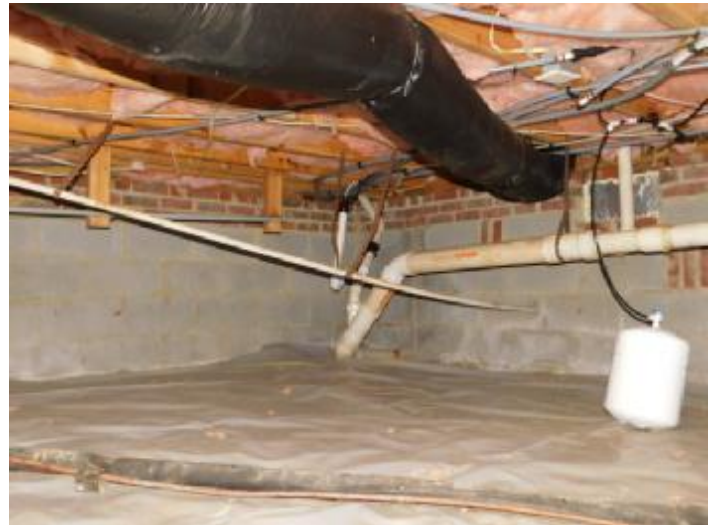
Evidence of past dry moisture at the foundation walls in the crawl space - Example
