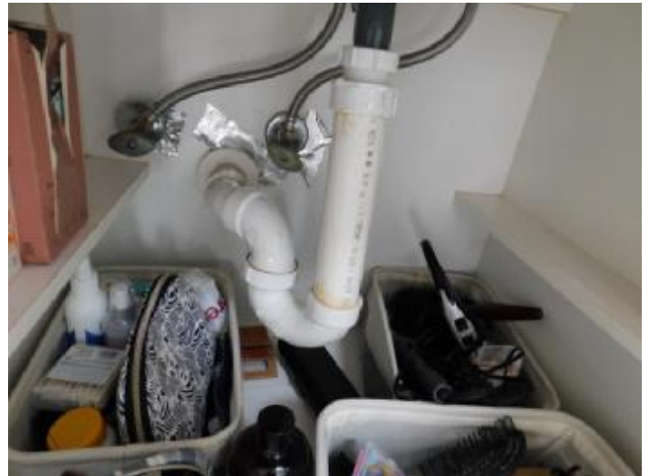
Example of below bathroom sinks
