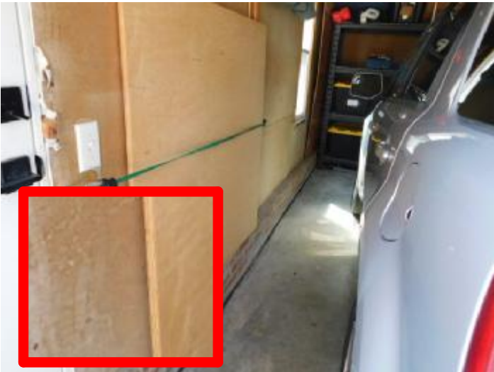
Evidence of past dry moisture at the wall in the garage, past/future performance unknown
