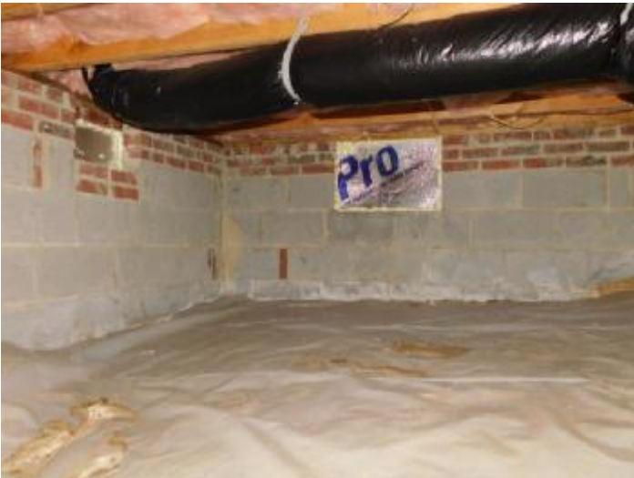
Evidence of past dry moisture at the foundation walls and vapor barrier in the crawl space - Example
