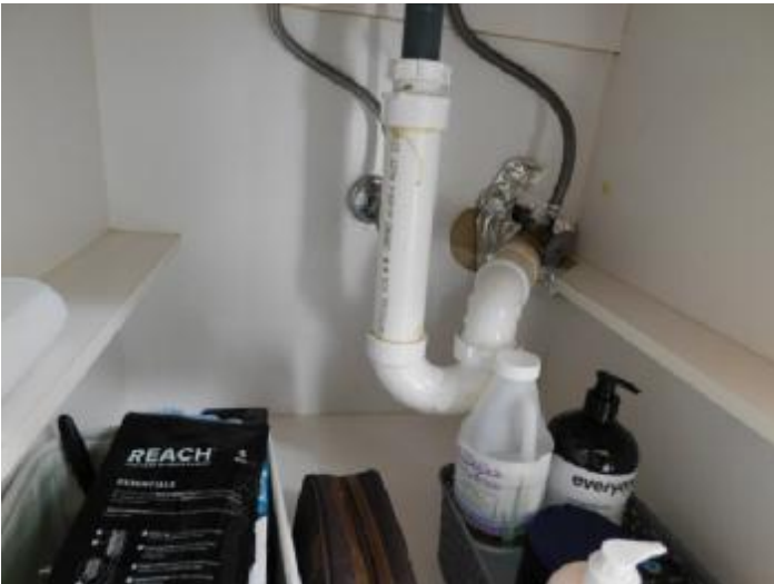
Example of below bathroom sinks
