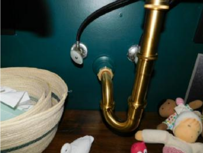
Example of below bathroom sinks
