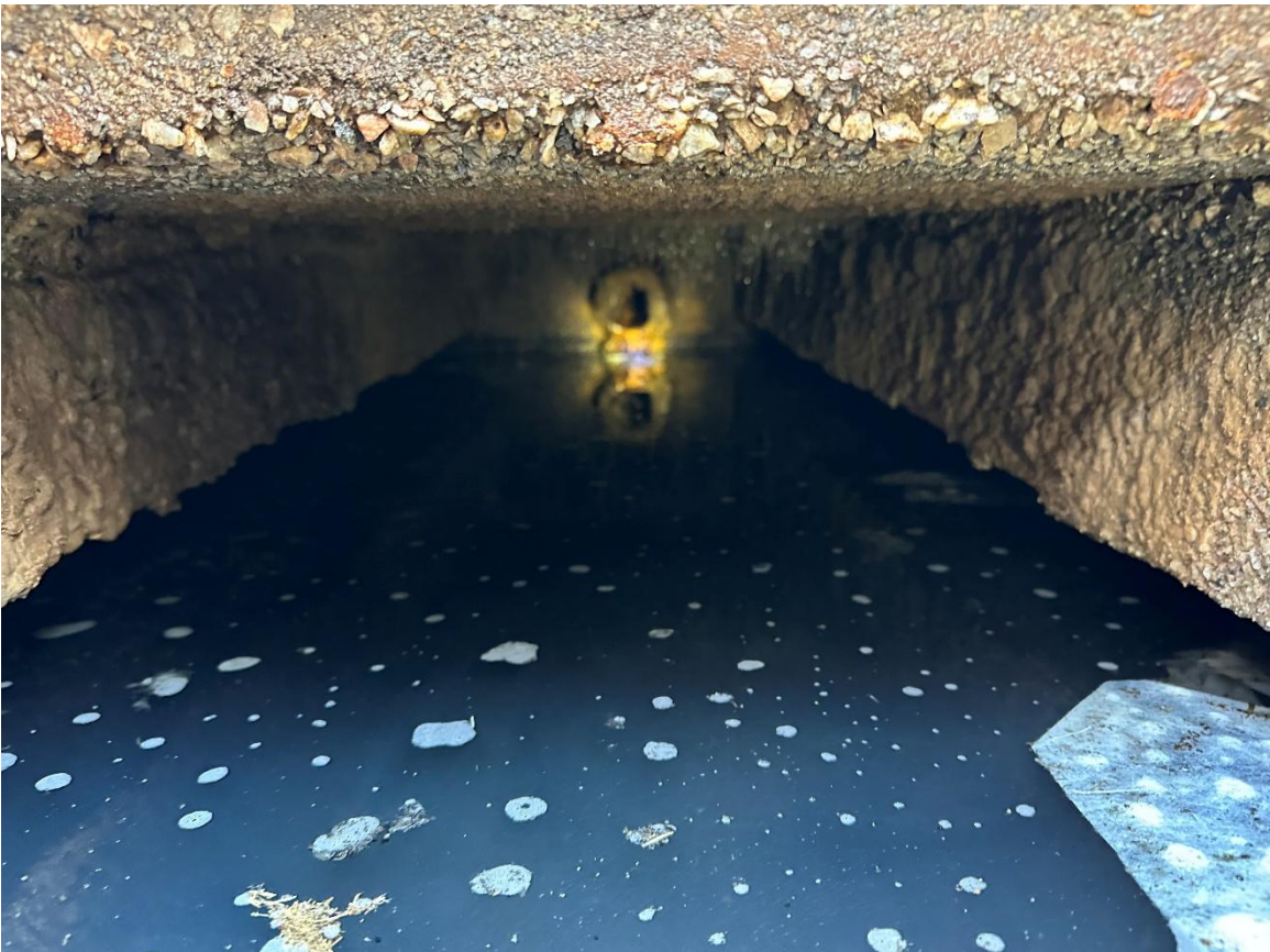
Septic Tank Interior
