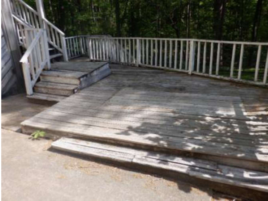
Photograph Number 5 - Rear decks are in poor condition. Remove and rebuild both levels of the deck.
