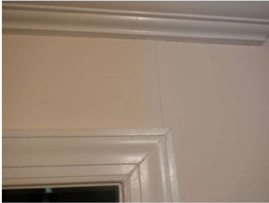
Photograph Number 1 - Example of drywall crack found in isolated areas. Patch and monitor.
