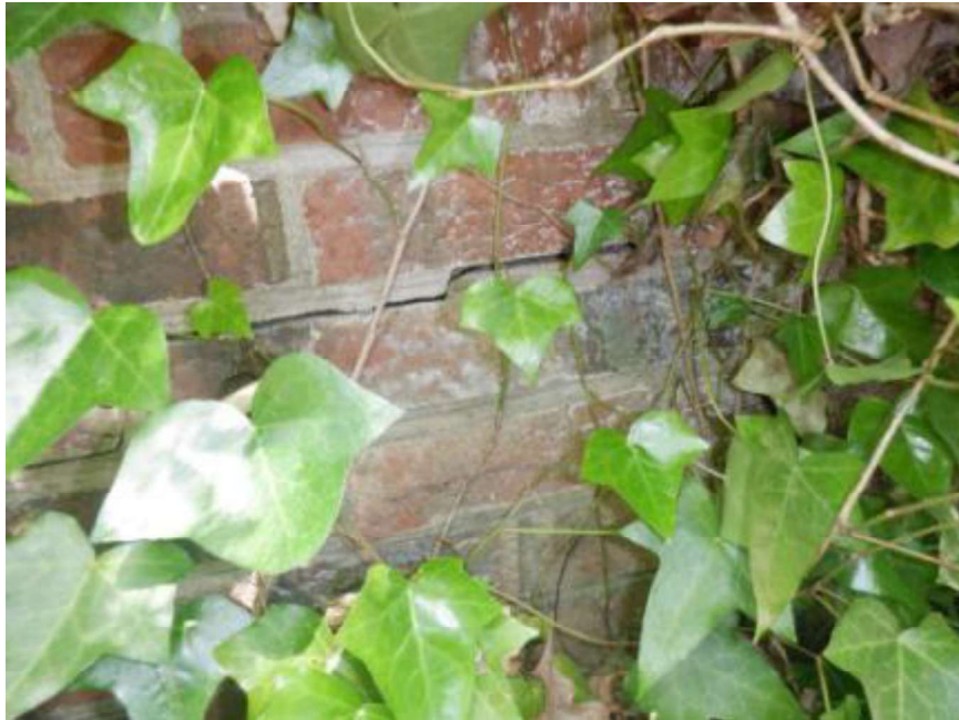
Photograph Number 8 - Cracks in brick retaining wall.
