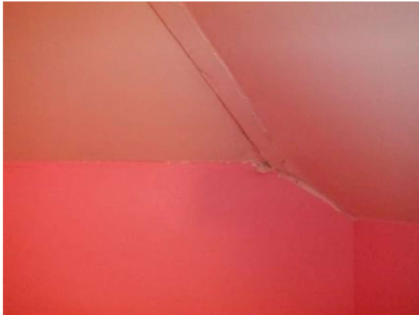
Photograph Number 2 - Separation of drywall in attic. Framing was not present along edge of drywall for properly securing.
