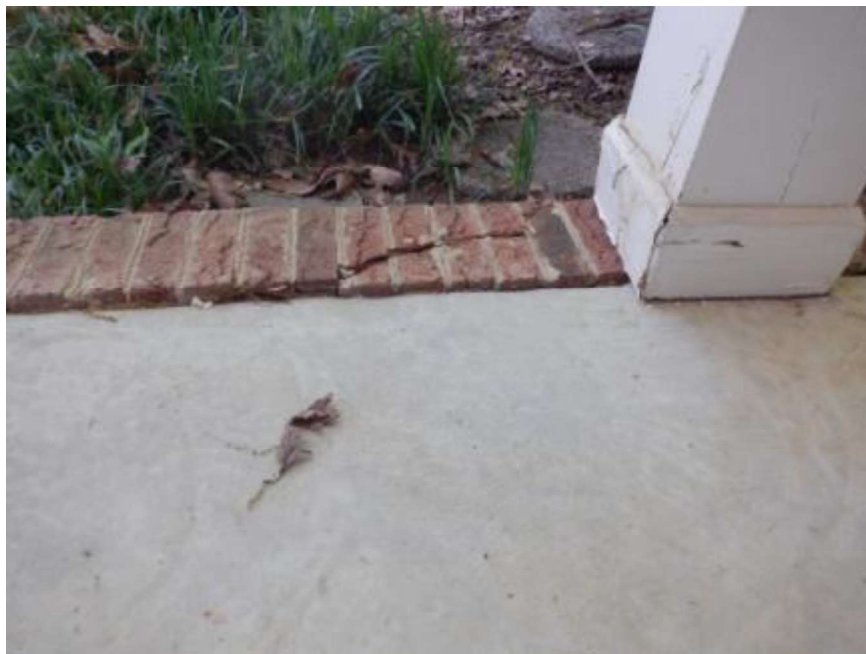
Photograph Number 4 - Brick rowlock rotating to the side of support column. Shim columns and monitor.
