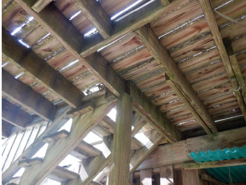
Photograph Number 7 - View of poor deck connections and support details.
