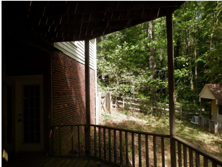
Photograph Number 6 - View of undersized deck posts.
