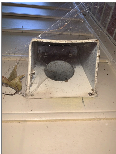
5.4 Item 1(Picture) There is no damper or screen installed at duct hood to rear of chimney
