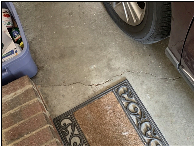
4.2 Item 1(Picture) Minor cracks visible in the garage concrete slab
