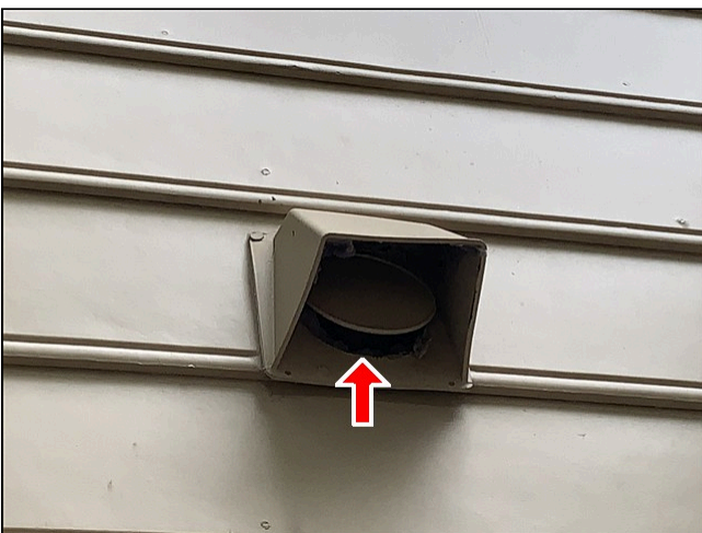
5.4 Item 2(Picture) Damper does not fully close at dryer vent duct hood at rear over deck
