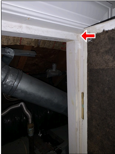
9.2 Item 1(Picture) Weather stripping missing at attic access doors at third floor
