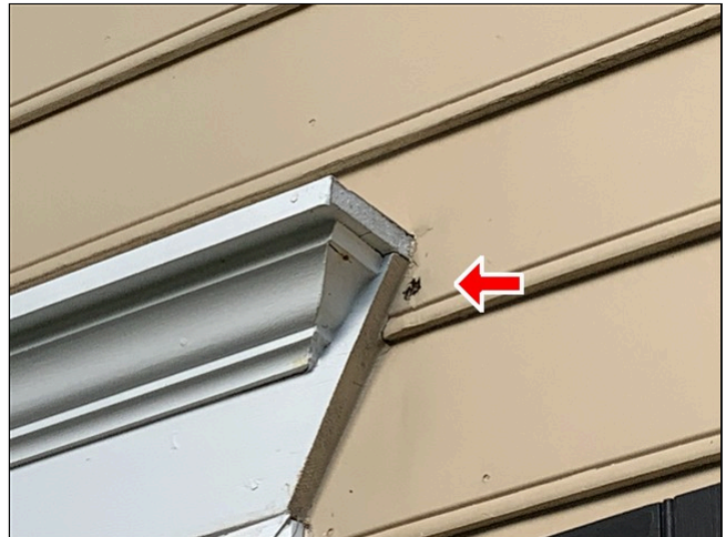
2.1 Item 3(Picture) Hard board siding is deteriorated
