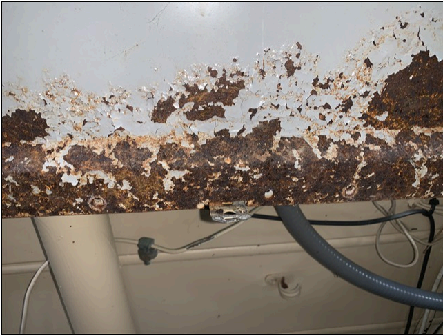
7.1 Item 1(Picture) Base of inner cover is heavily rusted at left side main electric panel
