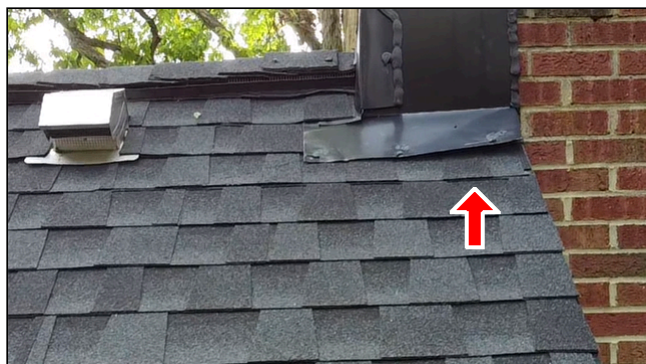
3.1 Item 1(Picture) Flashing is lifted on roof at rear of chimney
