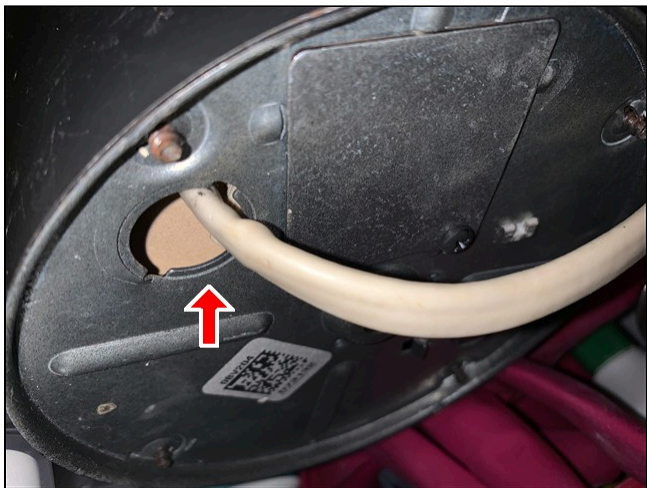
10.2 Item 1(Picture) Wire clamp/bushing missing where electrical wire penetrates base of garbage disposal
