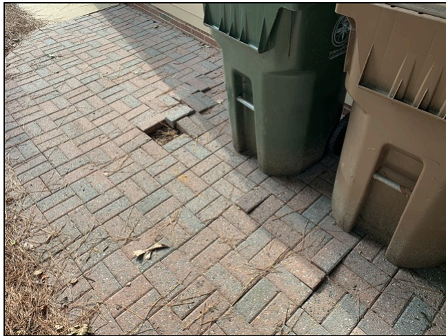
1.1 Item 2(Picture) Right side brick walk is heaved and uneven
