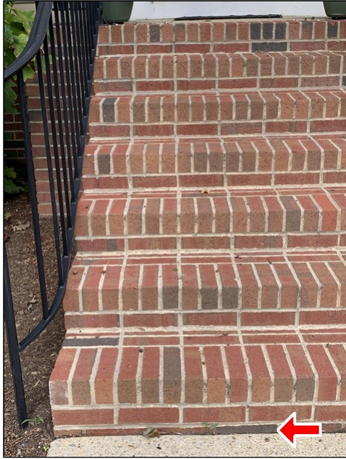
2.6 Item 1(Picture) Riser heights are uneven at front steps
