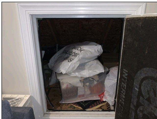
4.6 Item 3(Picture) Stored belongings block full access to some attic areas
