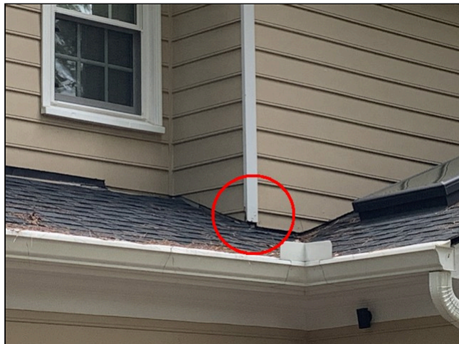
2.2 Item 2(Picture) Trim deteriorated
