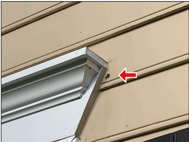
2.1 Item 3(Picture) Hard board siding is deteriorated
