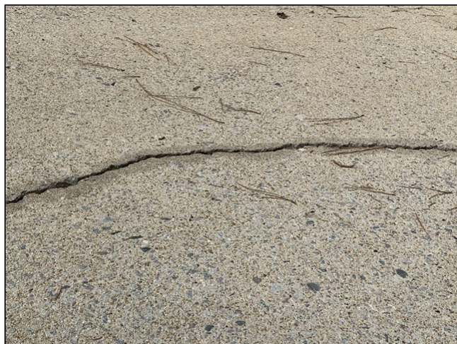
1.0 Item 1(Picture) The driveway has cracked and heaved
