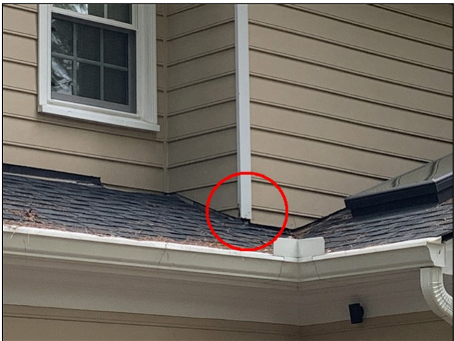
2.2 Item 2(Picture) Trim deteriorated
