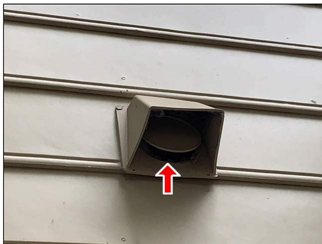
5.4 Item 2(Picture) Damper does not fully close at dryer vent duct hood at rear over deck
