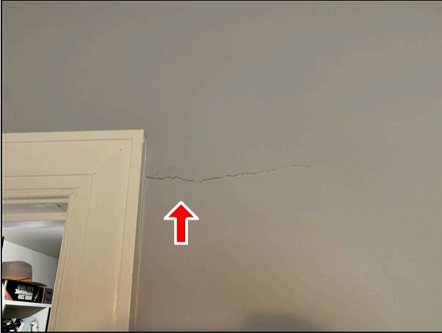
9.0 Item 2(Picture) Minor crack(s) visible in wall sheathing at right top of master bedroom closet door
