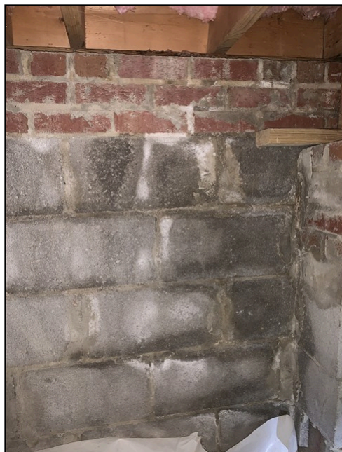
4.5 Item 1(Picture) Signs of minor water penetration visible in the crawlspace at left front (efflorescence on foundation wall)
