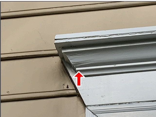
2.2 Item 1(Picture) Trim deteriorated
