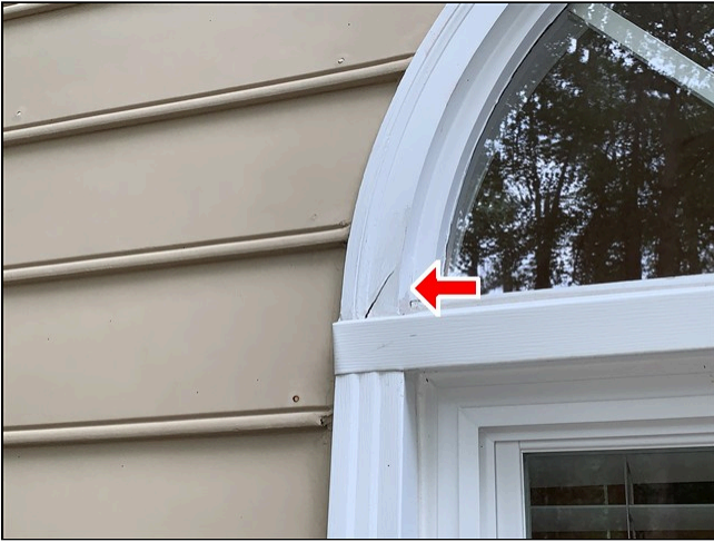
2.2 Item 3(Picture) Trim deteriorated
