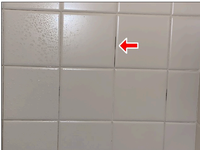
9.0 Item 1(Picture) Gaps visible between some wall tiles at the third floor bathroom shower
