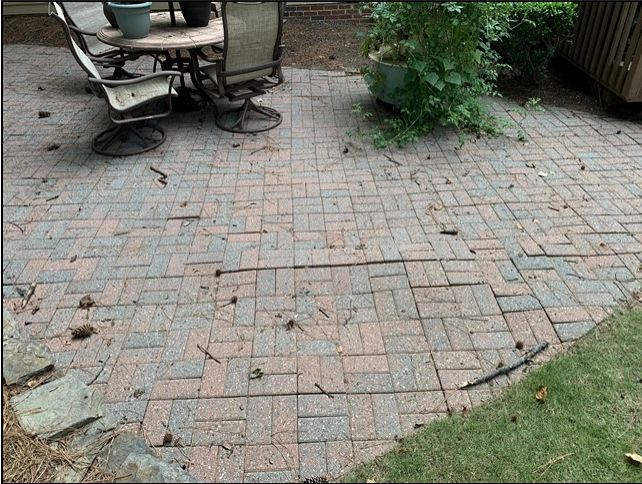
2.9 Item 1(Picture) Rear brick patio is uneven
