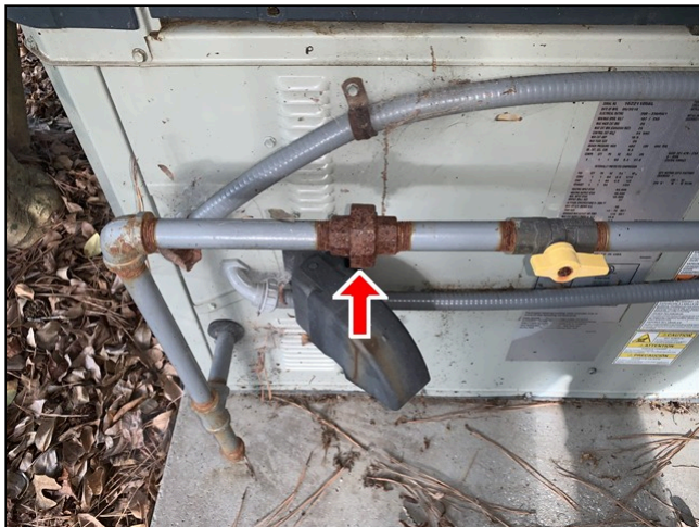
8.3 Item 1(Picture) Gas line rusted near left side gas pack
