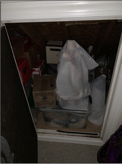
4.6 Item 4(Picture) Stored belongings block full access to some attic areas
