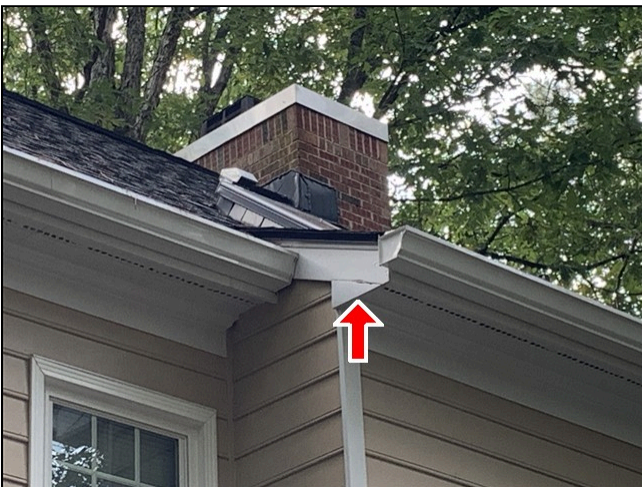
2.2 Item 5(Picture) Rake deteriorated
