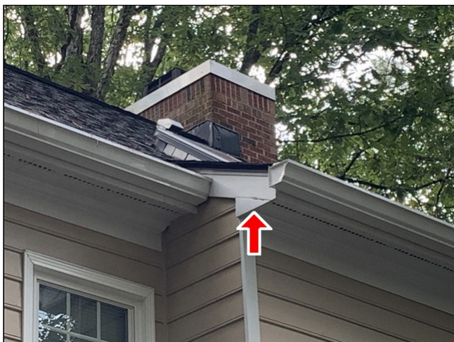
2.2 Item 5(Picture) Rake deteriorated
