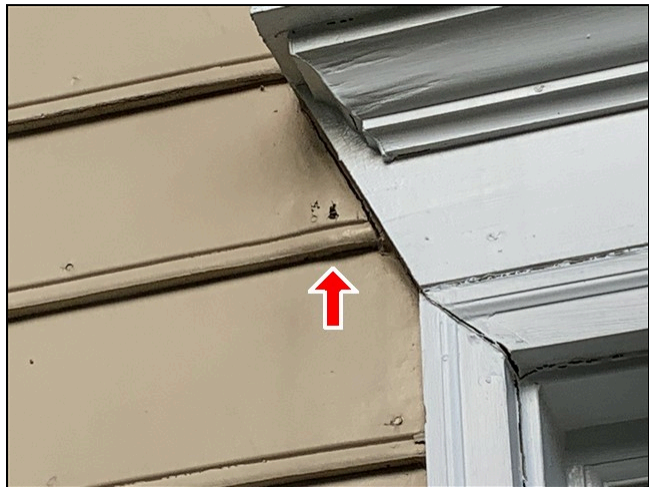
2.1 Item 2(Picture) Hard board siding is deteriorated
