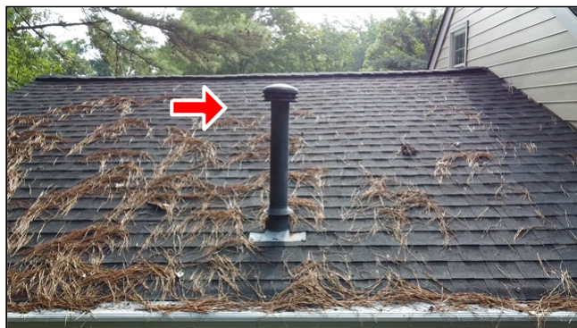
6.7 Item 1(Picture) Water heater flue is leaning on left rear roof (viewed from rear)
