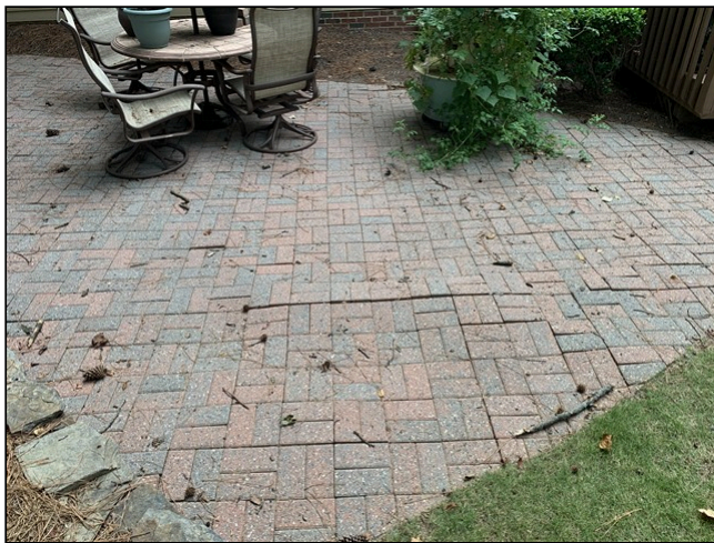
2.9 Item 1(Picture) Rear brick patio is uneven
