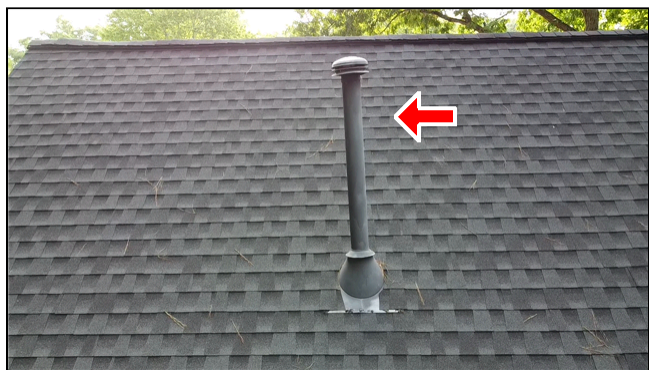
8.0 Item 1(Picture) Furnace flue is leaning on rear upper roof
