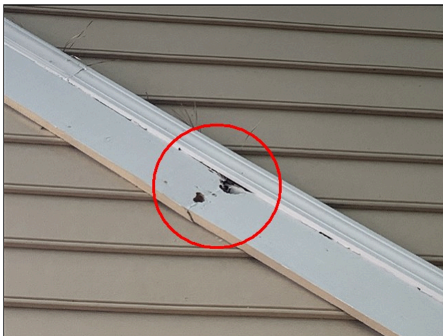
2.2 Item 4(Picture) Trim deteriorated
