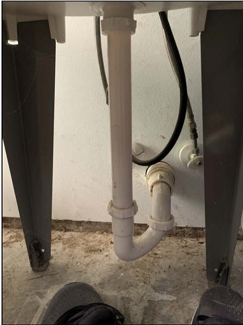
6.0 Item 1(Picture) Water lines and drain trap not insulated at garage sink
