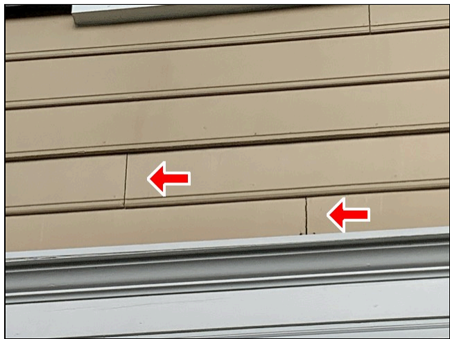
2.1 Item 1(Picture) Gaps are visible at joints between sections of hard board siding in several areas around house
