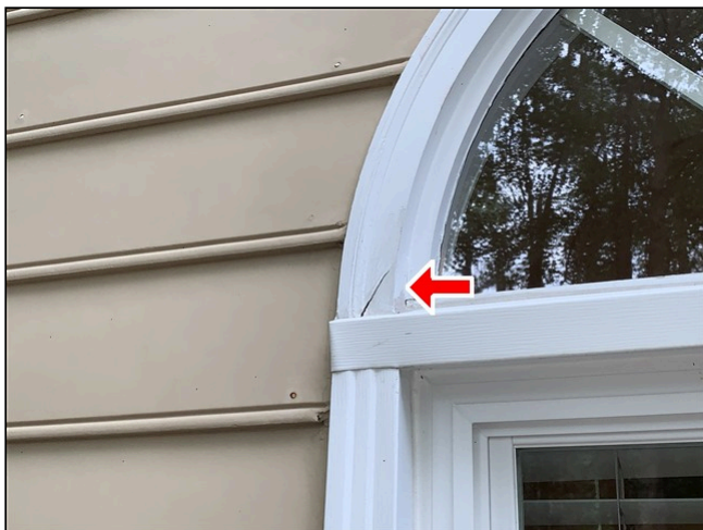
2.2 Item 3(Picture) Trim deteriorated
