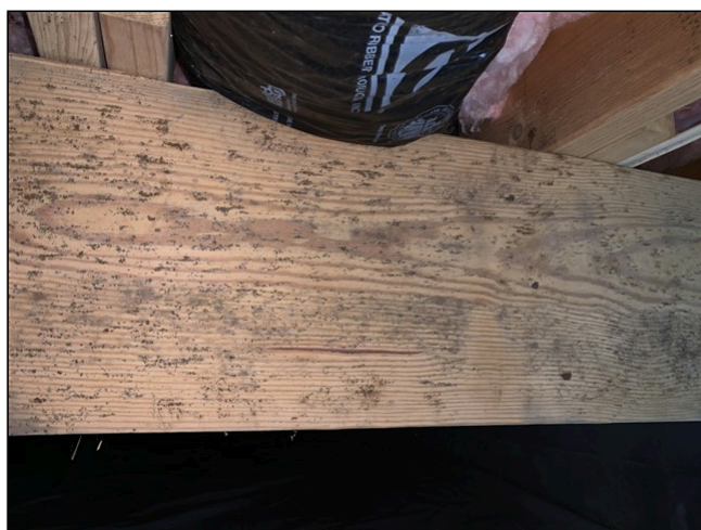
4.6 Item 1(Picture) Light fungus growth visible on main left to right girder at right front of crawlspace
