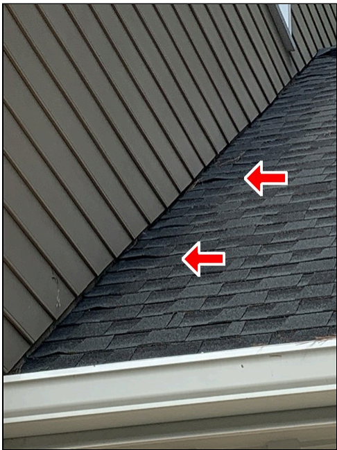
3.0 Item 1(Picture) Lifted shingles visible at left edge of right front lower roof
