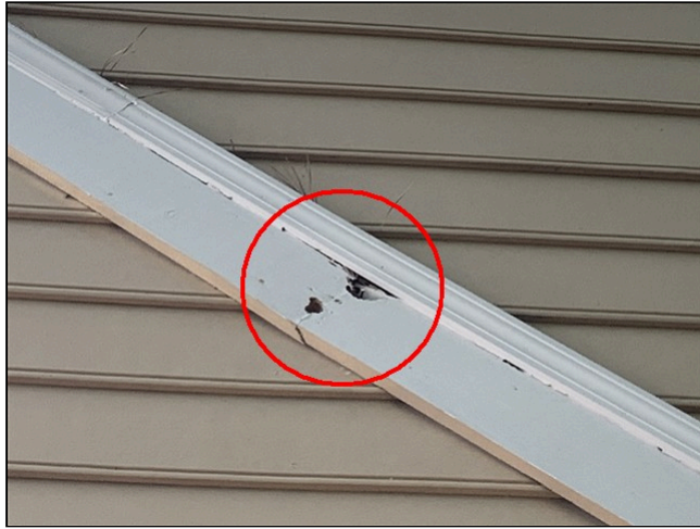
2.2 Item 4(Picture) Trim deteriorated
