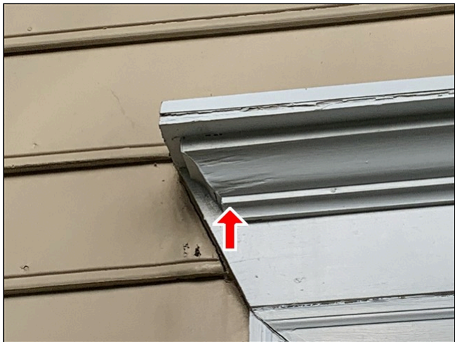
2.2 Item 1(Picture) Trim deteriorated
