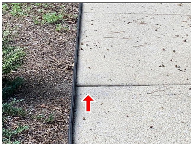
1.1 Item 1(Picture) The front concrete walk has cracked and heaved
