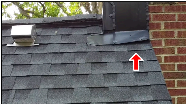
3.1 Item 1(Picture) Flashing is lifted on roof at rear of chimney
