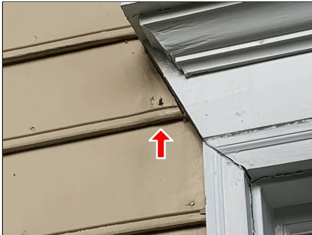
2.1 Item 2(Picture) Hard board siding is deteriorated
