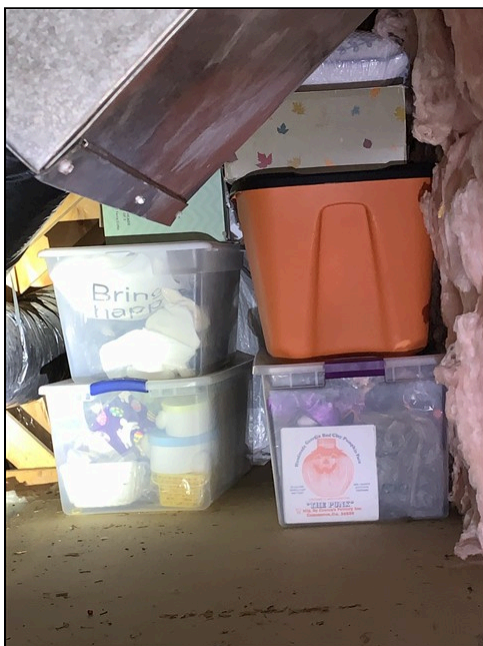
4.6 Item 2(Picture) Stored belongings block full access to some attic areas
