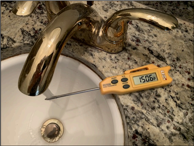
6.7 Item 2(Picture) Water temperature over 150°F. when measured at the half bathroom sink
