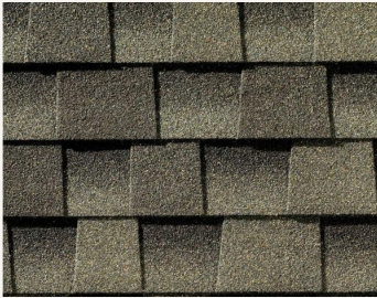
Roof: Weathered Wood
