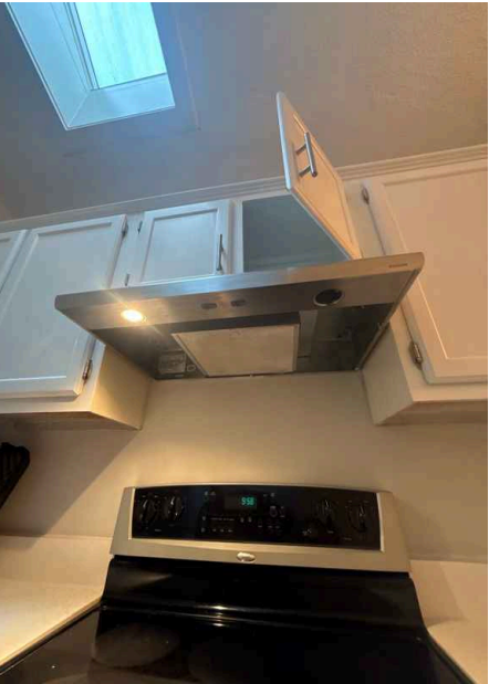
Ventilation Equipment/Hood: Ventilation Type Hood recirculates
