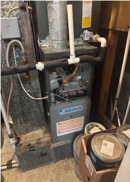
Equipment: Photo Heating Equipment
