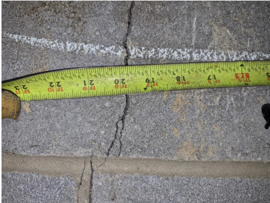
Picture 3 – Approximately 1/16" wide (foundation crack same as shown in picture 2)
