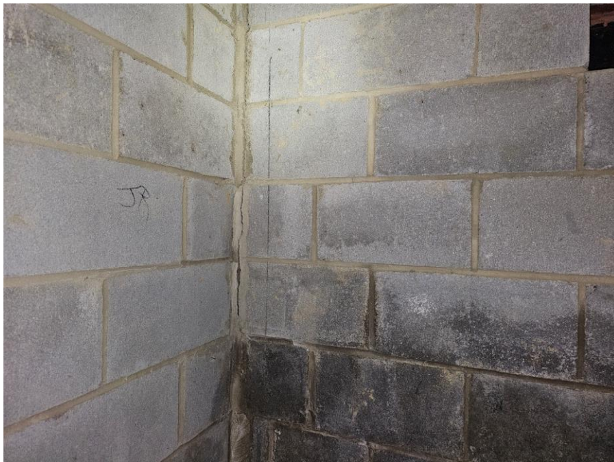
Picture 4 – Foundation crack
