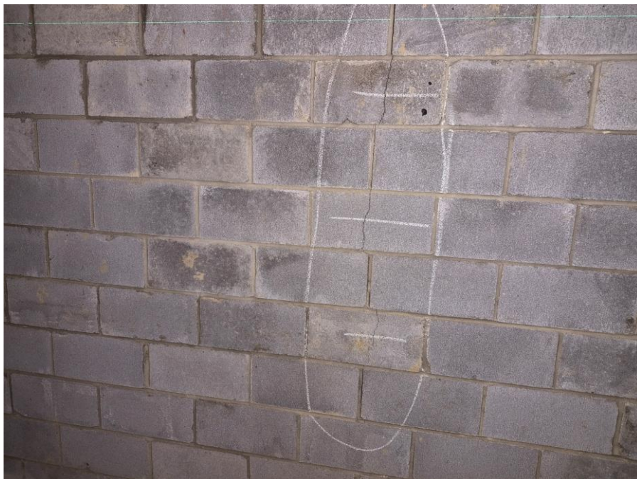
Picture 2 – Foundation crack reported to have previously been circled
