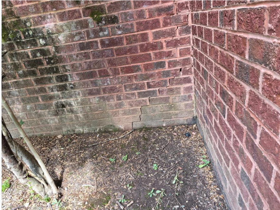
Picture 5 – Retaining wall crack
