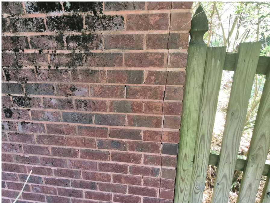
Picture 6 – Retaining wall crack
