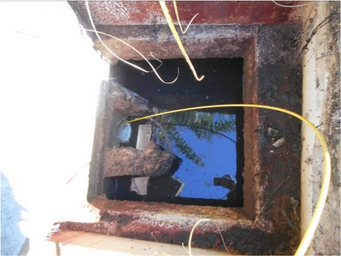
Outlet Compartment of Septic Tank
