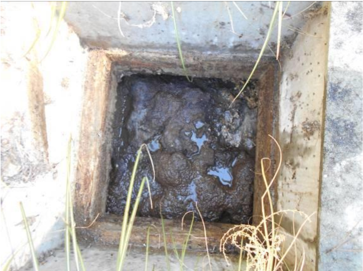
Inlet Compartment of Septic Tank
