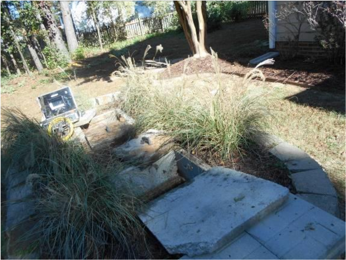
Septic Tank Location
