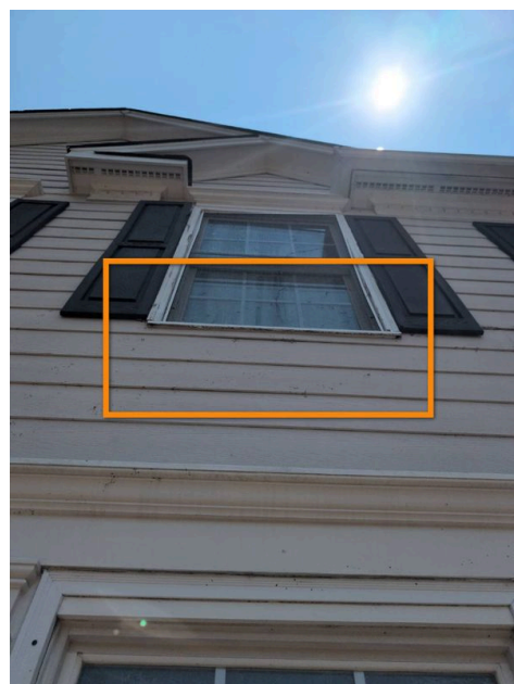
Wood deterioration on windows
