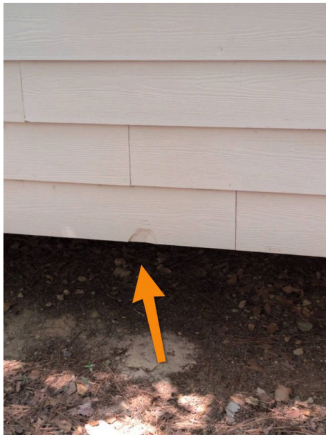
Back of home, damaged siding
