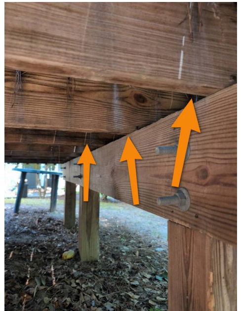
Having joist hangers or brackets for reinforcement can prevent further rotation of the deck
