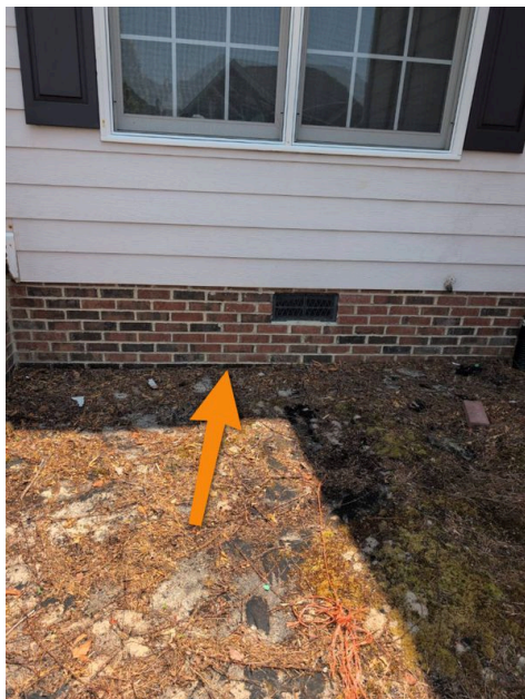
Front of house - again, check gutters for functionality
