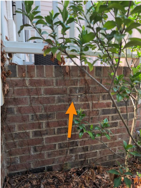
Missing mortar - check all areas where brick exists
