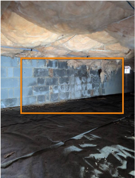
Front of the house - moisture Intrusion
