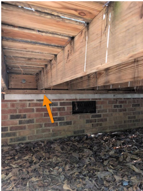
Some joists are twisted in place
