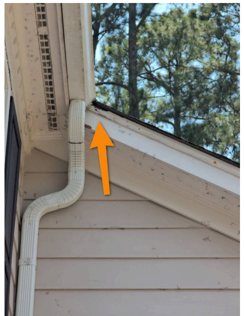
Front of house - deterioration
