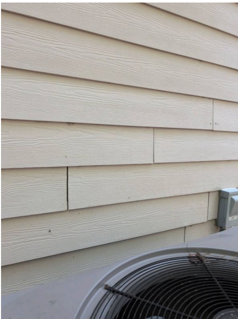
Left side of home - loose siding
