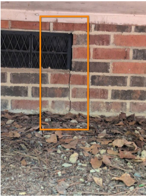
Back of home - brick facade is cracked at crawlspace vents
