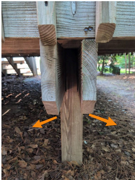
These beams are slightly shifted
