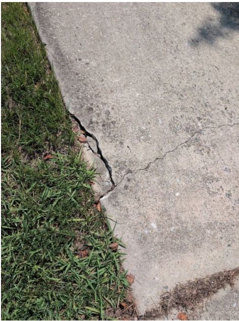
Slab cracks on driveway
