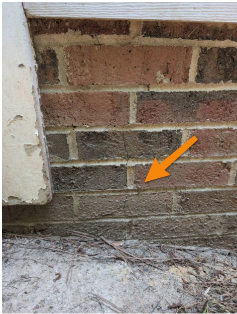
Small cracking on right side of crawlspace entrance
