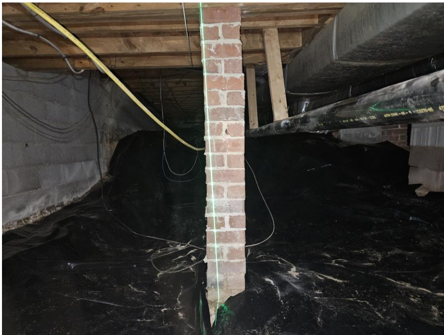
Picture 10 – Leaning pier
