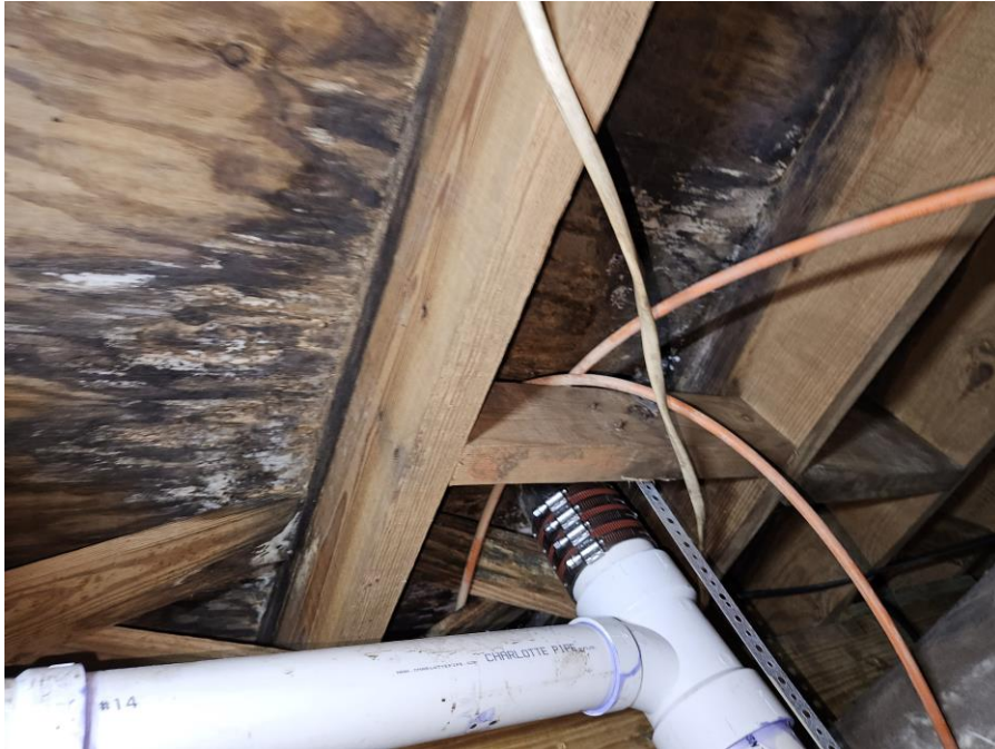
Picture 5 – Damaged subfloor
