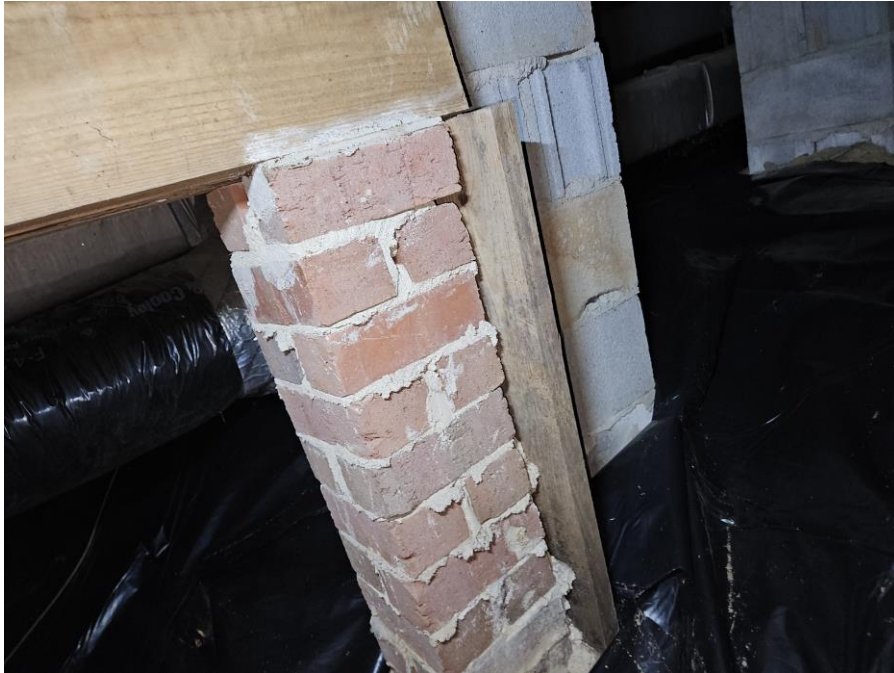
Picture 9 – Leaning pier with undermined footing
