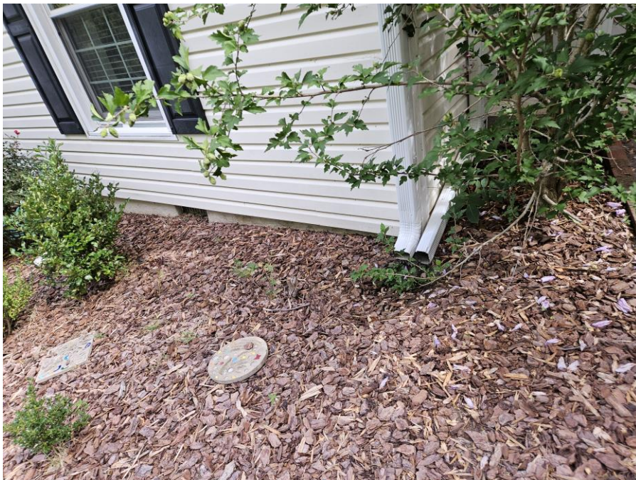
Picture 4 – Roof gutter downspouts set for discharge at foundation soils
