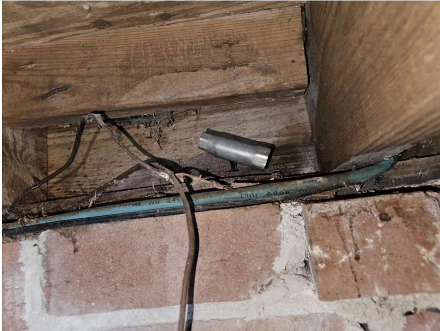
Picture 11 – Damaged sill plate and rim band
