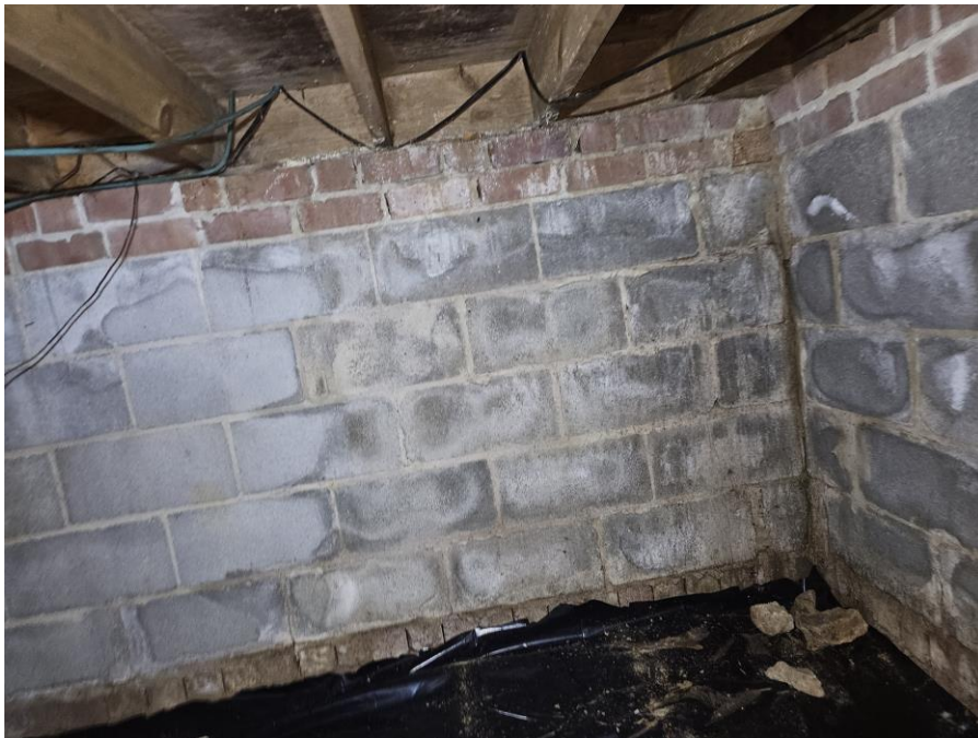
Picture 2 – Efflorescence and signs of water intrusion
