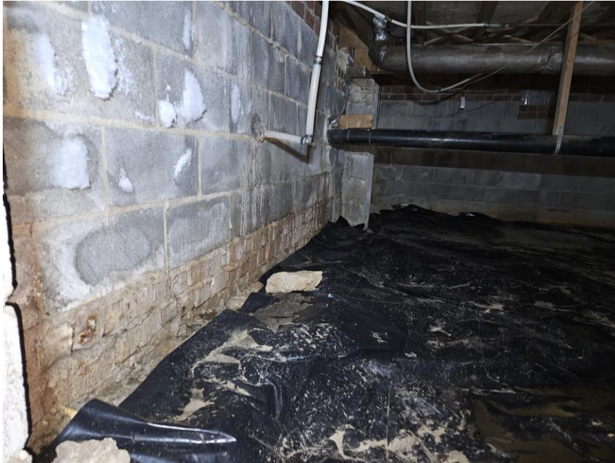
Picture 3 – Standing water in the crawlspace
