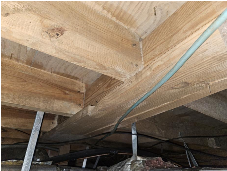
Picture 12 – Example of slipped ledger
