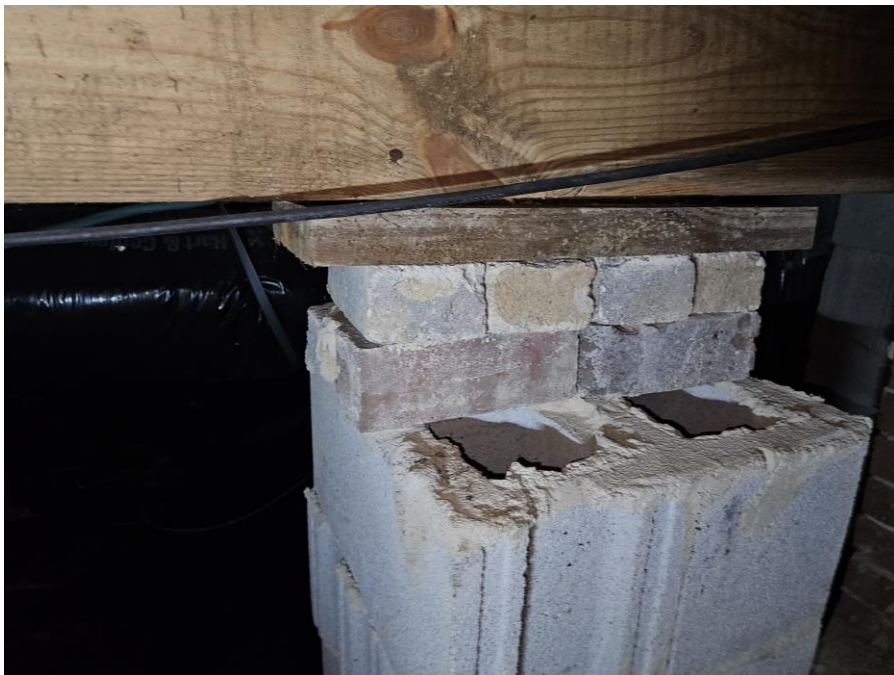
Picture 6 – Example of hollow pier missing solid caps
