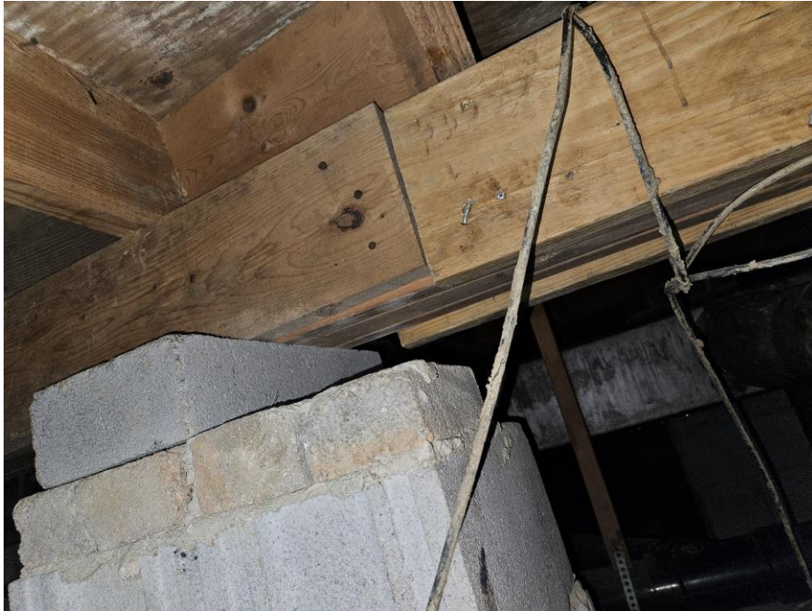
Picture 7 – Non-continuous plies of dropped girder
