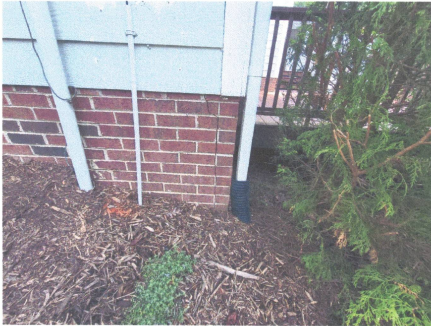
Picture 3 – Foundation crack
