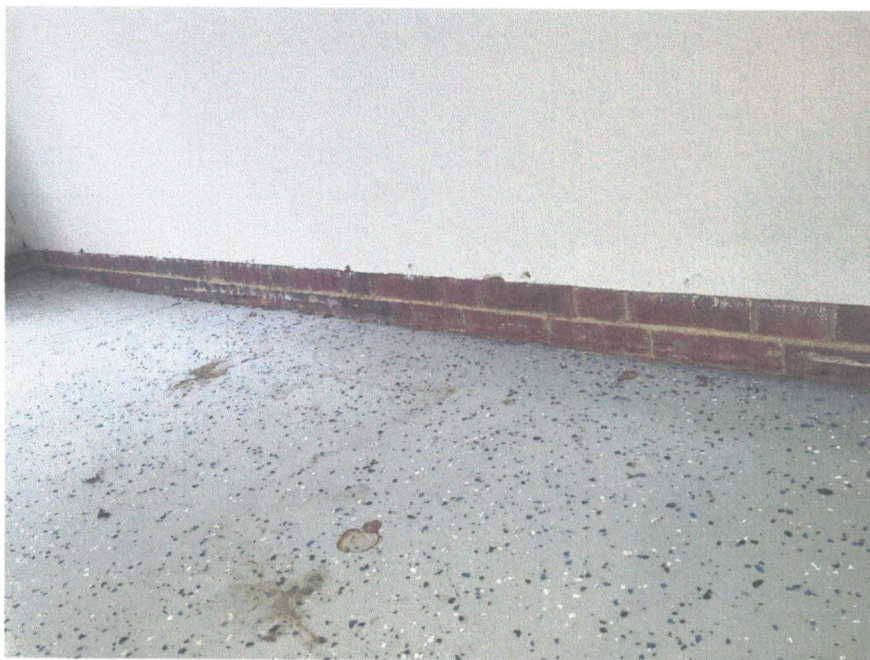
Picture 4 – Slab settled into fill material
