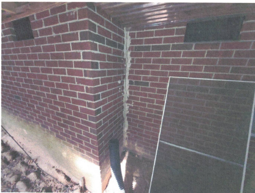
Picture 6 – Foundation crack
