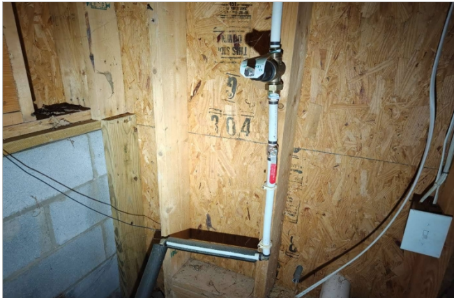
The main water shutoff is located in the crawlspace.
