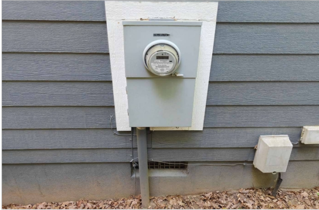
The electrical service entry is located on the left elevation.
