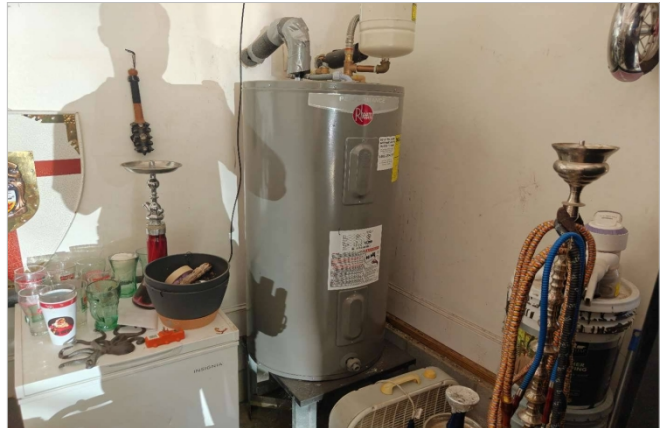
The water heater is located in the garage.
