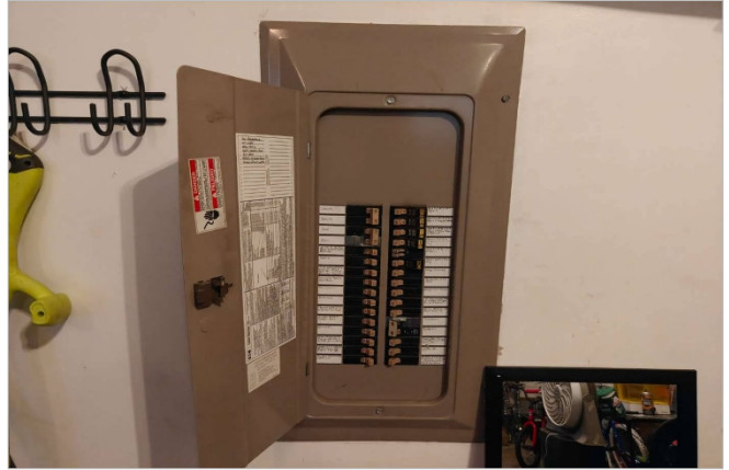
The sub-electrical panel is located in the garage.
