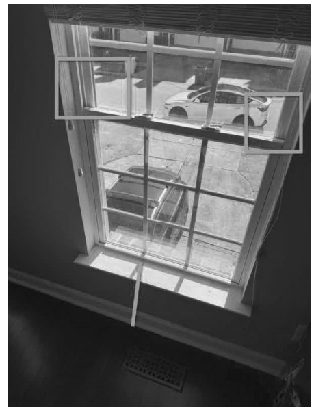
Multiple windows throughout home missing safety locks
