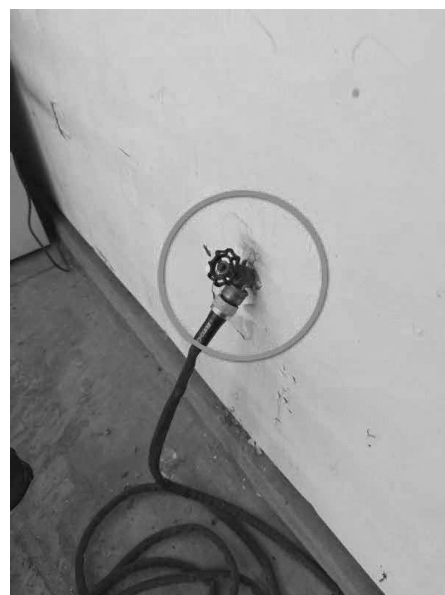
Garage area hose bib
