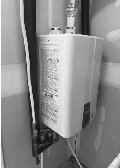
Located in garage utility room
