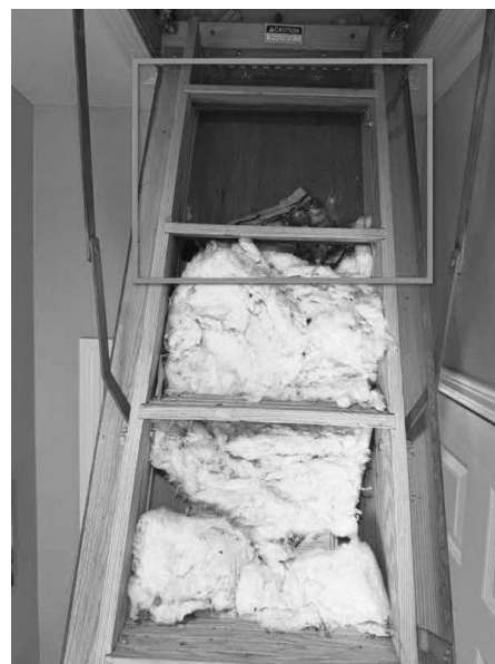
Missing insulation at drop down staircase
