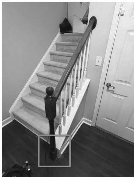
1st floor staircase. Loose at base attachment
