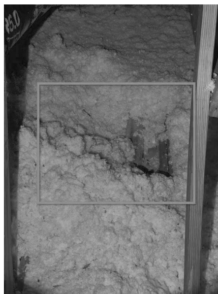
Low spot in middle attic area
