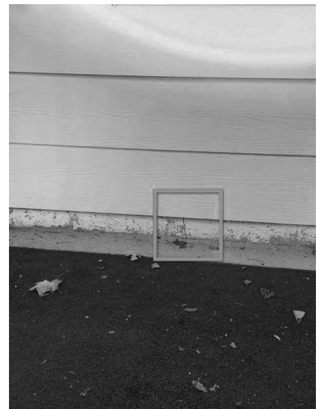
Rear patio area, vertical crack at slab
