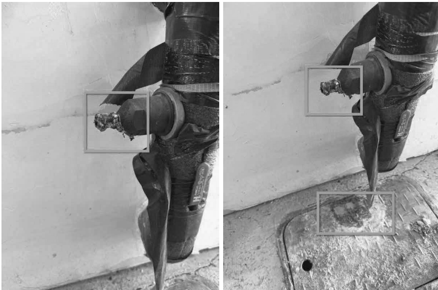
Prv leaking in garage utility close
