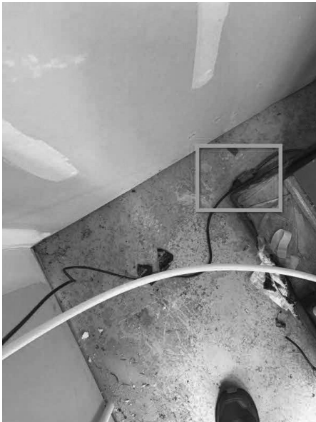
water heater is powered via extension cord
