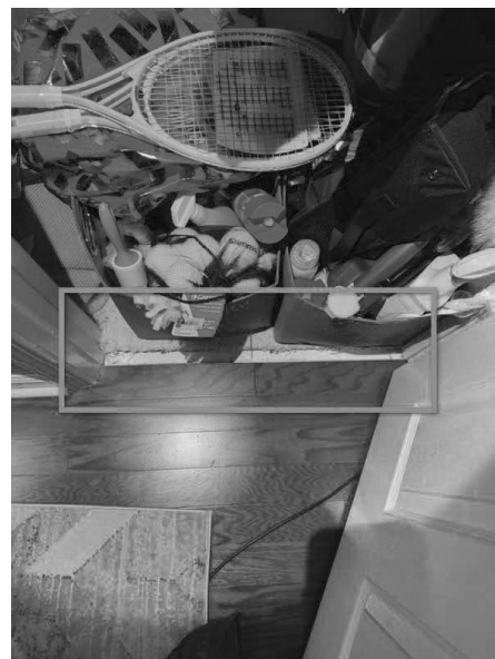
2nd floor hall closet. Transition strip missing
