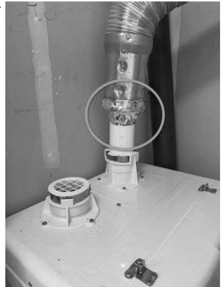
Questionable install of vent/exhaust. Typically a pvc to metal adapter is needed.
