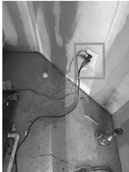
Typically recommended to have a dedicated circuit for water heater plug
