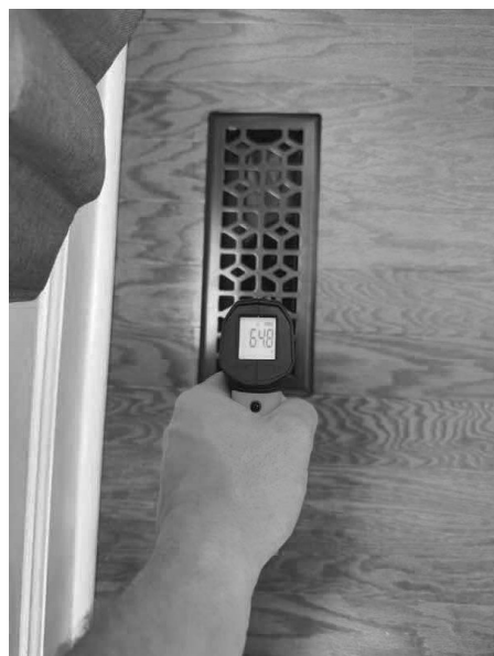
2nd floor. Higher than normal supply temp
