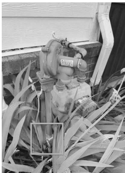
Located at rear exterior meter
