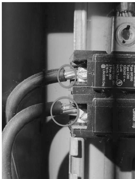
Rear exterior panel box
