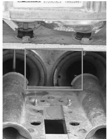
1st/2nd floor furnace
