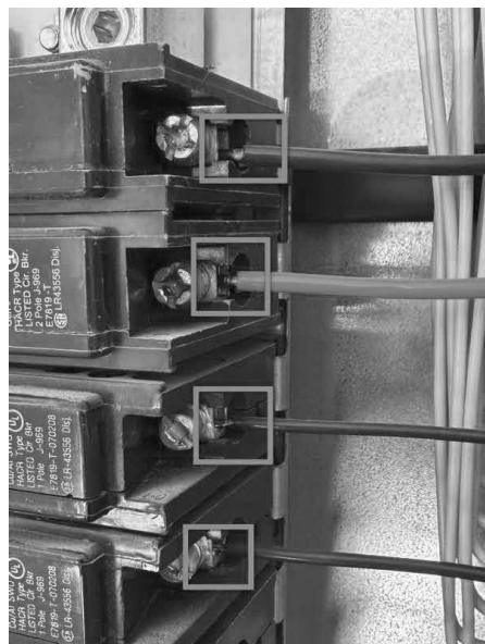
Garage panel box
