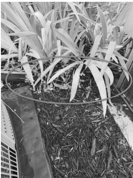
Older unit line set
