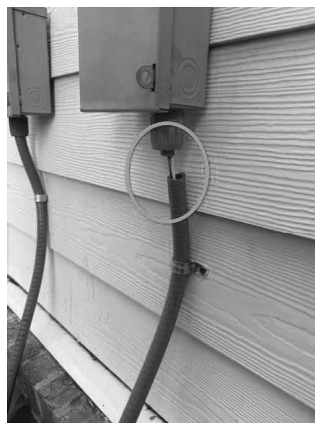
Rear exterior, hvac disconnect wiring/flex conduit
