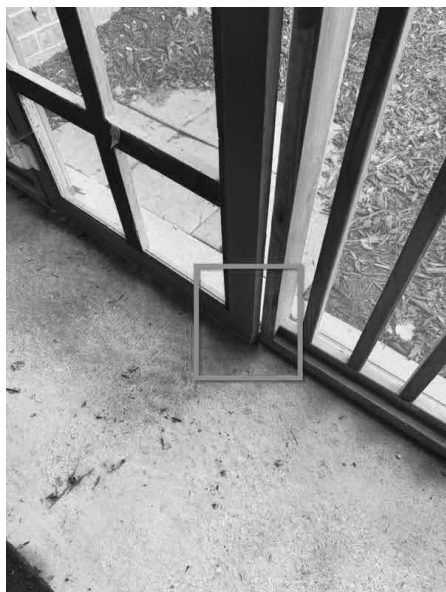
Rear deck screen door. Hitting frame
