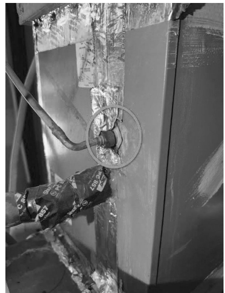
Garage utility room furnace. Leaking conditioned air
