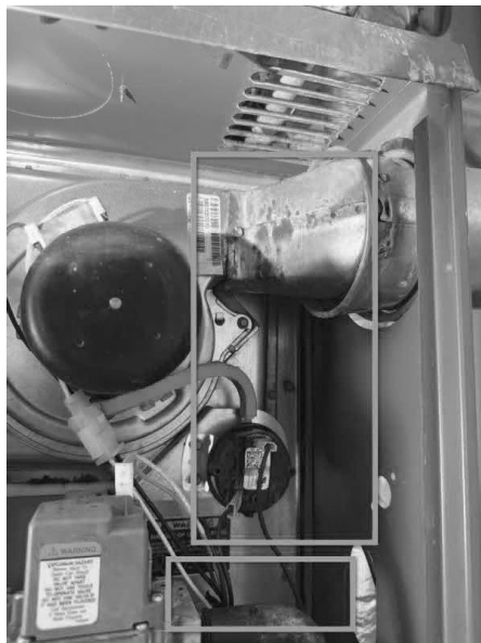
1st floor furnace cabinet
