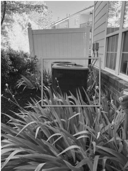
Older unit not level
