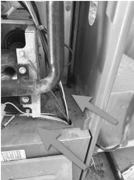
Garage utility room furnace
