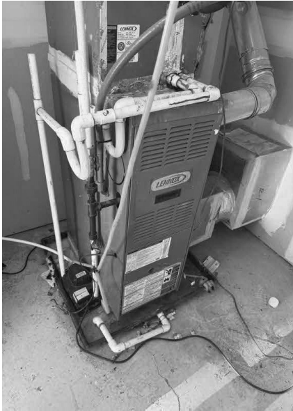
Located in garage utility room
