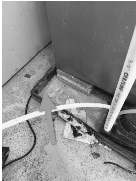
Garage utility room furnace
