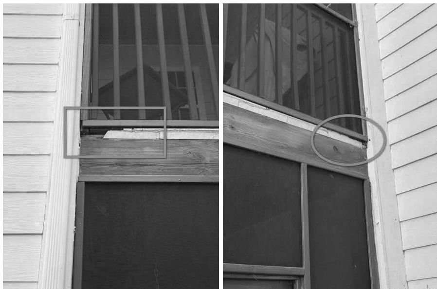
2nd floor deck tile, damaged/missing
