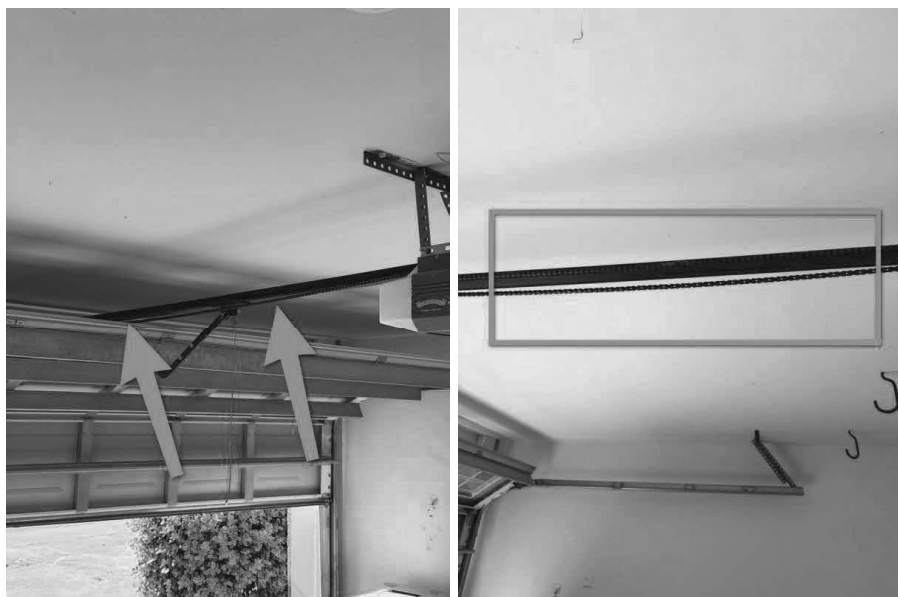
Garage door drive chain had excessive slack and movement
