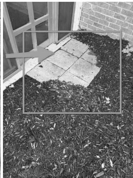
Rear patio pavers. Settlement noted
