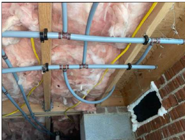
PB piping with copper directional fittings and copper compression band fittings
