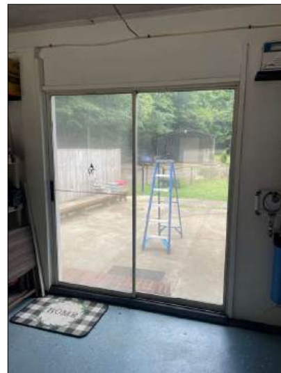
The garage to exterior sliding glass door panes appear to have a defective hermetic seal.
