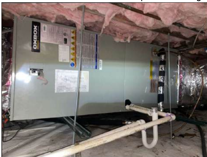
The air handler and evaporator coil unit
