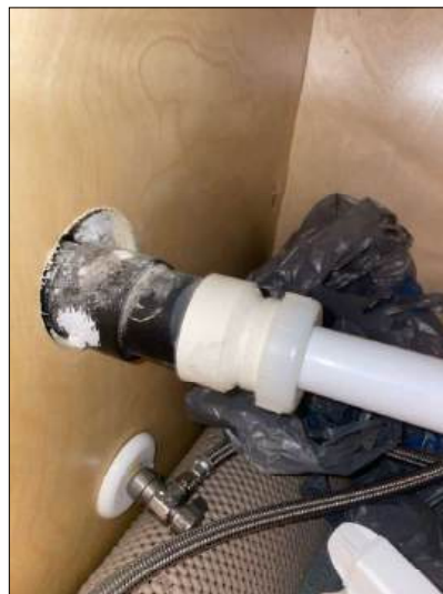
PVC to ABS pipes should be mated using a coupler fitting, as opposed to being glued together.
