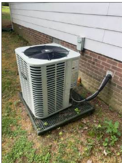
The outside coil/compressor unit
