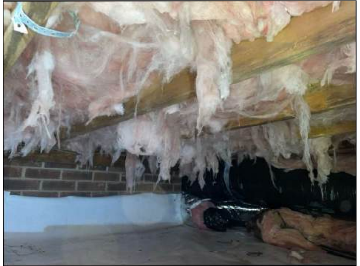
Stripped insulation in the right crawlspace
