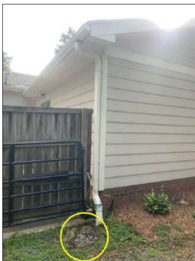
The ground depression at the rear left corner.
