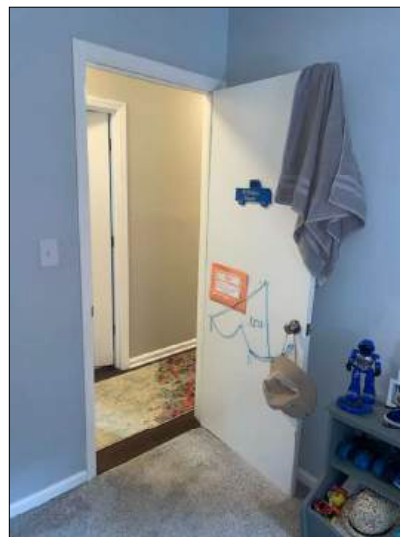
The entry door for the rear middle bedroom drags on the carpet, and contacts its frame.
