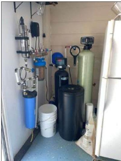
There is a water softener system present. This system is not evaluated as a part of this home inspection.
