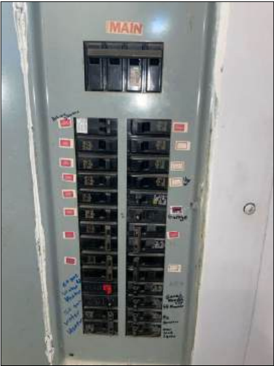
The main panelboard
