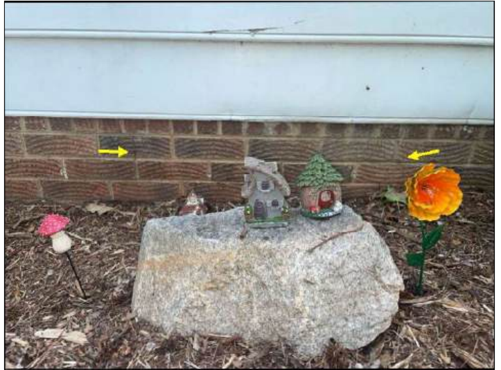
Two cracks at the left side middle area
