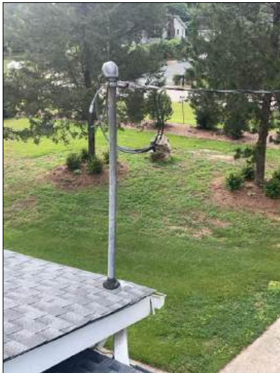
The electrical service entrance is overhead
