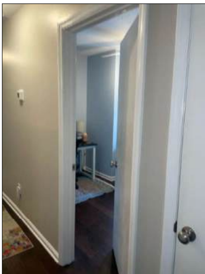
The front left bedroom entry door does not latch closed.
