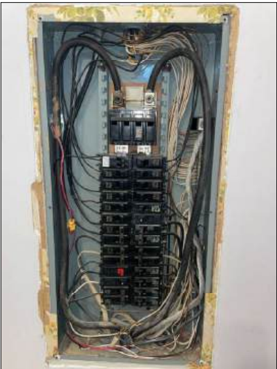
The main panelboard
