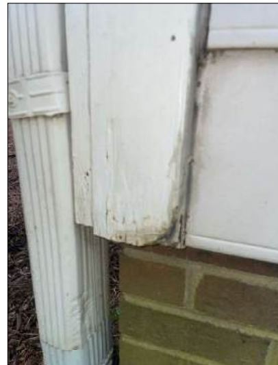
Damaged trim at the right front corner
