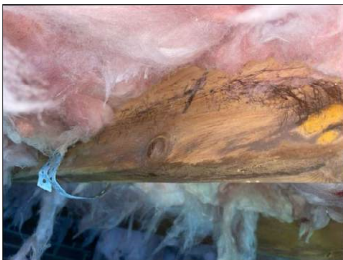
The veiny pattern is indicative of previously active wood destroying fungus.
