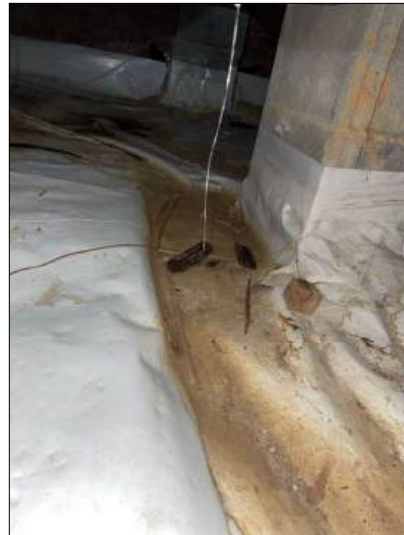
Mud stained vapor barrier liner is indicative of previously puddled water.
