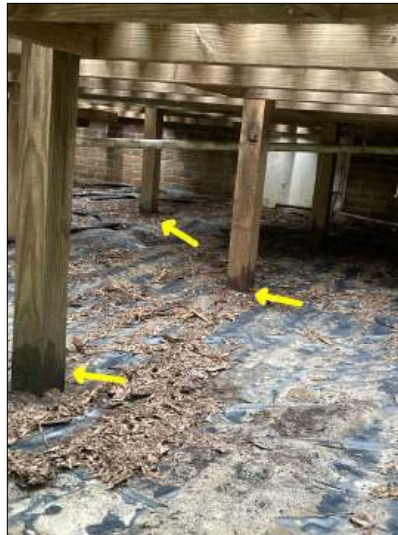
There appears to be some level of wood decay at the base of stiff knee supports.
