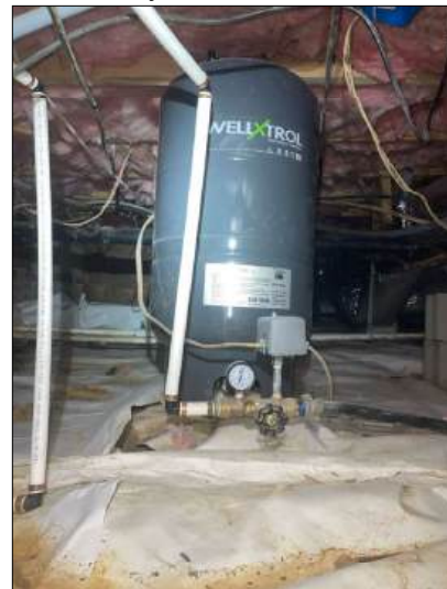
The water pressure tank
