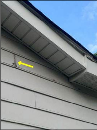
Damaged siding at the right side middle area
