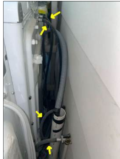
I recommend proactive replacement of the rubber fill lines, with stainless steel braided flex lines.
