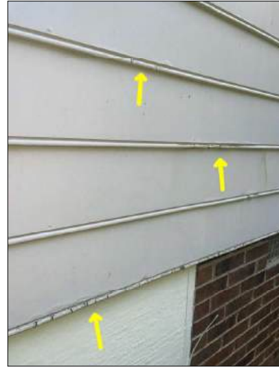
Damaged siding at the rear side right
