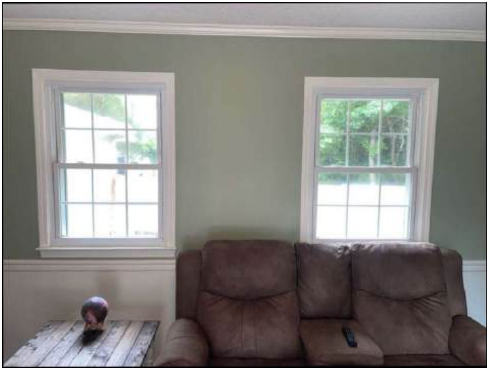
Cloudiness, mineral deposits, and/or condensation between the glass panes is indicative of a failed hermetic seal.
