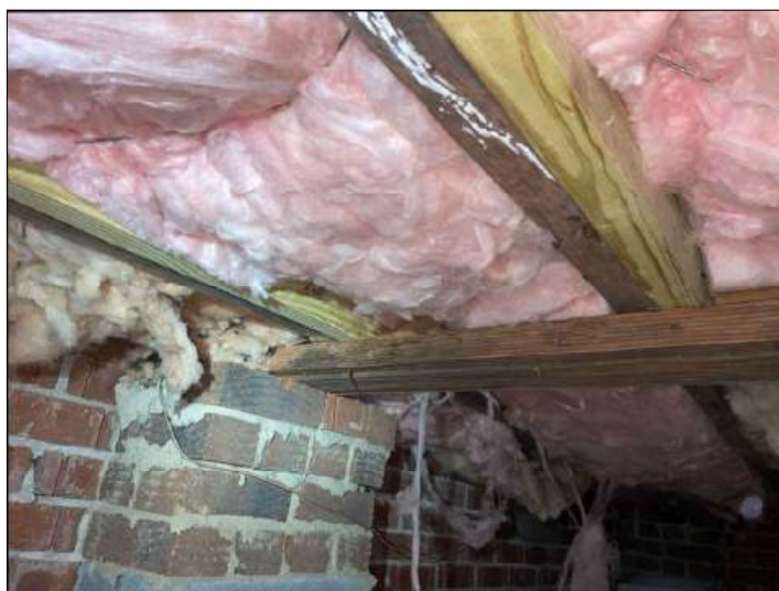
Discoloration of the girder and on the bottom surface of the floor joist.
