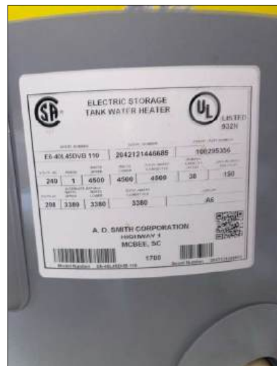
The water heater data plate
