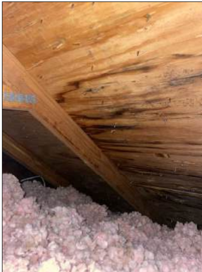
Roof structure discoloration located adjacent to the attic access ceiling scuttle, above the primary bedroom closet.
