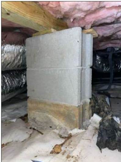
The addition of CMU piers and drop girders indicate foundation repair.
