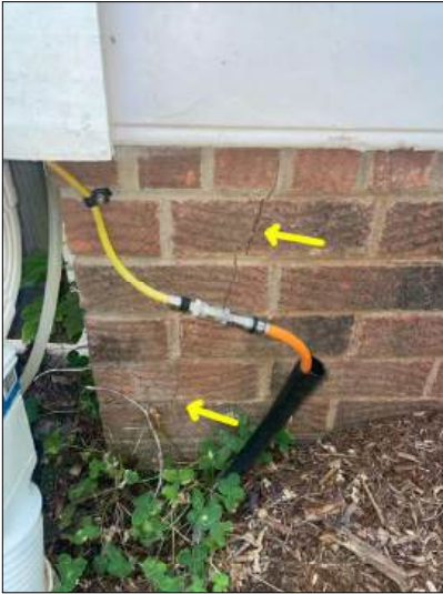
Foundation wall crack at the left side rear corner
