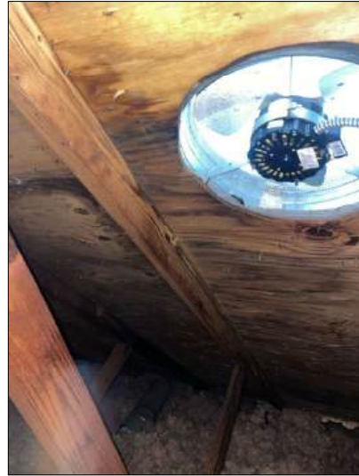
The discoloration is indicative of water exposure to the roof structure.
