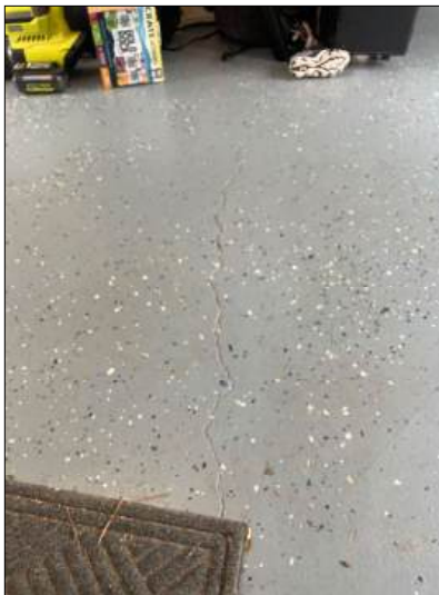
Garage slab crack
