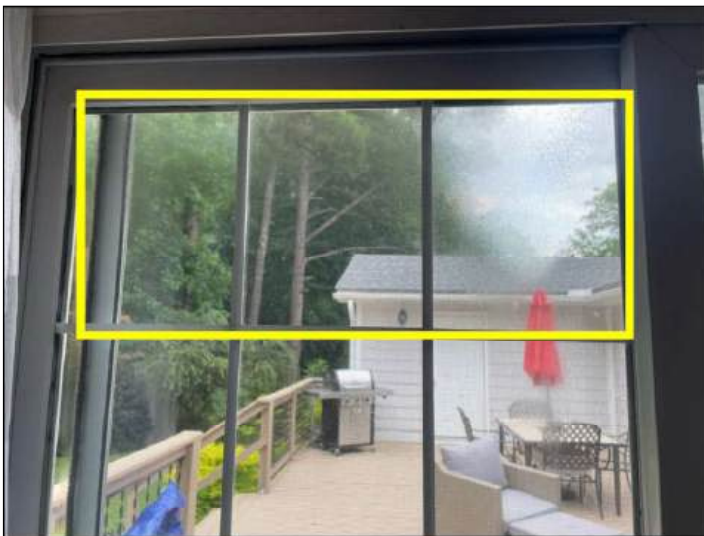
Condensation between the glass panes is indicative of a failed hermetic seal.
