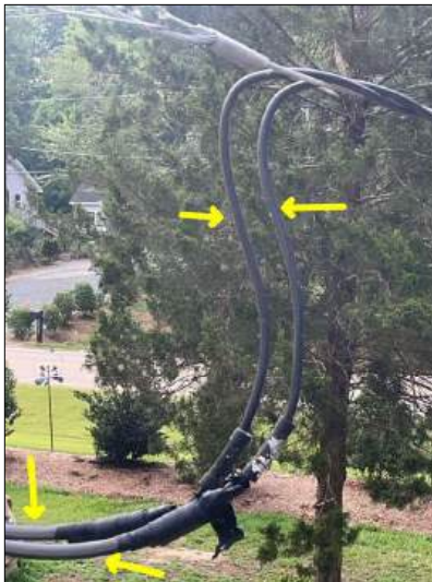
There is an obvious gauge size difference between the conductors that are fed from the street, and the conductors that are fed to the panelboard.
