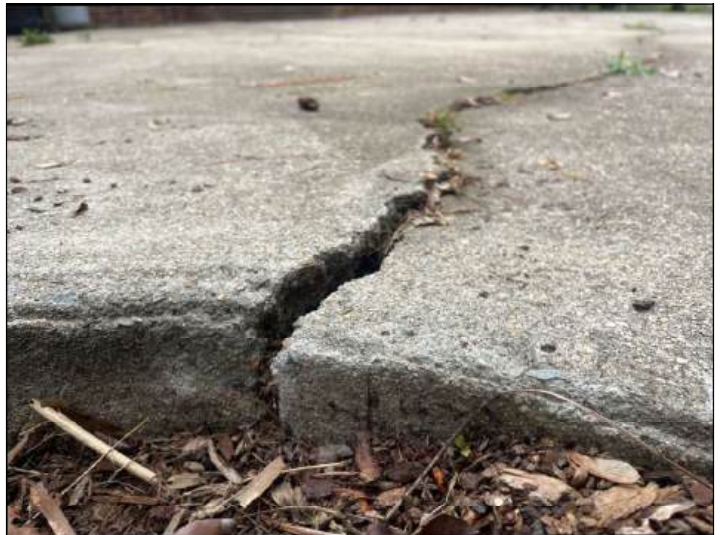
The most significant patio crack has translation.
