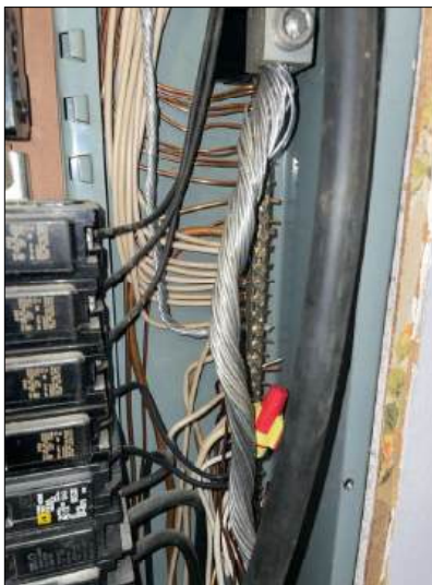
Ground connections in the panelboard
