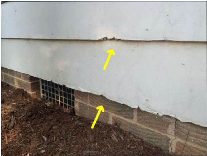
Damaged siding at the front side right
