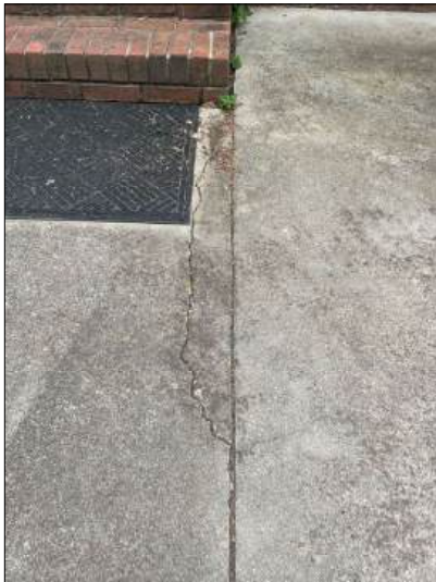
Patio cracks should be sealed
