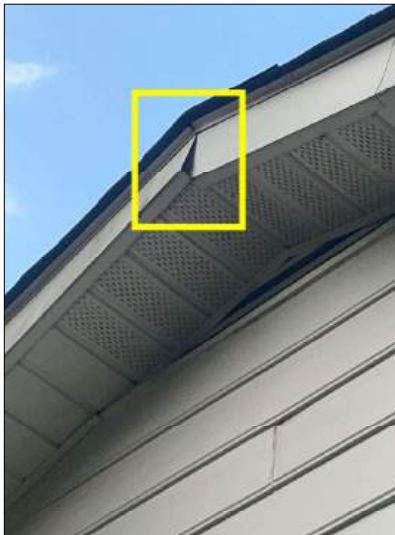
Loose metal fascia on the right side
