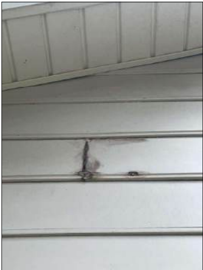
Damaged siding at the right side front
