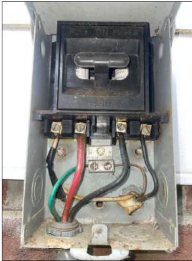
Energized conductors and contacts are accessible
