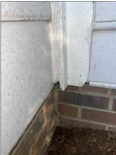
Damaged trim at the front side right
