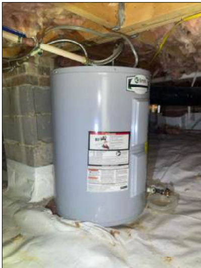
The water heater
