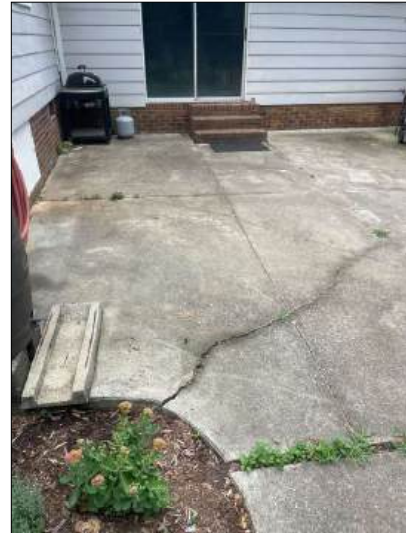
Patio cracks should be sealed
