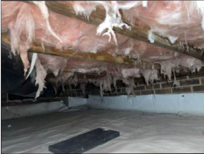
Stripped insulation in the right crawlspace
