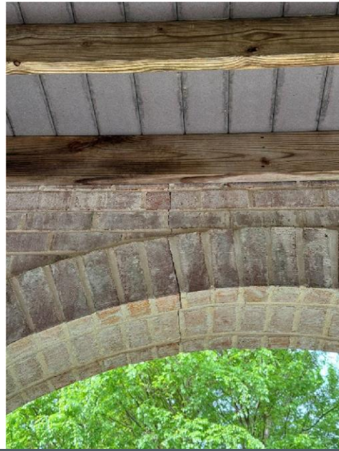
Photo 10: Cracking above arches at rear patio
