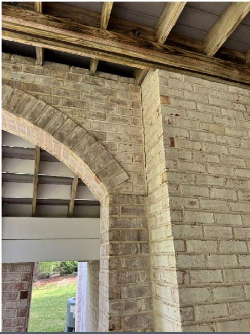
Photo 9: Cracking at rear patio along home and patio wall
