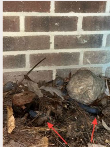
Condensate drains for ductless heat pump
