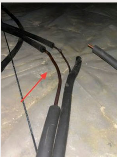
Ductless heat pump
