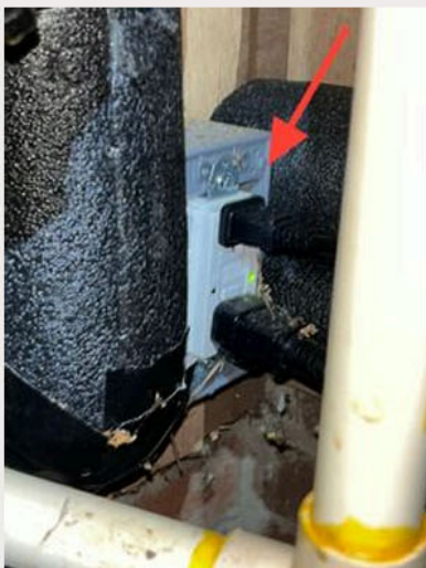
Garage at tankless water heater
