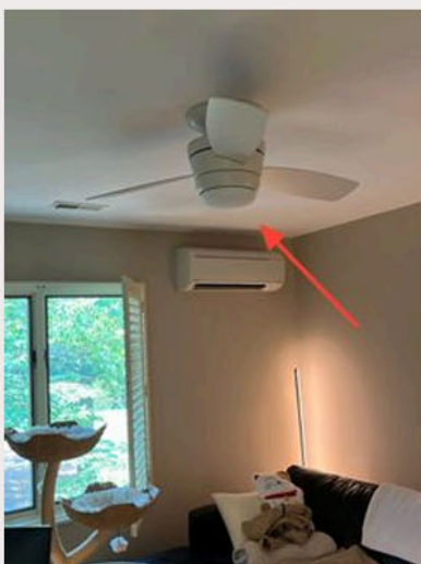
Both upstairs bedroom fan lights
