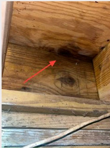
Under sliding glass door in master bedroom
