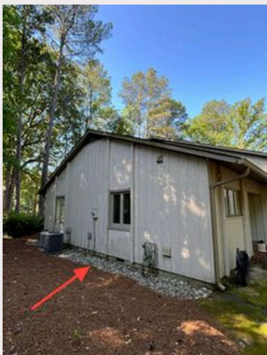
Left side of unit (drainage system installed here)
