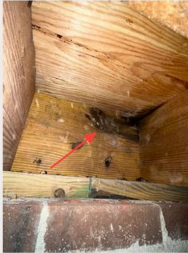
Under sliding glass door in the living room
