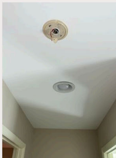
Missing smoke detector at second floor hallway. Combination smoke/CO detectors should be installed at each floor in the hallways outside bedrooms.
