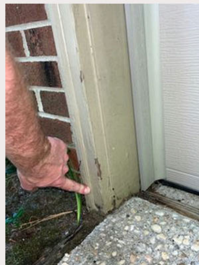
Left corner of Garage - siding/trim should not contact the ground
