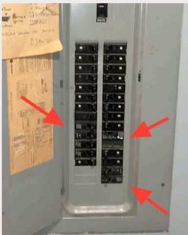
Siemens breakers should not be installed in a GE panel
