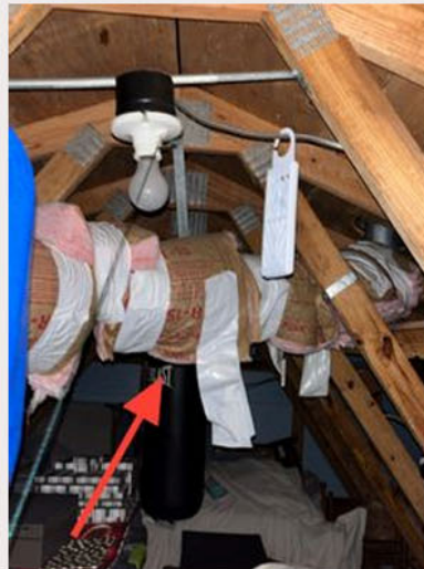
The furnace flue should not be insulated
