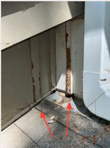
Squirrel damage at rear side of house
