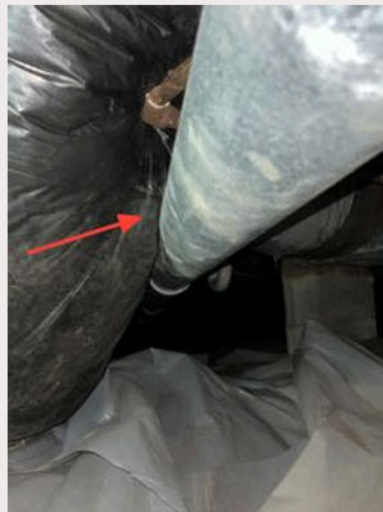
Furnace flue contacts ductwork in the crawl space
