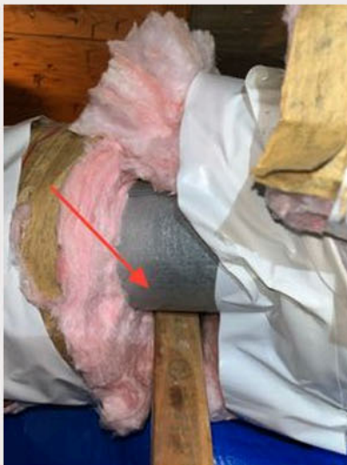
Furnace flue contacts wood truss in the side attic
