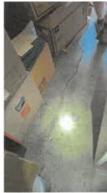
Garage slab crack
