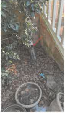
Gutter deposits next to basement
