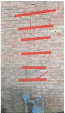
Brick facade cracking
