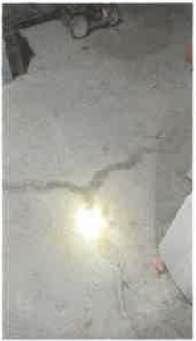
Basement slab moisture
