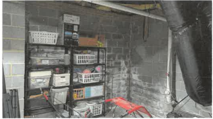
Efflorescence in basement
