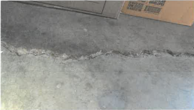
Garage slab settlement
