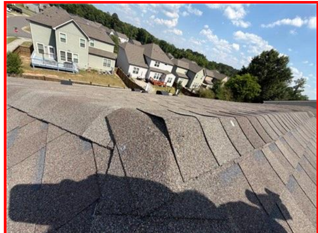
Lifted Ridge Cap Shingle
