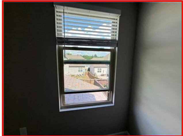
Windows Difficult to Lock / Secure
