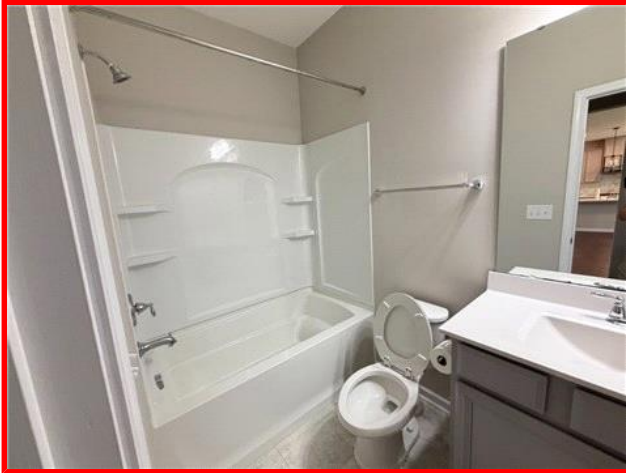
Toilet in Downstairs Bathroom Loose at Base
