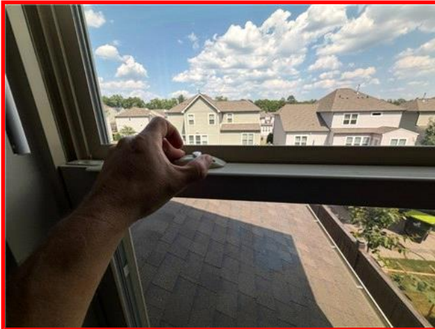
Windows Difficult to Lock / Secure
