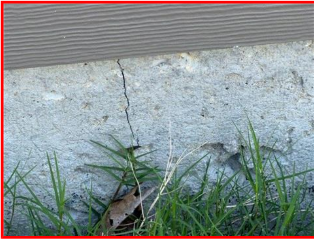
Crack in Left Foundation Wall
