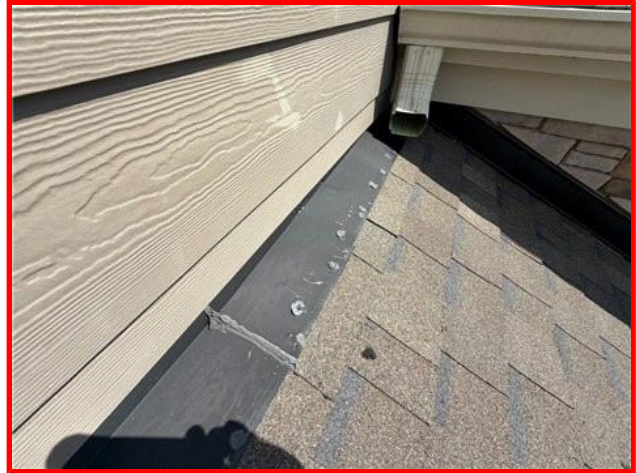
Exposed Nail Heads at Headwall Flashing
