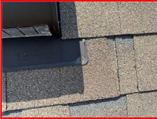
Exposed Nail Head at Dryer Vent
