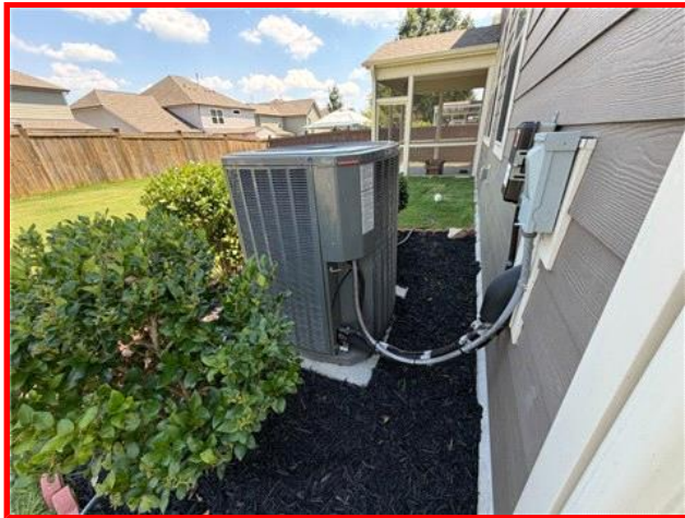
A/C Unit -Temp Diff too Low
