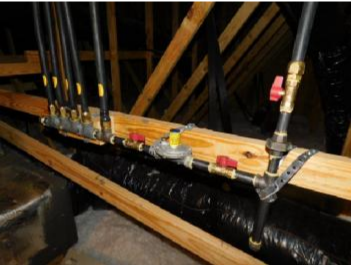
HS-9 No visible bond/ground wire to CSST gas tubing
