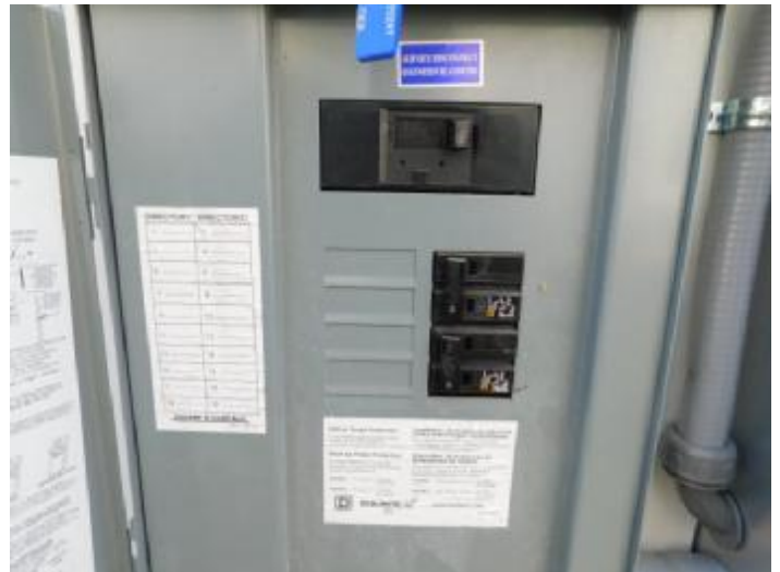
Main electric disconnect panel
