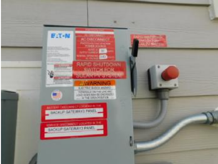
Solar panel system
