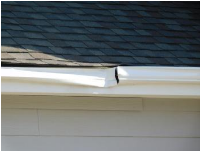
R-11 Damaged gutters at front above garage
