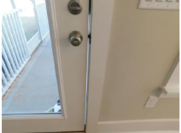
ES-3 Damaged weather stripping at rear exterior door
