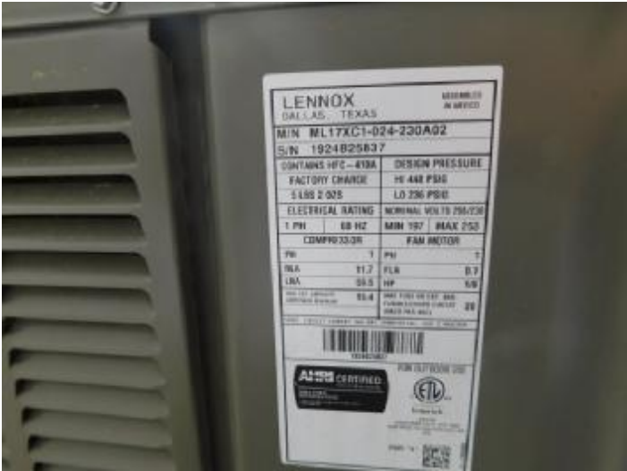
Air conditioner #2 label
