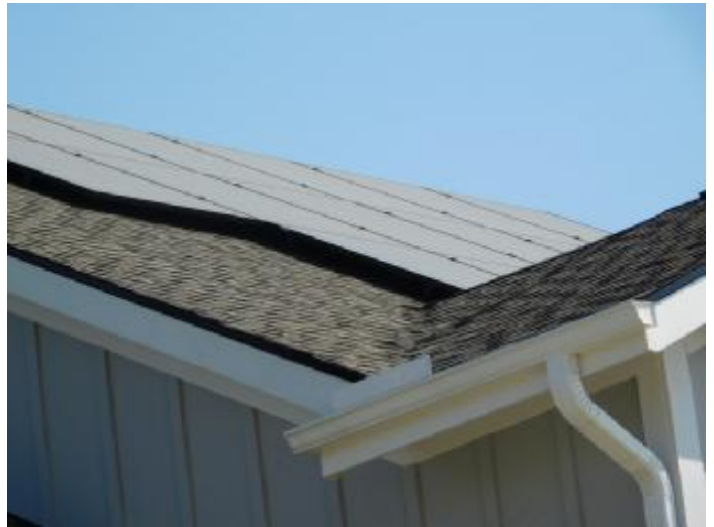
Solar panel system
