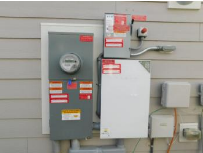
Electric meter and main electric disconnect panel
