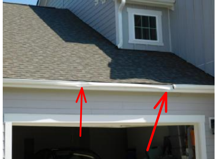
R-11 Damaged gutters at front above garage
