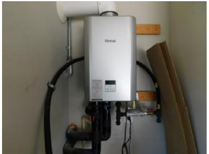
Tankless water heater
