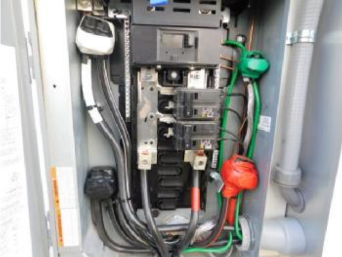
Main electric disconnect panel
