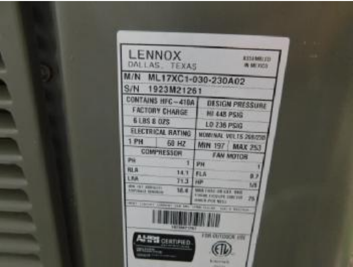
Air conditioner #1 label
