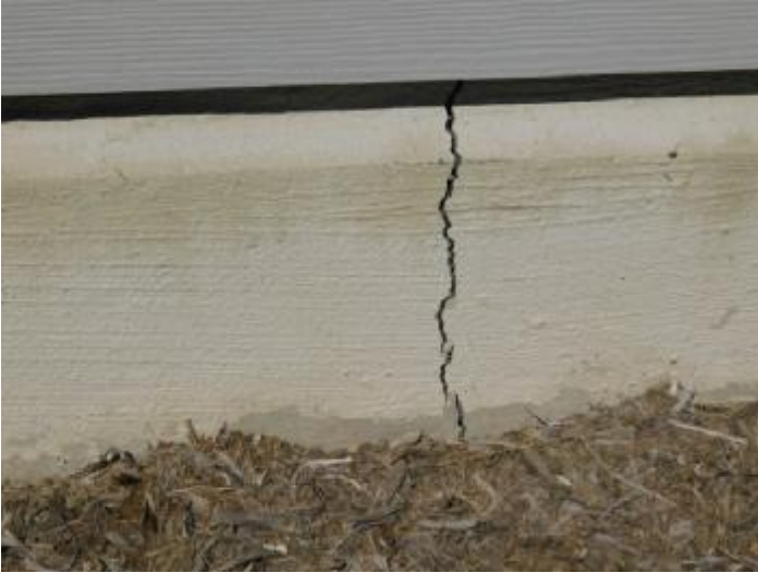
S-1 Cracks at concrete slab foundation at right side
