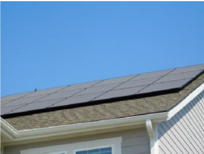
Solar panel system
