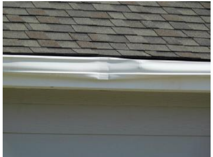
R-11 Damaged gutters at front above garage
