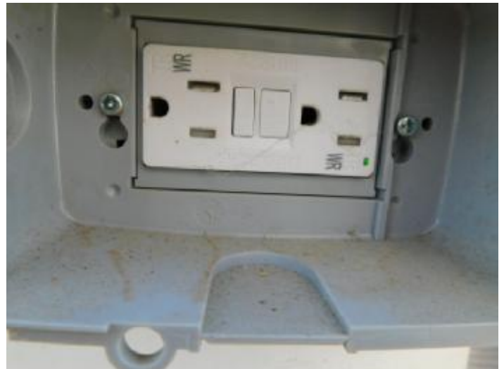
E-7 GFCI outlet at exterior left side did not reset when tested
