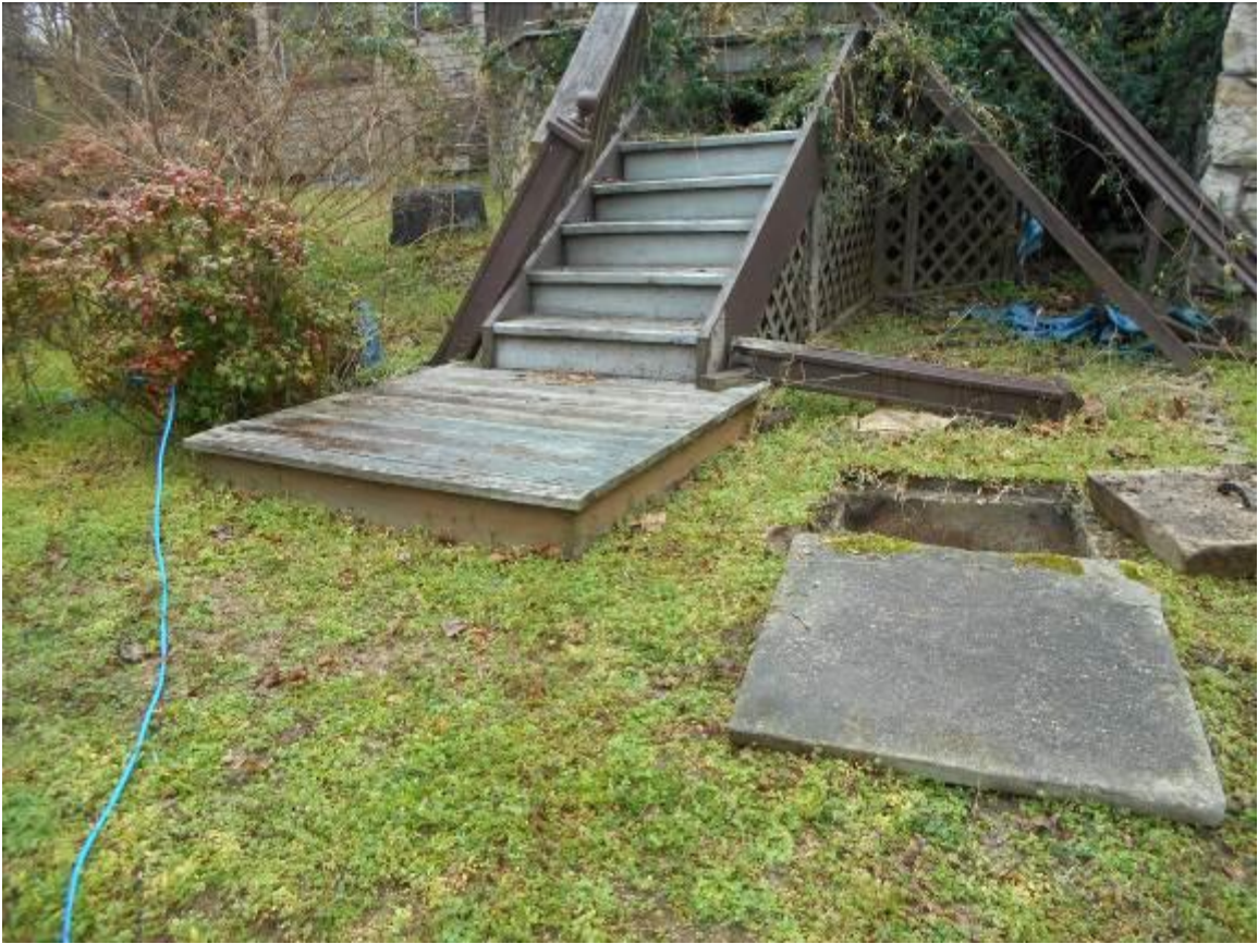
Septic Tank Location
