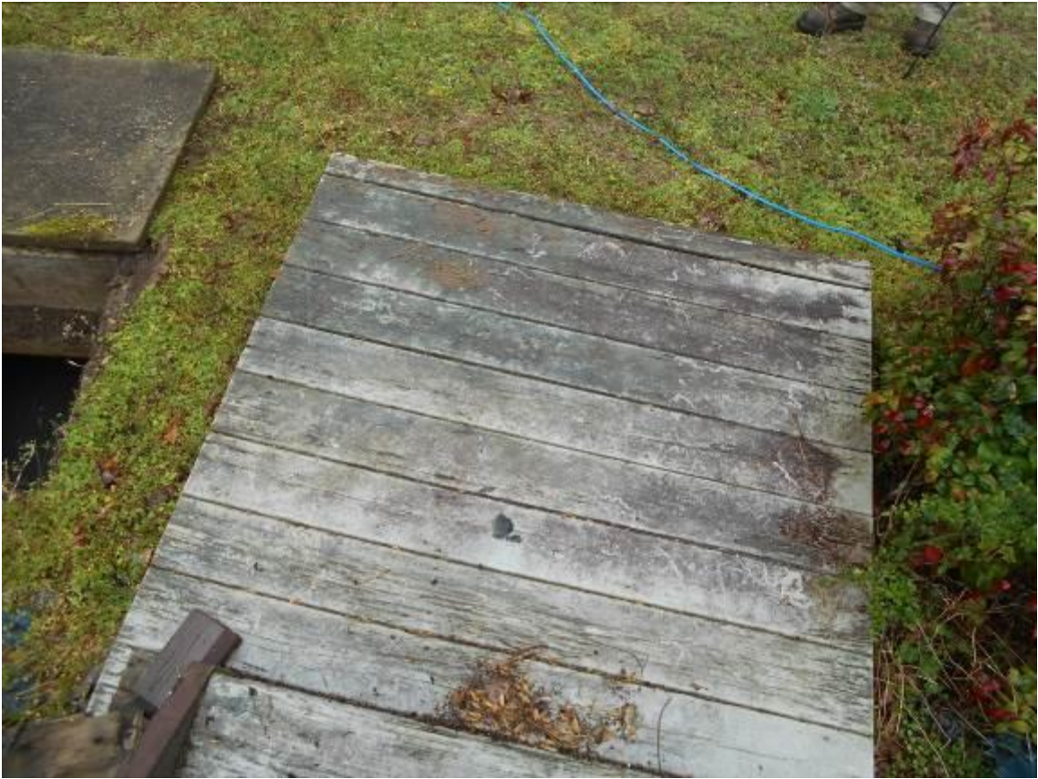
Outlet Compartment Location
