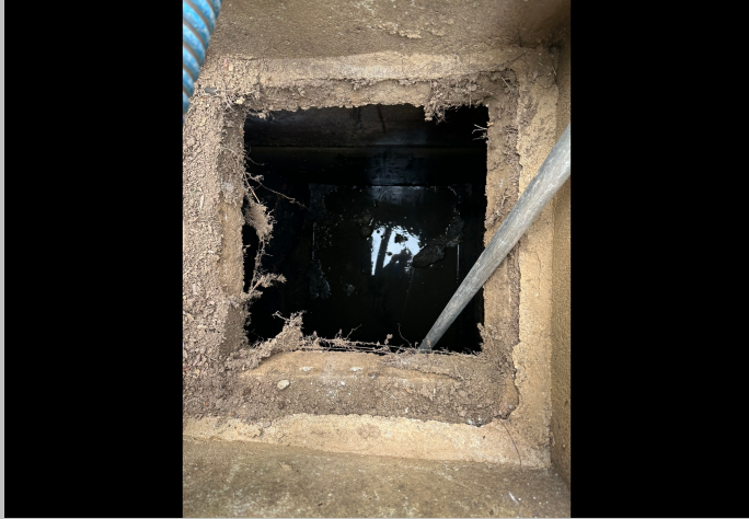
Inlet side of tank
