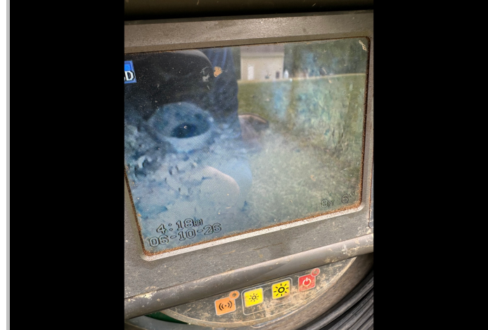
Distribution box shown deteriorated
