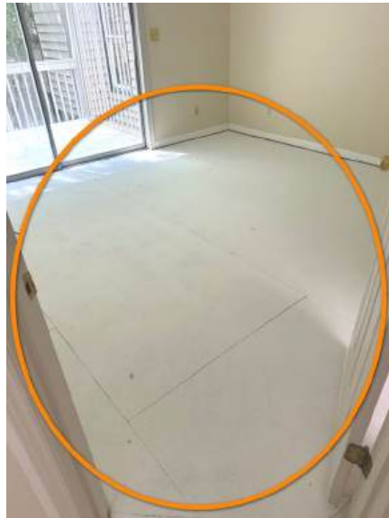
Flooring materials have been removed in numerous locations throughout interior of home (Main level, primary bedroom)
