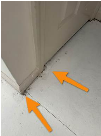
There was an area of deterioration in areas of the subflooring (main level, middle hallway)
