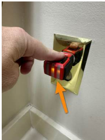
No GFCi protection present in main level hallway bathroom electrical receptacle
