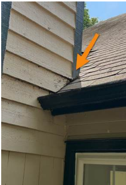
Deterioration observed in areas of siding/trim on left side exterior of home (chimney chase)
