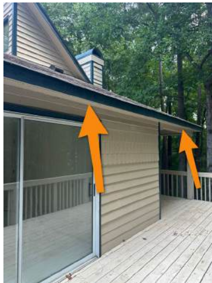
No gutters installed on rear of home
