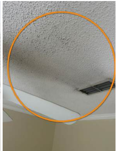
Dirt/debris and suspected organic growth was noted in ductwork and at distribution registers and returns throughout home
