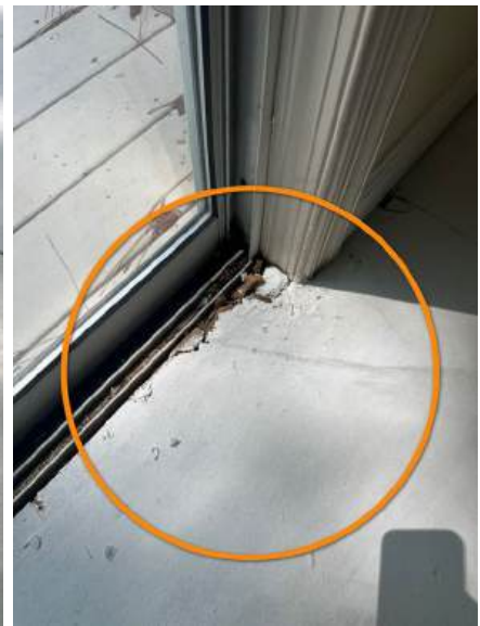
There was evidence of moisture intrusion near or at an exterior door (main level rear exterior sliding glass door, primary bedroom)
