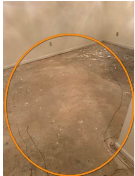
Flooring materials have been removed in numerous locations throughout interior of home (lower level, front bonus room)
