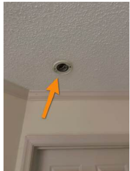
Smoke detector has been removed on ceiling in lower level family room
