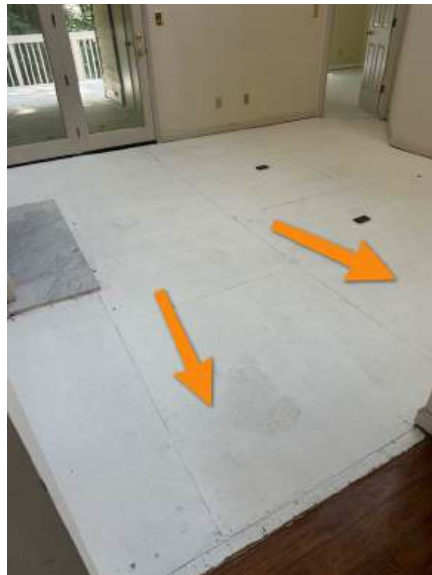
Areas of flooring are creaky on main level of home (living room)
