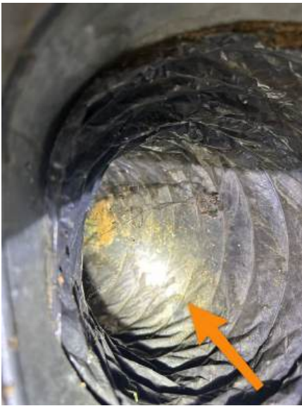
Dirt/debris and suspected organic growth was noted in ductwork at distribution registers and returns throughout home
