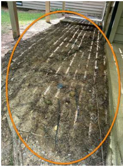
Evidence of soil erosion (rear exterior)
