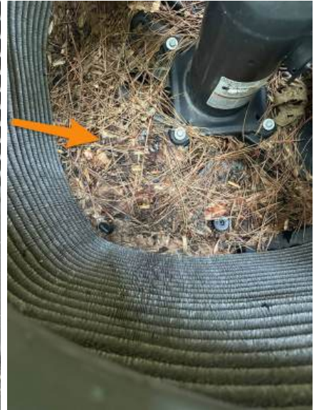
Organic debris present in main housing of exterior HVAC condenser unit/heat pump
