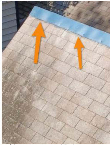
Uplift/gaps in areas of flashing on middle roofing of home
