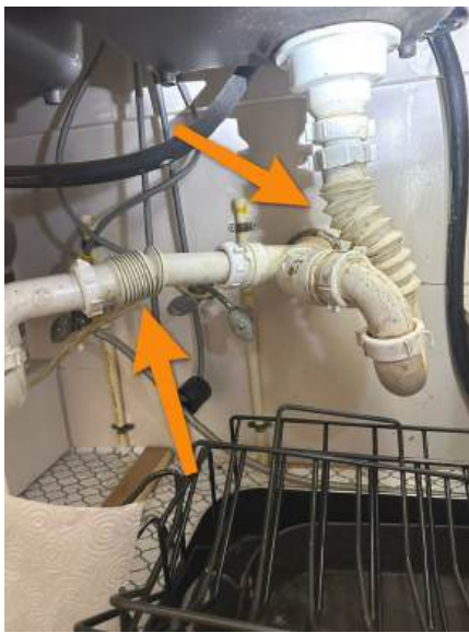
There was flexible drainage piping installed underneath kitchen sink
