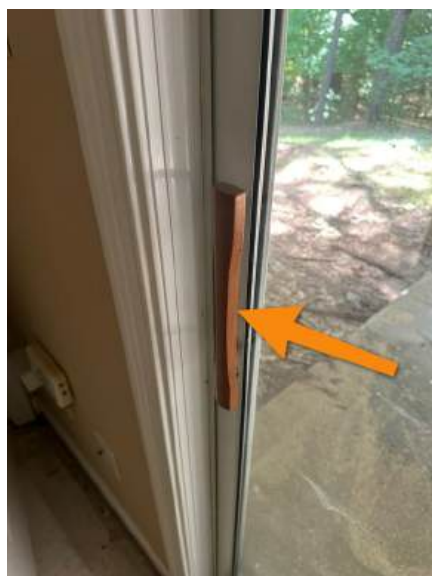
Handle is loose on rear exterior sliding glass door (lower level left rear family room)
