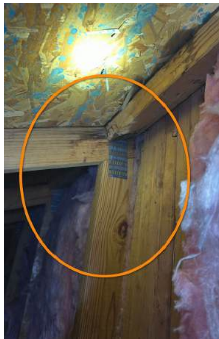
Moisture staining observed on areas of roof and side wall framing in middle right area of attic
