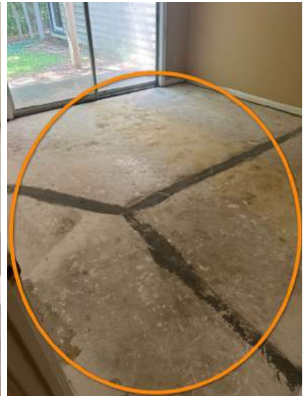
Flooring materials have been removed in numerous locations throughout interior of home (lower level, right rear bedroom)
