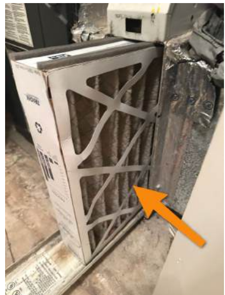
The HVAC in-line box air filter is dirty
