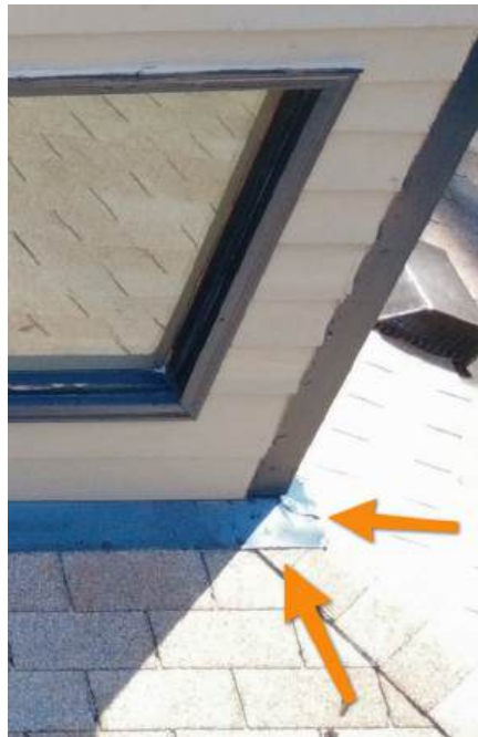
Uplift/gaps in areas of flashing on middle roofing of home
