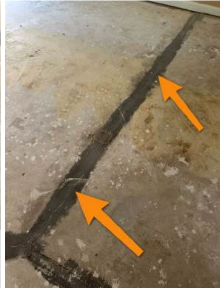
Interior foundation slab cracks observed in lower level right rear bedroom
