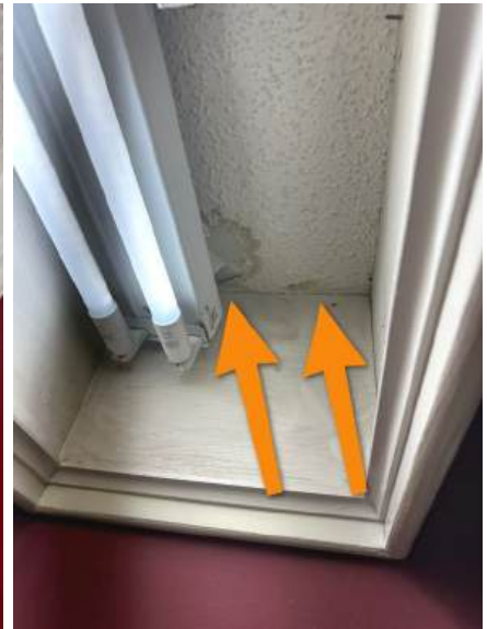
Moisture staining observed on ceiling in main level primary bathroom
