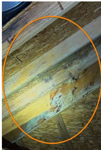
Moisture staining observed on areas of roof framing in front area of attic
