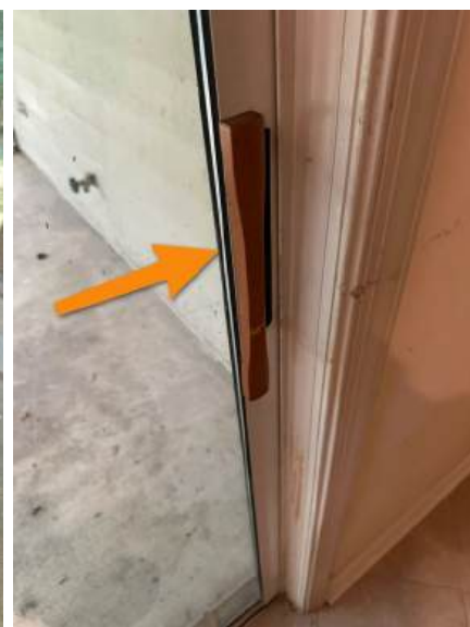
Handle is loose on rear exterior sliding glass door (lower level right rear bedroom)
