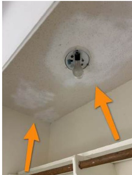
Moisture staining observed on ceiling in laundry area (main level hallway bathroom)
