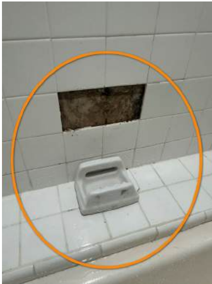
Areas of tile are damaged / detaching and missing in lower level bathroom shower area
