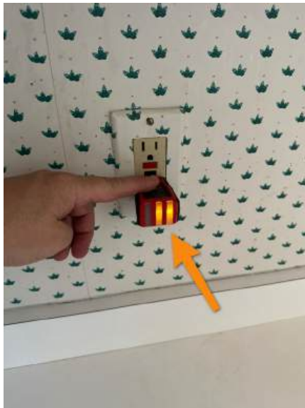
The GFCI receptacle in the did not work/trip off when tested at the time of inspection (Kitchen, left side)
