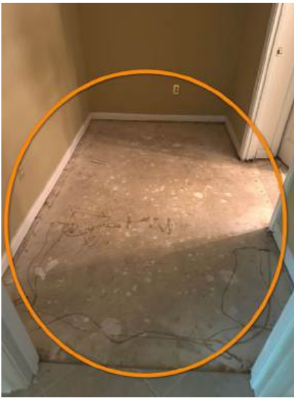
Flooring materials have been removed in numerous locations throughout interior of home (lower level, middle bonus room)
