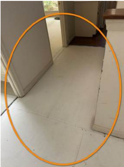
Flooring materials have been removed in numerous locations throughout interior of home (Main level, middle hallway)
