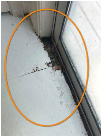
There was evidence of moisture intrusion near or at an exterior door (main level rear exterior sliding glass door, primary bedroom)
