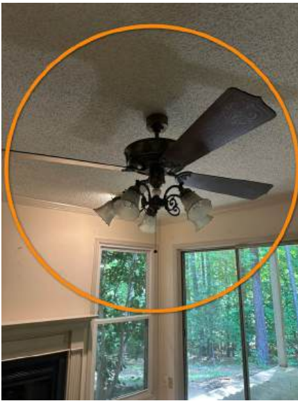
The ceiling fan did not operate in lower level left rear family room during the time of inspection
