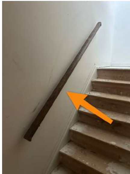
Right side lower handrail is loose on interior stairwell
