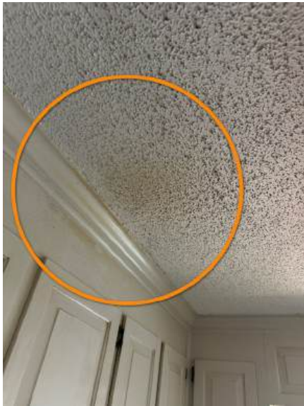
Moisture staining observed on ceiling and right side wall in kitchen
