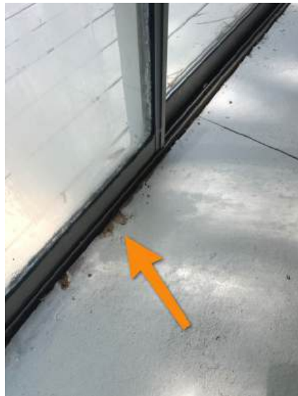
There was an area of deterioration in areas of the subflooring (At rear exterior door, main level primary bedroom)
