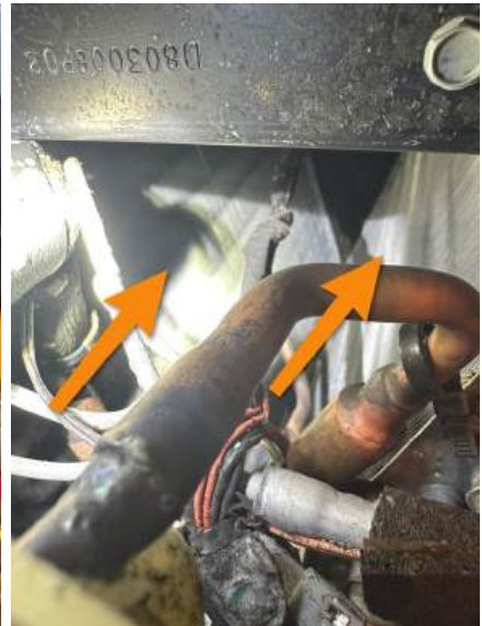
HVAC air handler & evaporator coil need cleaning
