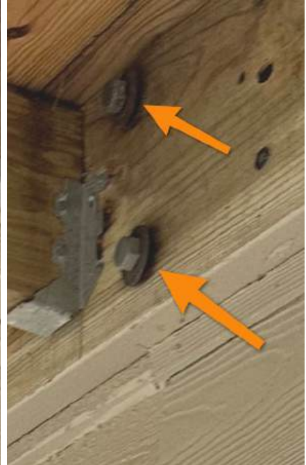
Several ledger board anchor bolts are loose / pulling away on rear deck of home
