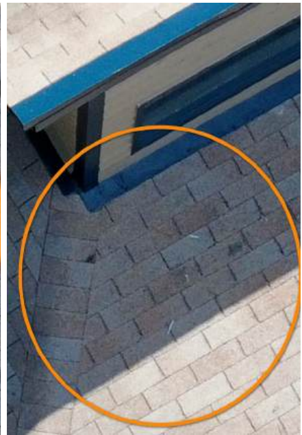
There was mineral granule loss on the roof coverings in several locations
