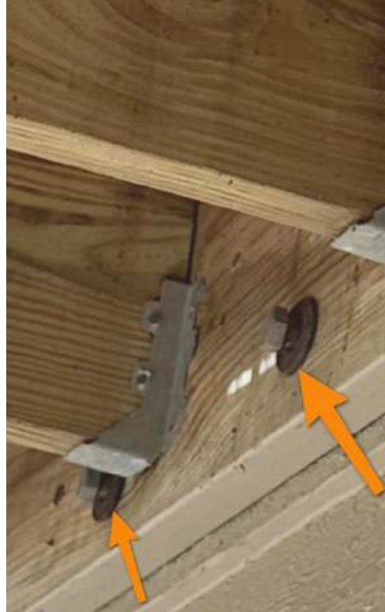
Several ledger board anchor bolts are loose / pulling away on rear deck of home
