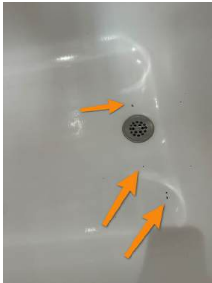
Damage (chipping) observed in areas of tub in main level primary bathroom
