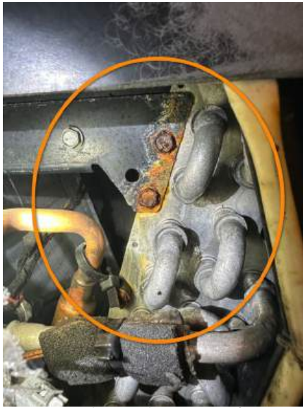
Corrosion observed on areas of evaporator coil in HVAC air handler
