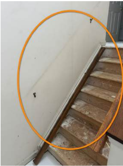
Right side upper handrailing is damaged and has detached on interior stairwell
