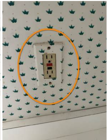
The GFCI receptacle in the did not work/trip off when tested at the time of inspection (Kitchen, right side)
