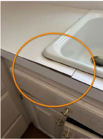
Area of countertop is delaminating at sink in kitchen
