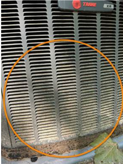
Condenser fins need cleaning on exterior HVAC condenser unit/heat pump
