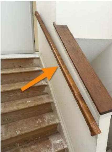
Left side upper handrail is loose on interior stairwell
