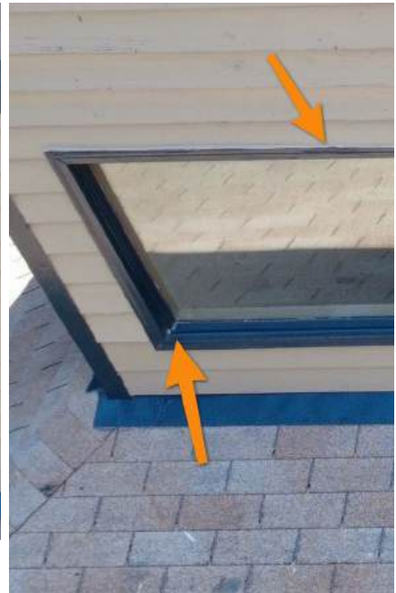
Members of wood around the exterior of the upper fixed windows on right side of home appear to be deteriorated in some areas
