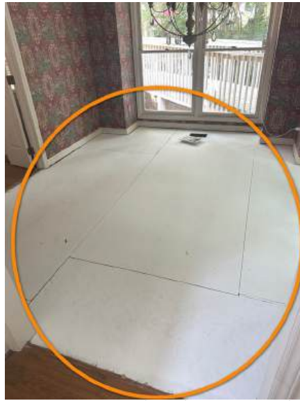
Flooring materials have been removed in numerous locations throughout interior of home (Main level, dining room)
