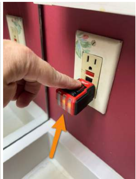
No GFCi protection present in main level primary bathroom electrical receptacle
