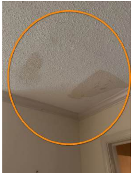
Moisture staining observed on ceiling in lower level hallway
