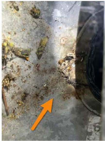
Dirt/debris and suspected organic growth was noted in ductwork and at distribution registers and returns throughout home
