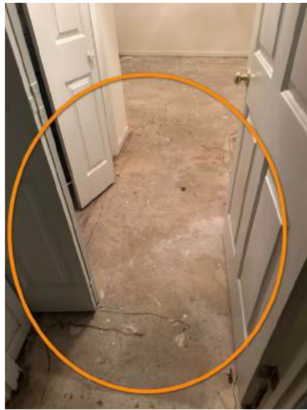
Flooring materials have been removed in numerous locations throughout interior of home (lower level, middle hallway)
