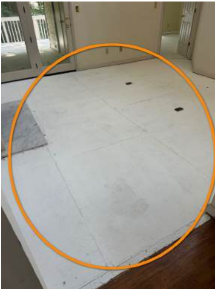
Flooring materials have been removed in numerous locations throughout interior of home (Main level, living room)
