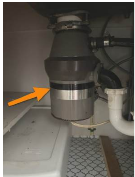
Garbage disposal was inoperable at the time of inspection
