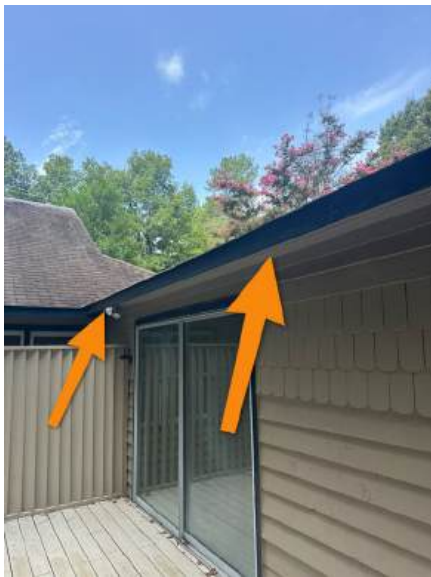
No gutters installed on rear of home
