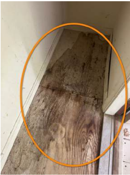
Subflooring had areas of possible moisture intrusion (Rear attached utility closet, main level)
