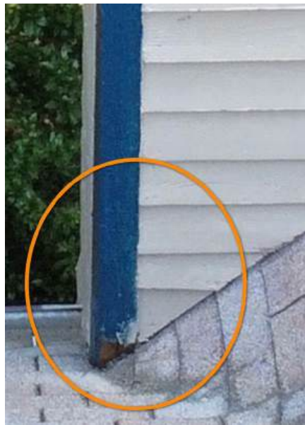
Deterioration observed in areas of siding/trim on left side exterior of home (chimney chase)
