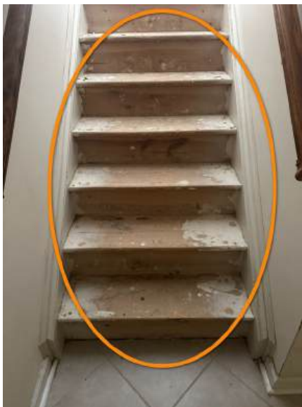
Several step treads are creaky on interior stairwell
