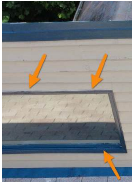
Members of wood around the exterior of the upper fixed windows on right side of home appear to be deteriorated in some areas
