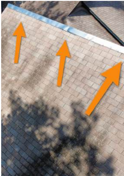
Uplift/gaps in areas of flashing on middle roofing of home
