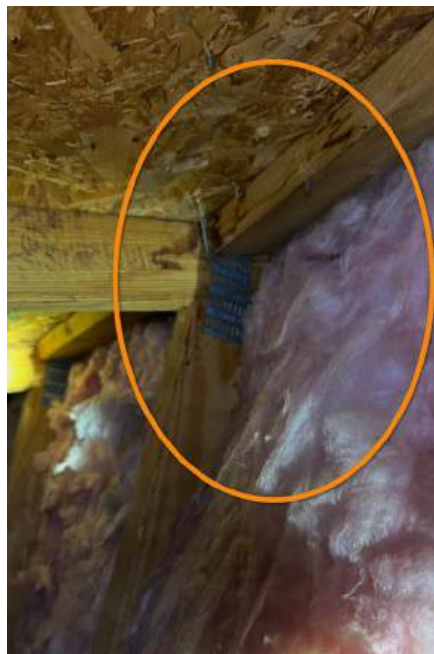
Moisture staining observed on areas of roof and side wall framing in middle right area of attic
