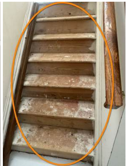
Several step treads are creaky on interior stairwell
