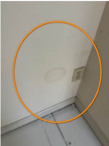
Moisture staining observed on rear wall in main level right front bedroom
