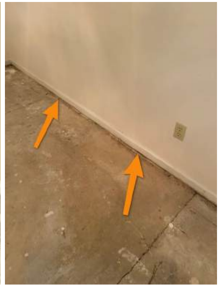
Moisture staining observed on baseboards in several locations throughout lower level of home
