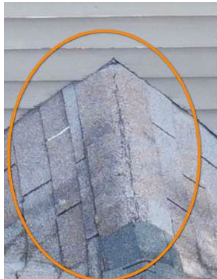
There was mineral granule loss on the roof coverings in several locations
