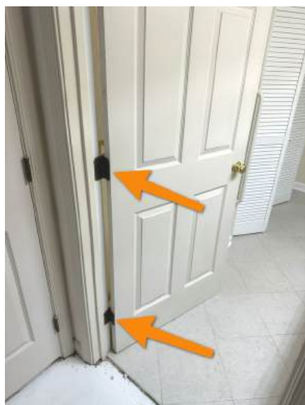
Hinges are loose/detaching on main level hallway bathroom door
