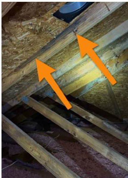
Moisture staining observed on areas of roof framing in front area of attic
