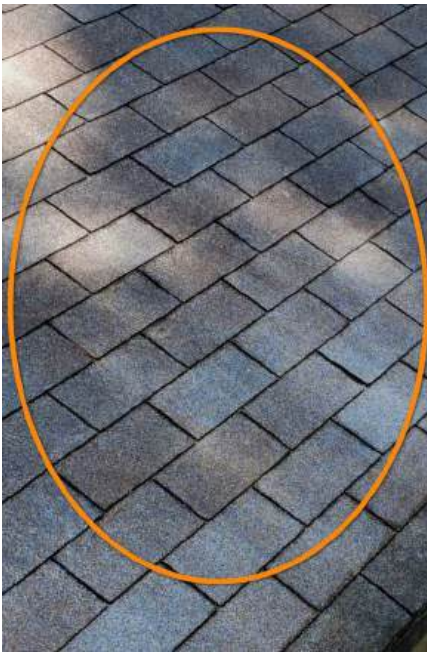
There was mineral granule loss on the roof coverings in several locations
