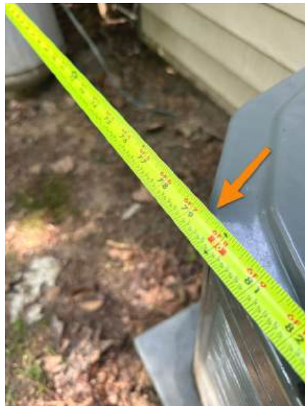
The propane tank has improper clearance from HVAC condenser unit on left side exterior of home (6' 8")
