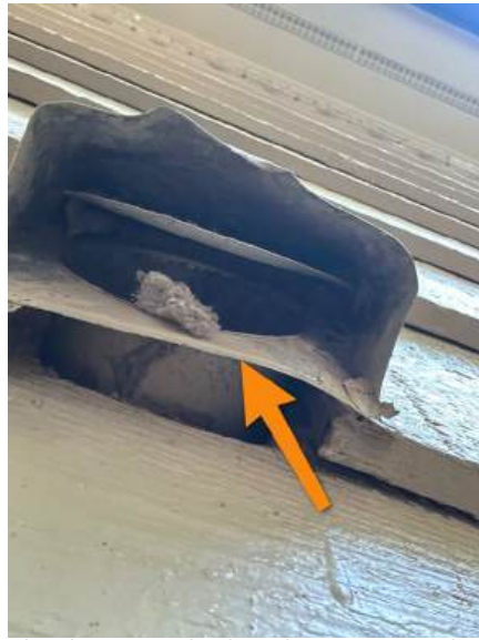
The dryer vent had lint built up on right side exterior of home
