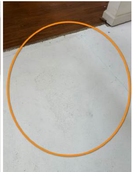
Subflooring had areas of possible moisture intrusion (Main level, living room)
