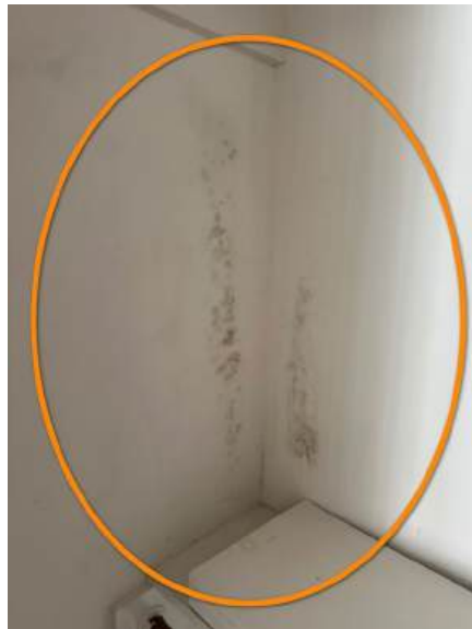
Moisture staining observed on wall in closet of main level right front bedroom
