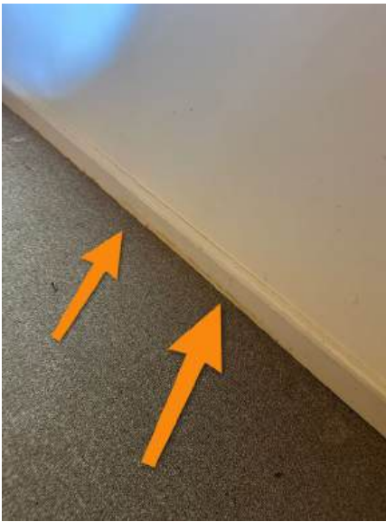
Moisture staining observed on baseboards in several locations throughout lower level of home
