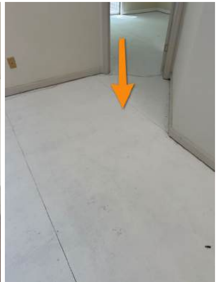
Areas of flooring are creaky on main level of home (living room)
