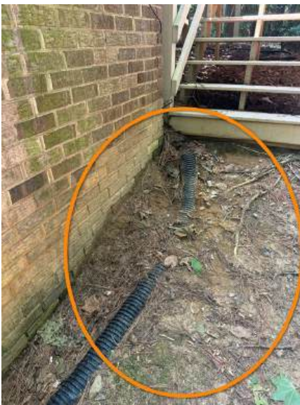
Evidence of soil erosion (left side exterior)
