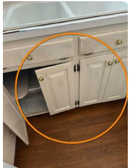
Front facing of cabinet underneath sink in kitchen is loose/detaching
