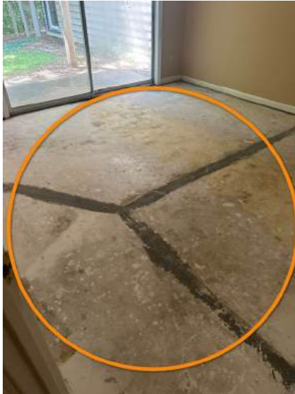
Interior foundation slab cracks observed in lower level right rear bedroom
