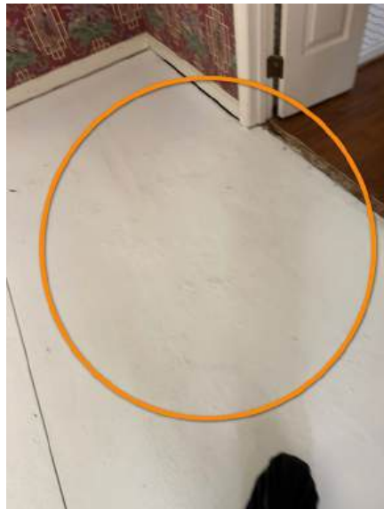
Subflooring had areas of possible moisture intrusion (Main level, dining room)
