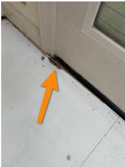
There was evidence of moisture intrusion near or at an exterior door (main level rear exterior door, living room)
