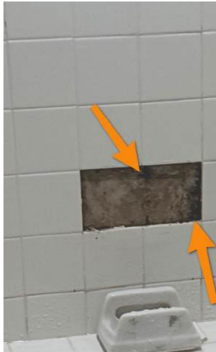
Suspected organic growth of based on wall sheathing where tiles are missing in shower area of lower level bathroom
