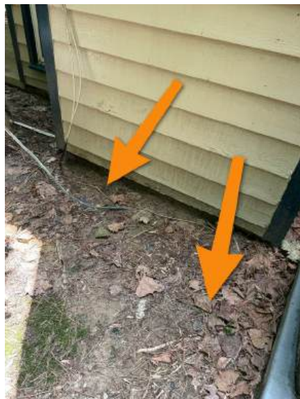
Evidence of soil erosion (left side exterior)
