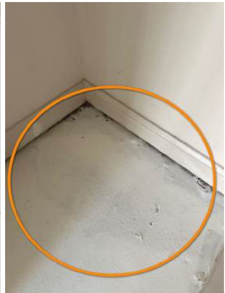
There was an area of deterioration in areas of the subflooring (in closet, main level right front bedroom)
