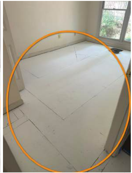
Flooring materials have been removed in numerous locations throughout interior of home (Main level, right front bedroom)
