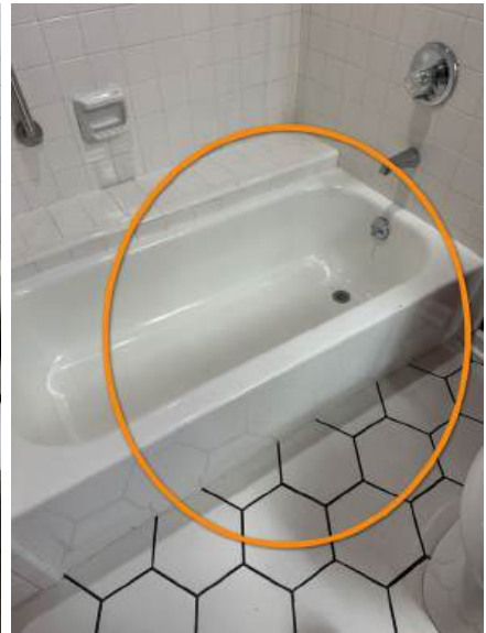
Damage (chipping) observed in areas of tub in main level primary bathroom
