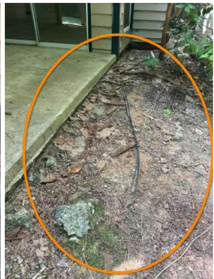
Evidence of soil erosion (left side exterior)
