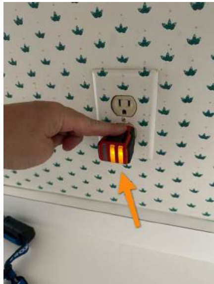
No GFCi protection present in kitchen electrical receptacles
