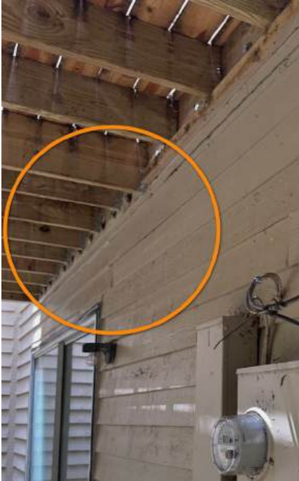
Several ledger board anchor bolts are loose / pulling away on rear deck of home
