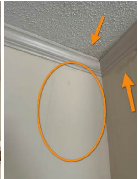
Moisture staining observed on rear wall and ceiling in main level right front bedroom
