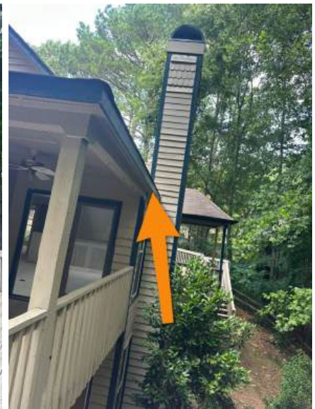
No gutters installed on left side rear of home
