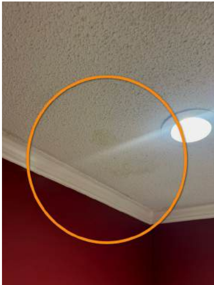
Moisture staining observed on ceiling in main level primary bathroom
