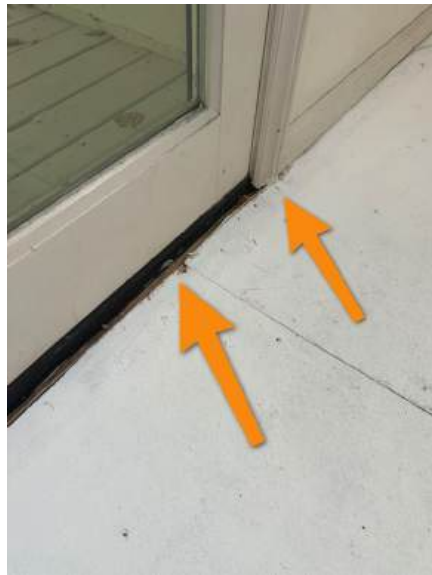
There was an area of deterioration in areas of the subflooring (At rear exterior door, main level living room)
