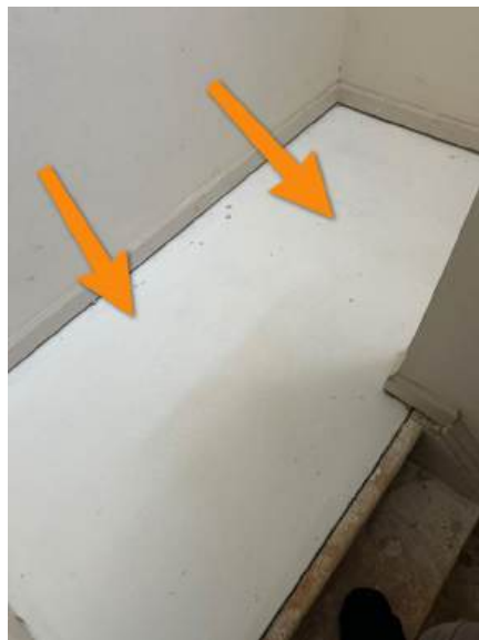
Flooring is creaky on middle stairwell landing
