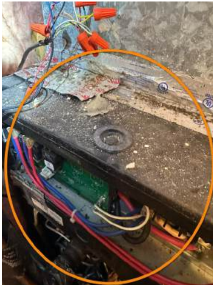
HVAC air handler & evaporator coil need cleaning
