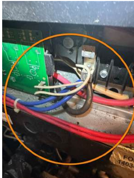
HVAC air handler & evaporator coil need cleaning
