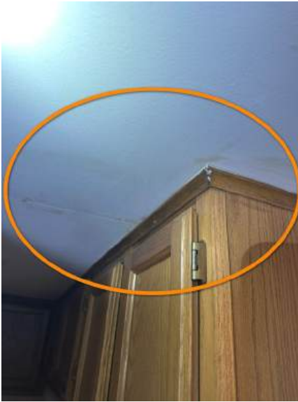
Moisture staining observed on ceiling in lower level front bonus room
