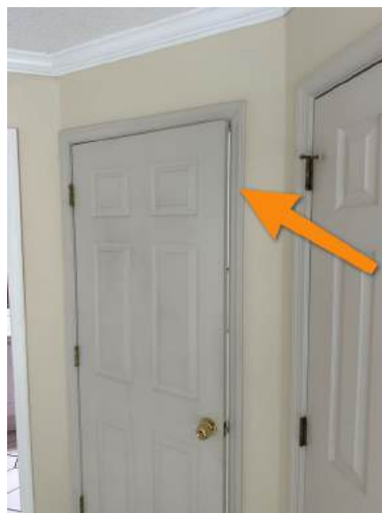
Main level primary bedroom door is binding against frame at top when closed
