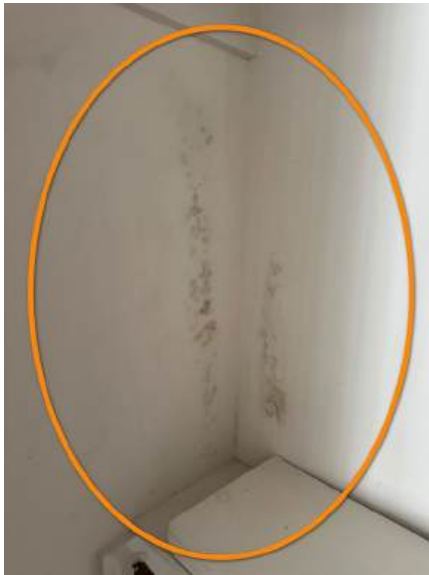
Suspected organic growth observed on walls in main level right front bedroom closet
