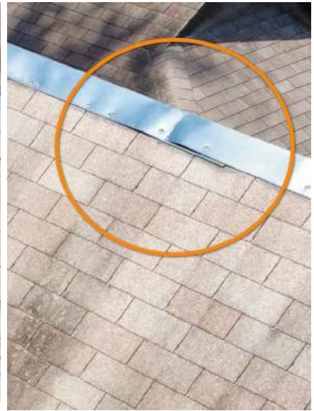
Uplift/gaps in areas of flashing on middle roofing of home
