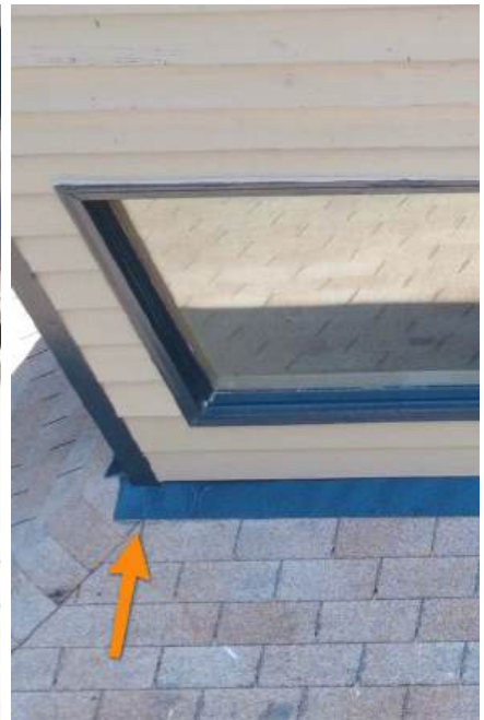
Uplift/gaps in areas of flashing on middle roofing of home
