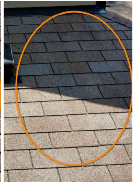
There was mineral granule loss on the roof coverings in several locations
