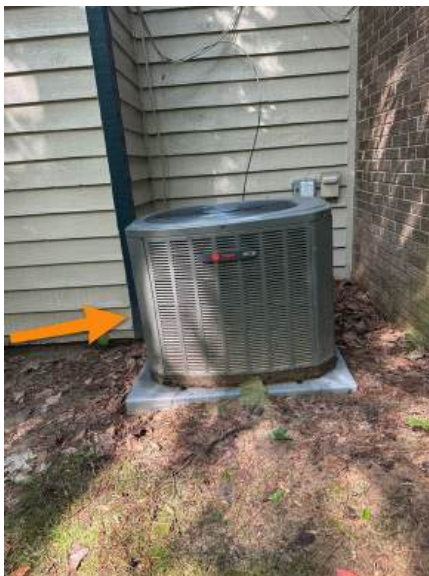
Exterior HVAC condenser unit/heat pump is not sitting level
