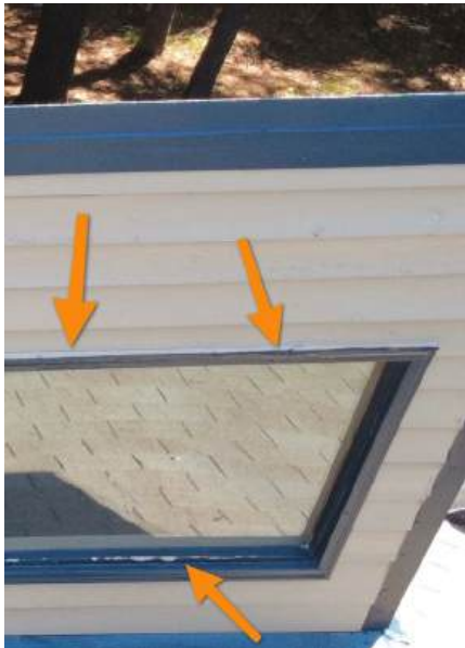
Members of wood around the exterior of the upper fixed windows on right side of home appear to be deteriorated in some areas
