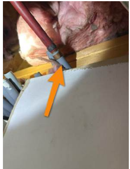
This home has a plumbing supply system that partially uses polybutylene plastic distribution lines and compression band fittings
