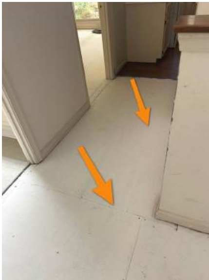
Areas of flooring are creaky on main level of home (middle hallway)
