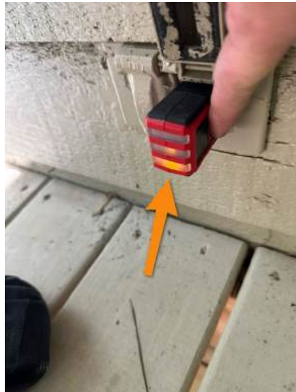
No GFCI protection in exterior electrical receptacles
