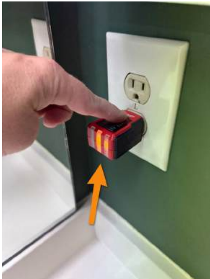
No GFCi protection present in lower level bathroom electrical receptacle
