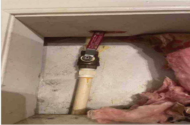
Main water shut off located in the basement
