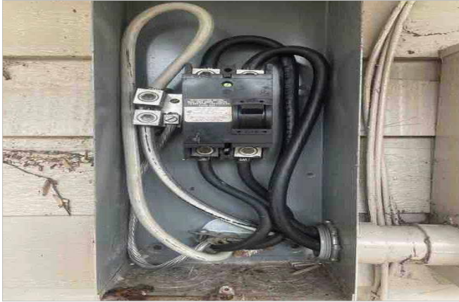
Inside of main electrical panel
