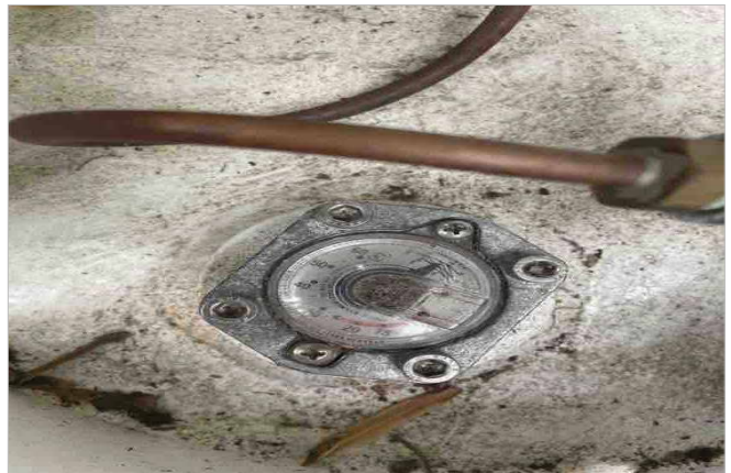
Propane tank guage
