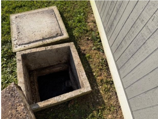
Home shown encroaching on septic tank
