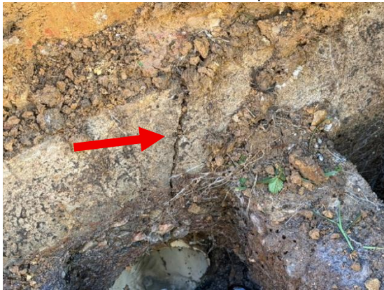
Crack shown on backside of septic tank
