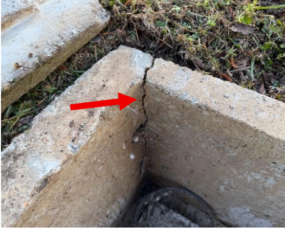
Pump chamber riser shown with crack
