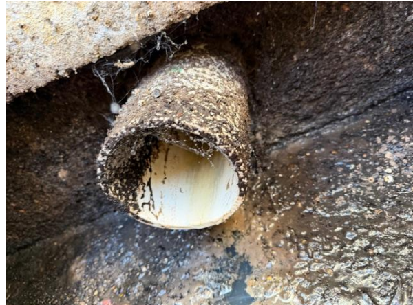
Inlet drain pipe shown
