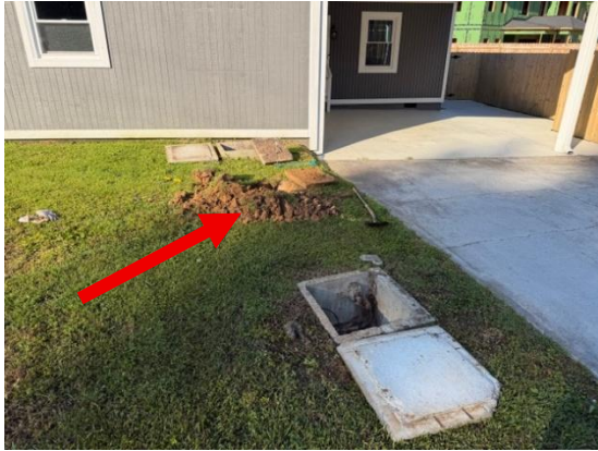
Outlet chamber location shown
