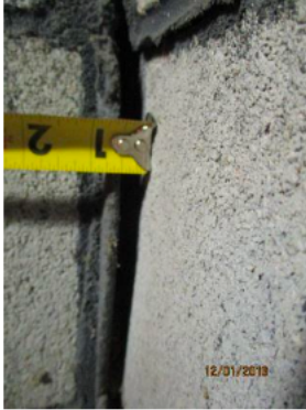
Interior Foundation: crack/separation back left corner
