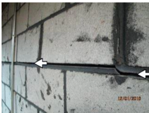
Interior Foundation: horizontal crack, note separation
