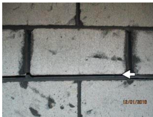
Interior Foundation: horizontal crack, note separation
