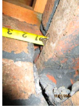
Interior Foundation: crack/separation back left corner
