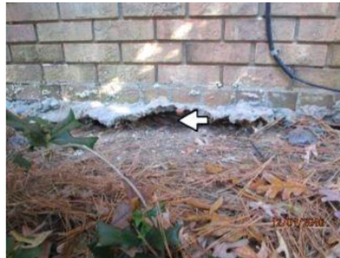
Exterior Surfaces & Eaves: brick veneer not supported
