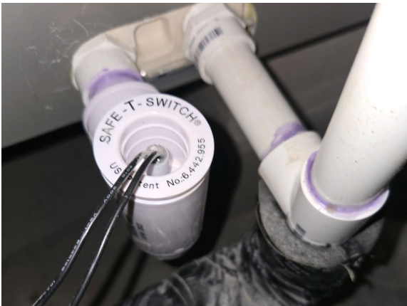
Secondary Drain Switch
