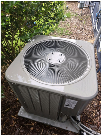
Condenser Coil Before (Clean)
