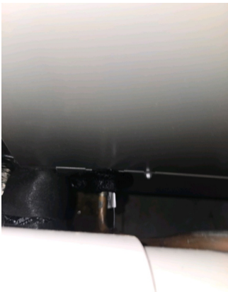
Solder/Braze Joints (Evaporator)
