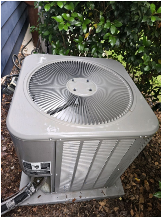
Condenser Coil After (Clean)
