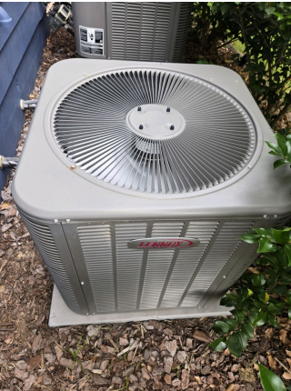
Condenser Coil Before (Clean)
