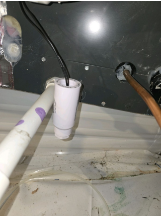
Secondary Drain Switch
