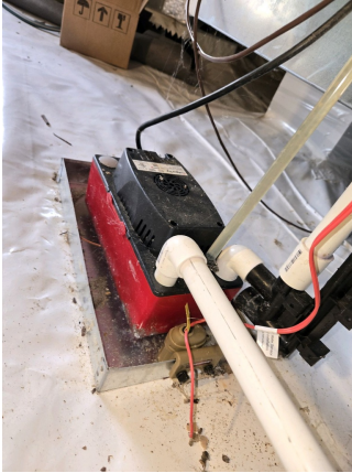
Condensate Pump GFI
