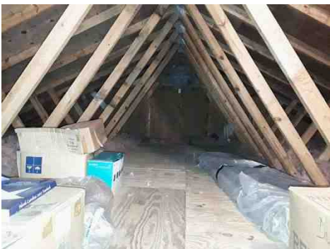
Attic Drop Stair
