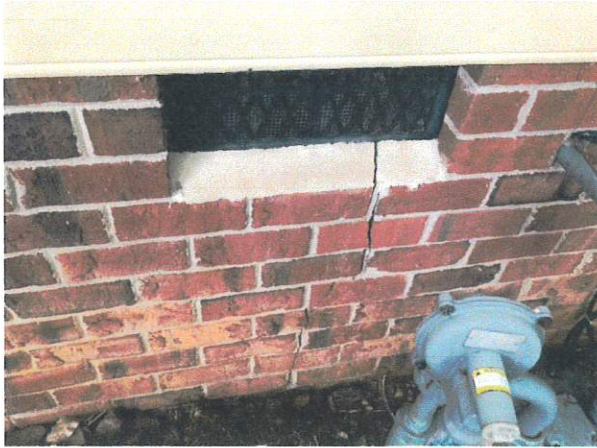
Crack in brick veneer under crawlspace vent on right side
