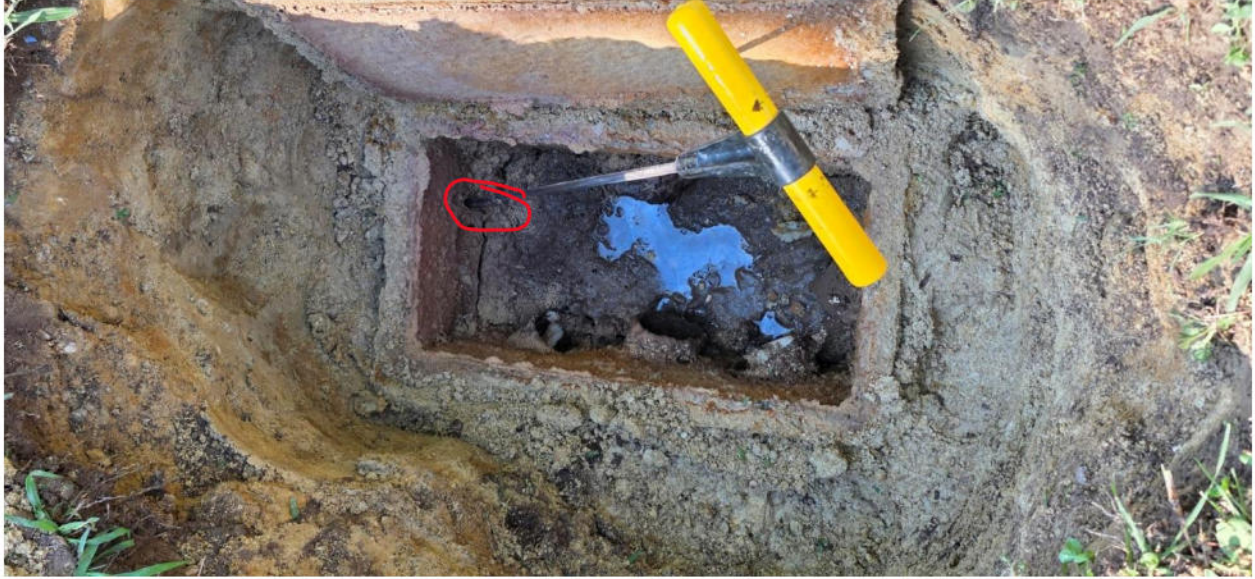
This is the distribution box. It is corroded and needs to be replaced.
