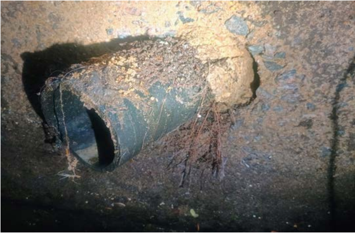
Separation around inbound pipe should be resealed
