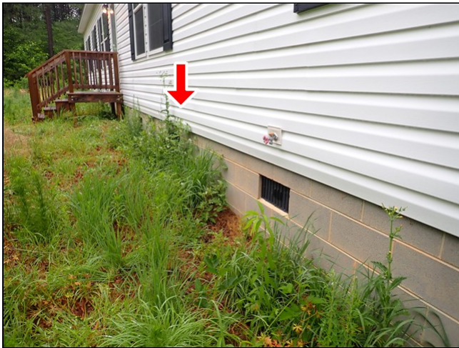
2.4 Item 1(Picture) Vegetation too close to house
