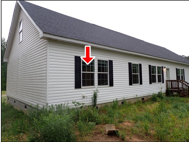
2.2 Item 1(Picture) Broken window glass
