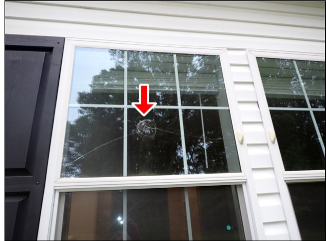
2.2 Item 2(Picture) Close up of broken window glass
