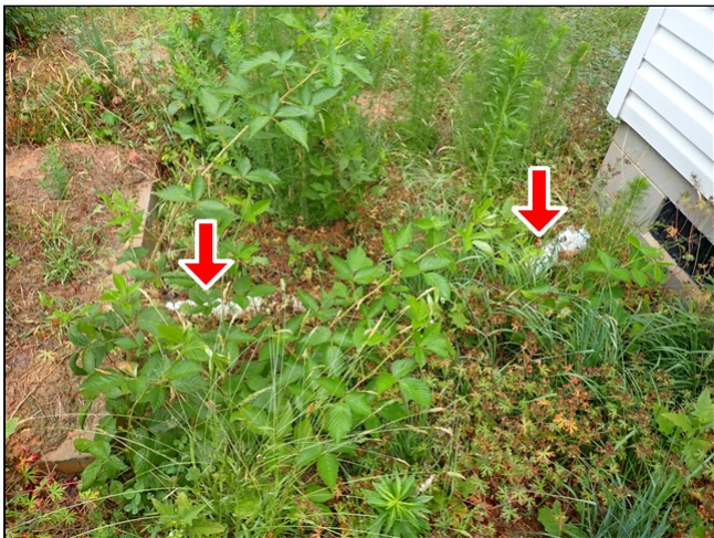
4.0 Item 1(Picture) Exposed drain pipe
