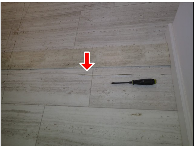
8.3 Item 6(Picture) Close up of separated vinyl flooring
