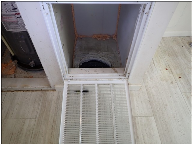
7.0 Item 2(Picture) Missing filter
