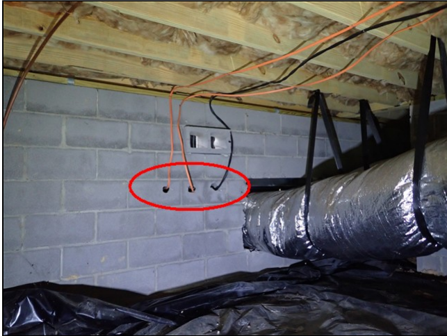
5.2 Item 1(Picture) Cables without conduit
