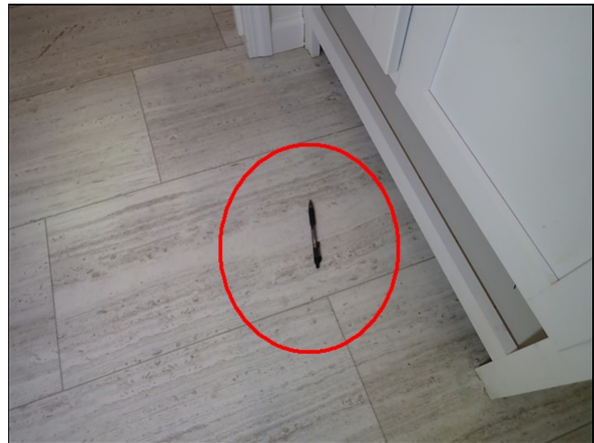
1.2 Item 2(Picture) Close up of soft subfloor
