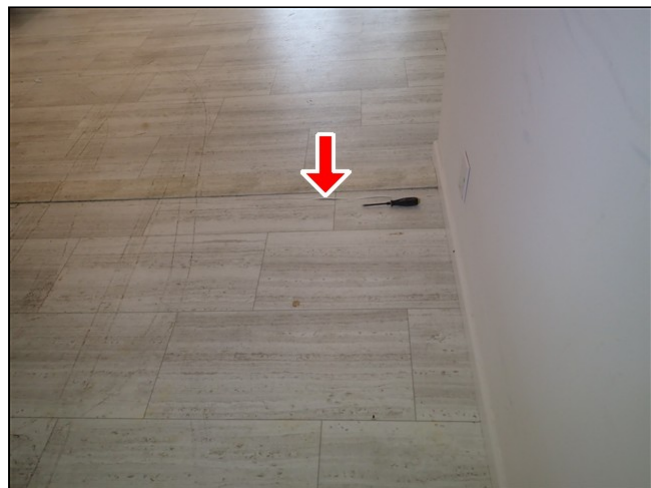
8.3 Item 5(Picture) Separated vinyl flooring
