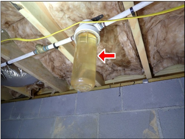
4.1 Item 6(Picture) Missing cartridge
