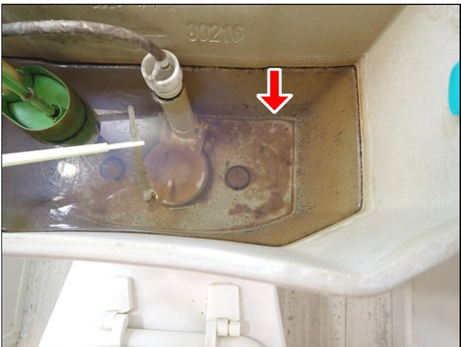
4.1 Item 2(Picture) Sediment in toilet tank
