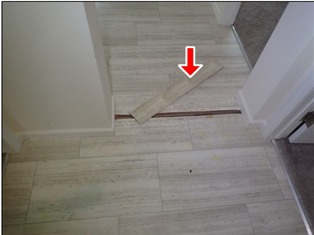
8.3 Item 1(Picture) Loose threshold
