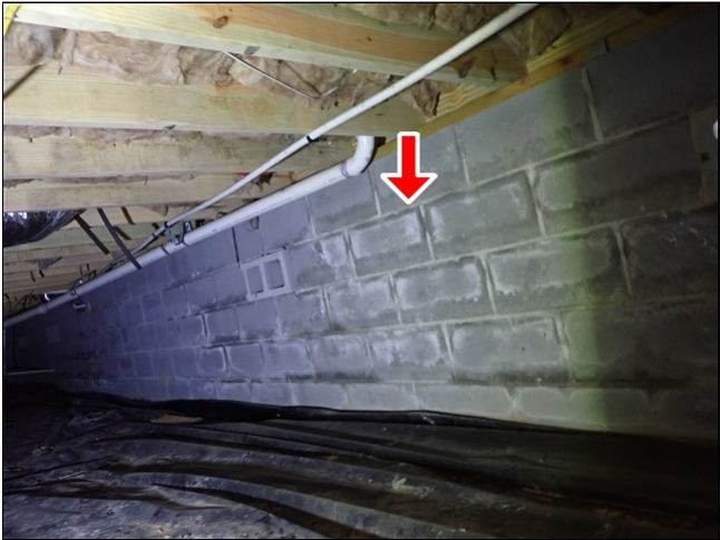
1.0 Item 8(Picture) Efflorescence
