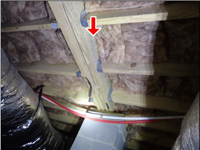
1.0 Item 6(Picture) Fungal growth
