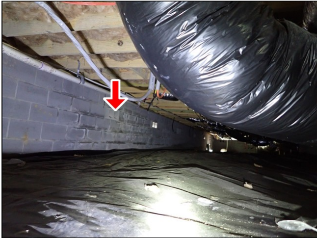
1.0 Item 7(Picture) Efflorescence
