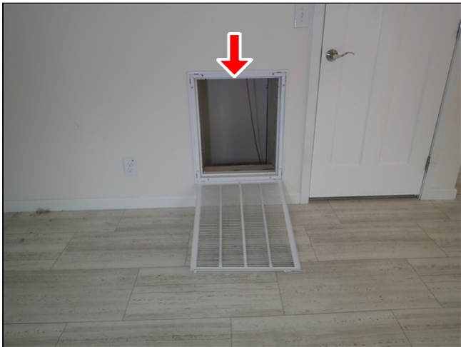
7.0 Item 1(Picture) Missing filter
