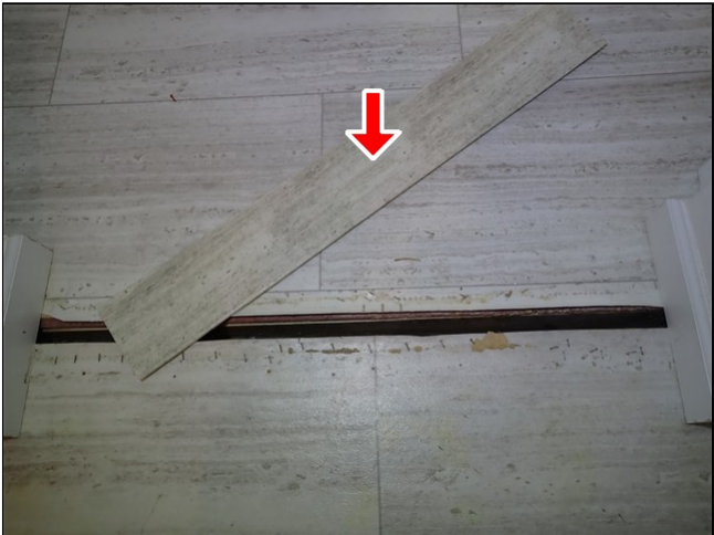
8.3 Item 2(Picture) Close up of loose threshold
