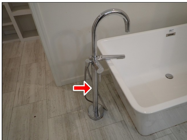
4.4 Item 5(Picture) Loose faucet
