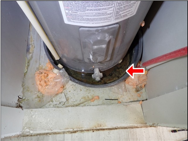
4.3 Item 2(Picture) Water in drip pan
