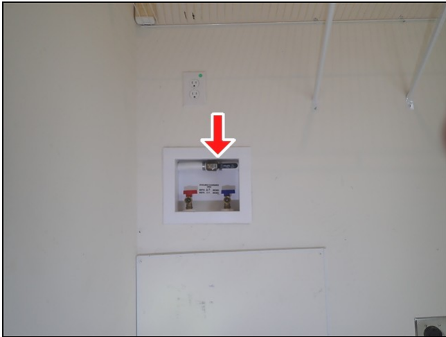
4.2 Item 1(Picture) Main water shut off valve
