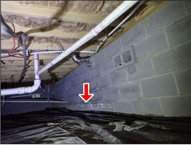
1.0 Item 9(Picture) Efflorescence
