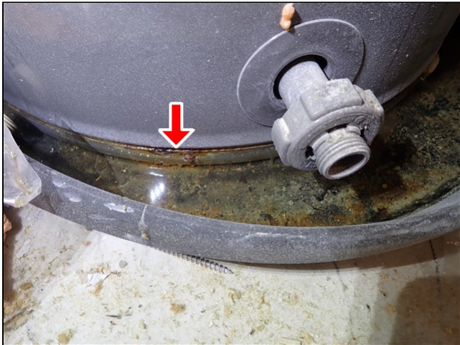
4.3 Item 3(Picture) Rusted metal
