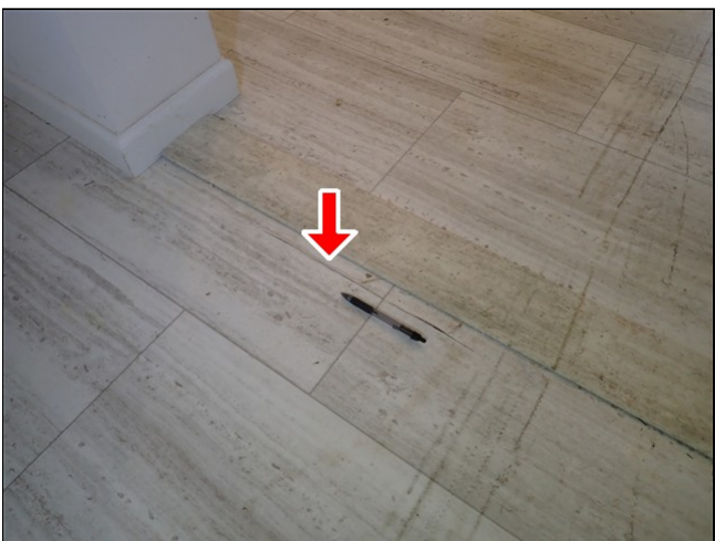
8.3 Item 4(Picture) Close up of separated vinyl flooring
