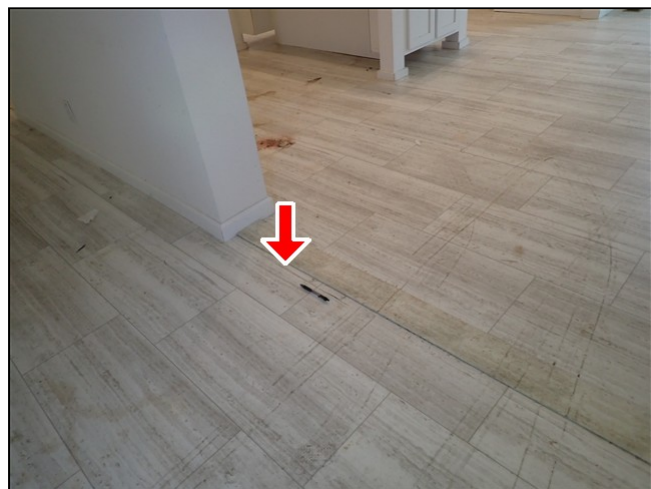
8.3 Item 3(Picture) Separated vinyl flooring
