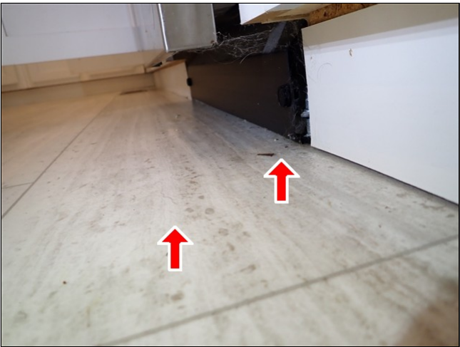
10.0 Item 2(Picture) Puddled water
