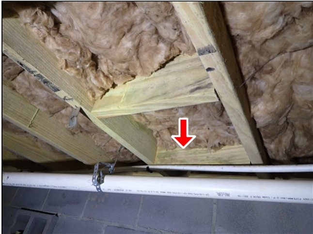
1.0 Item 5(Picture) Fungal growth
