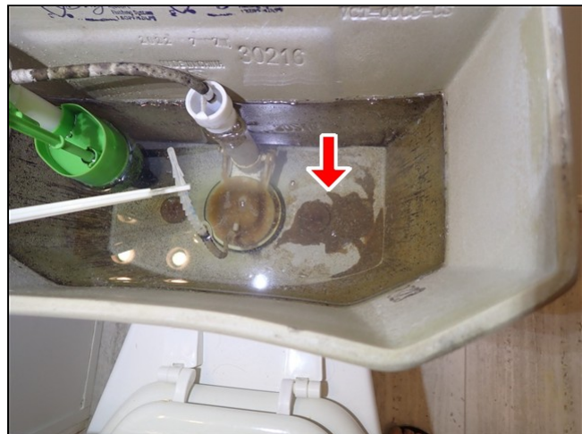
4.1 Item 1(Picture) Sediment in toilet tank
