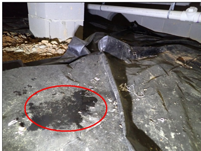
4.4 Item 4(Picture) Puddled water
