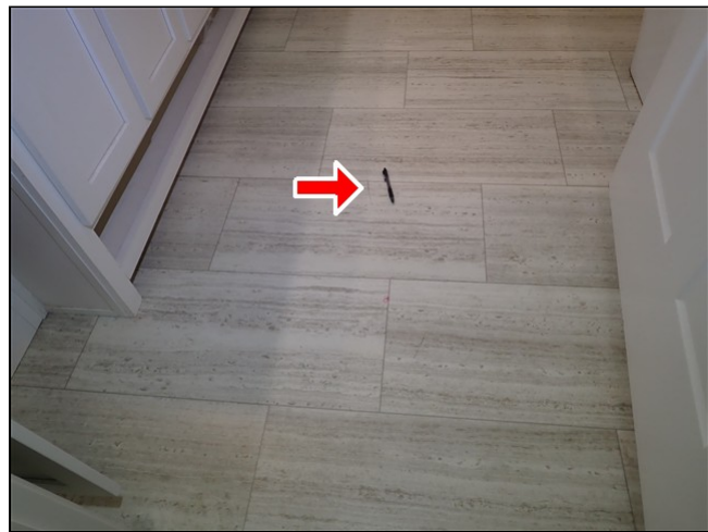
8.3 Item 7(Picture) Torn vinyl flooring
