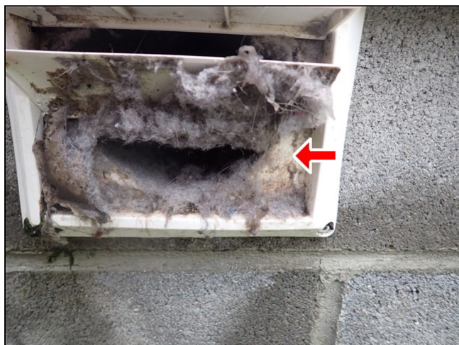
9.4 Item 2(Picture) Lint in dryer exhaust vent
