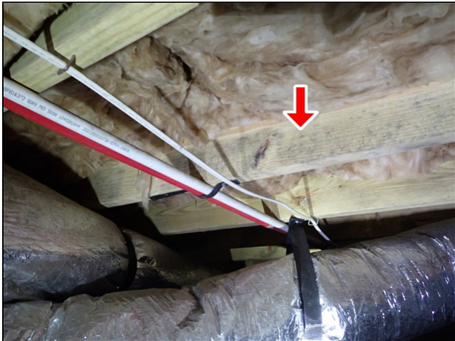
1.0 Item 3(Picture) Fungal growth
