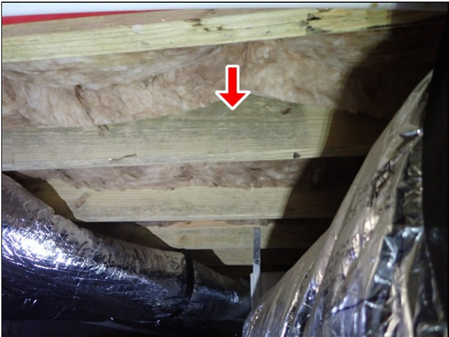
1.0 Item 4(Picture) Fungal growth
