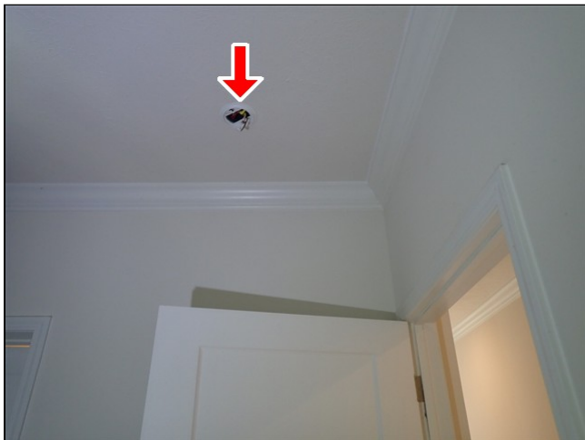
5.6 Item 1(Picture) Missing cartridge
