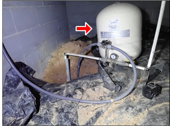
4.1 Item 8(Picture) Pressure tank
