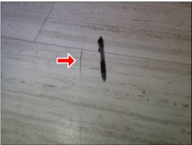
8.3 Item 8(Picture) Close up of torn vinyl flooring
