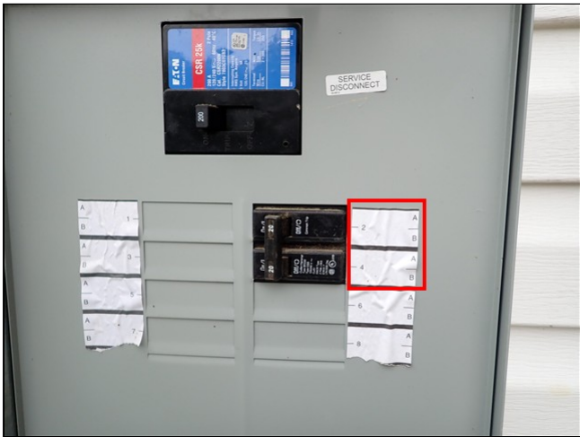
5.1 Item 1(Picture) Breaker lacks labels
