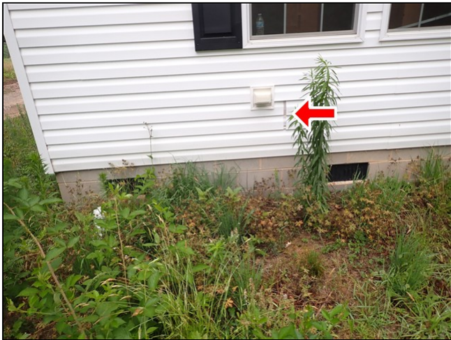
2.0 Item 1(Picture) Gap between vinyl siding
