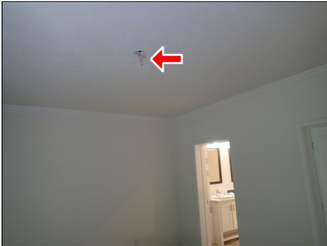
5.2 Item 2(Picture) Bare conductors
