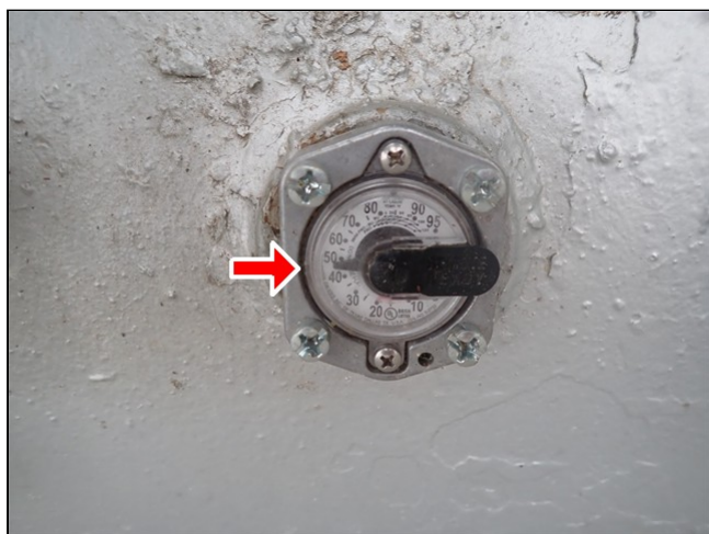
4.8 Item 1(Picture) Propane tank approximately 45% full
