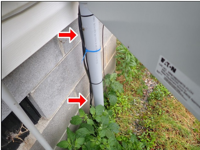
5.2 Item 4(Picture) Conductors without conduit
