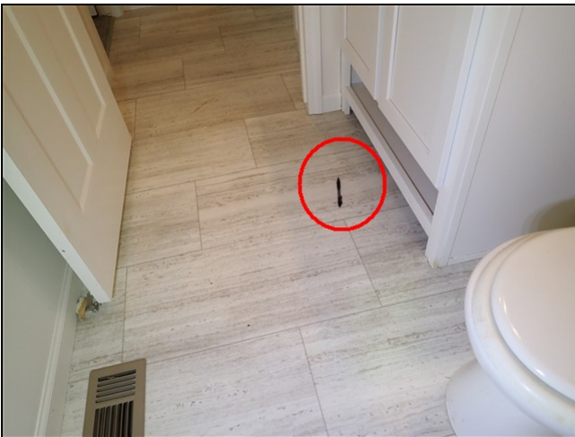
1.2 Item 1(Picture) Soft subfloor
