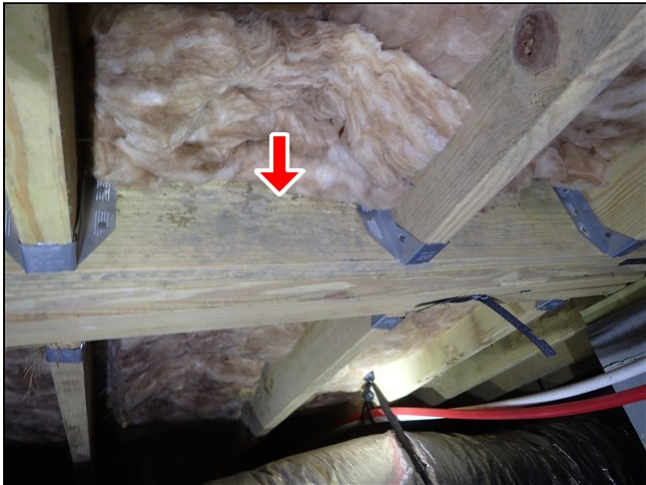
1.0 Item 1(Picture) Fungal growth
