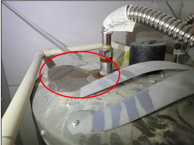
4.3 Item 1(Picture) Leak at water heater
