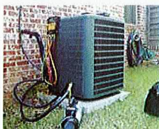
Pre-season HVAC tune ups
