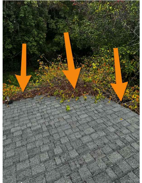
Significant decay is expected in all areas of the roof and wall where plant growth like this is located.
