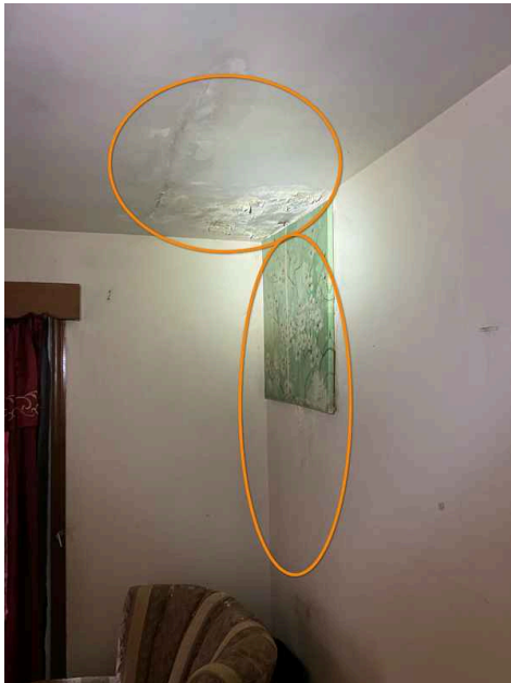
See description for this finding located in the living room.
