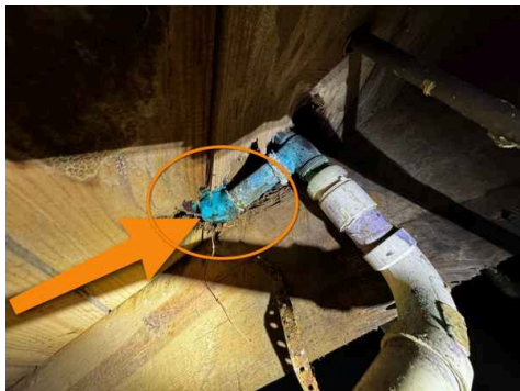
The drain under the tub is leaking.
