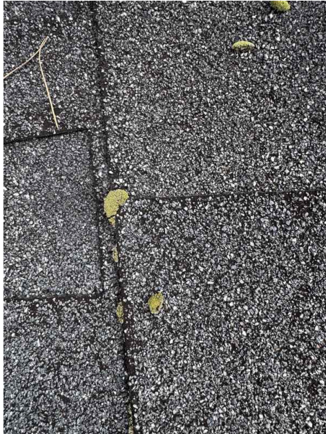
Additional photo of this finding.
