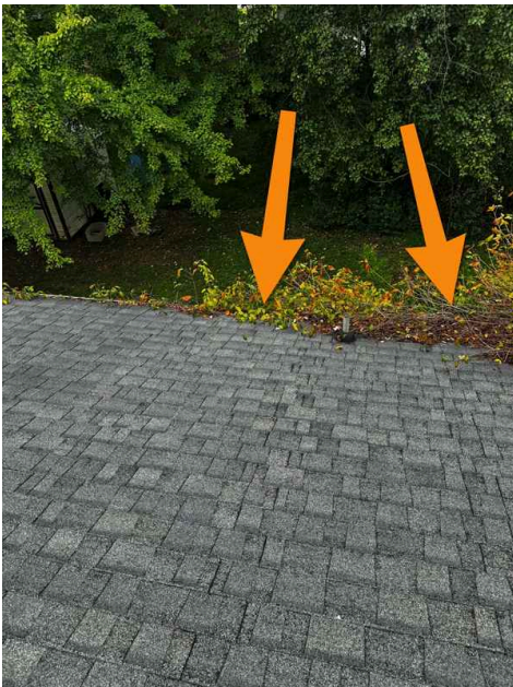
Additional photo of this finding.
