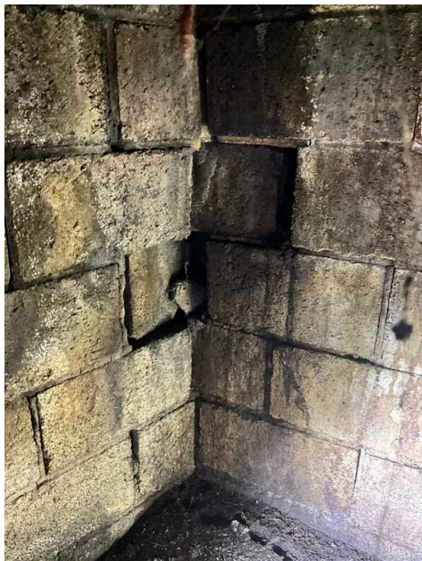
The first place is damaged. This exposes structure though to excessive heat which is a fire hazard.
