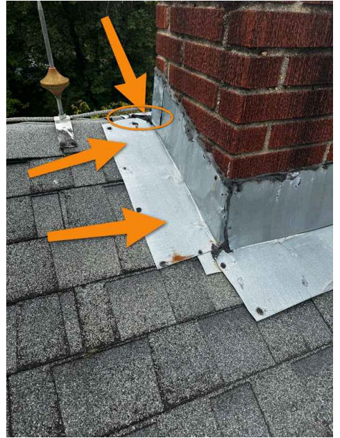
Additional photo of this finding. The flashing on the sides should be under the shingles.
