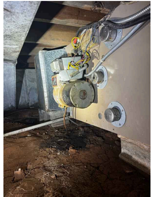
The furnace side was not functional. See flue section of the report.
