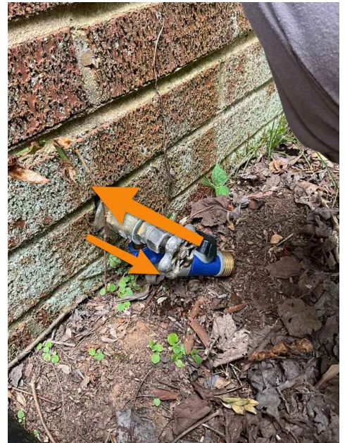
Located on the front of the home. Also the hose bib leaks.
