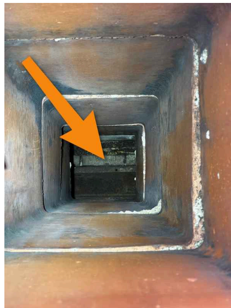
Rainwater falls directly into the fireplace.
