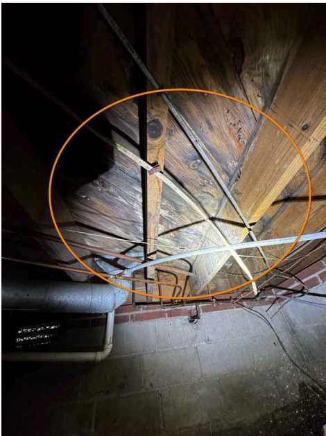
The area in the crawlspace was the most water damage was under the kitchen.
