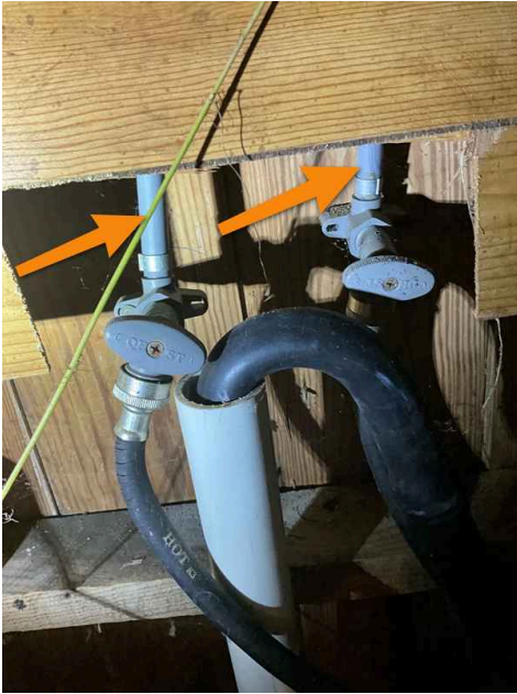
See description for this finding located behind the washing machine.
