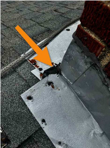
This is a hole and roof leak in the flashing.
