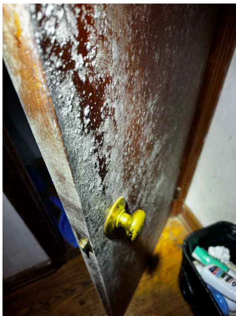
Additional photo of this finding.
