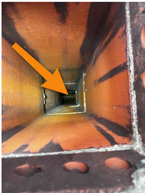
Water flows directly into the crawlspace.
