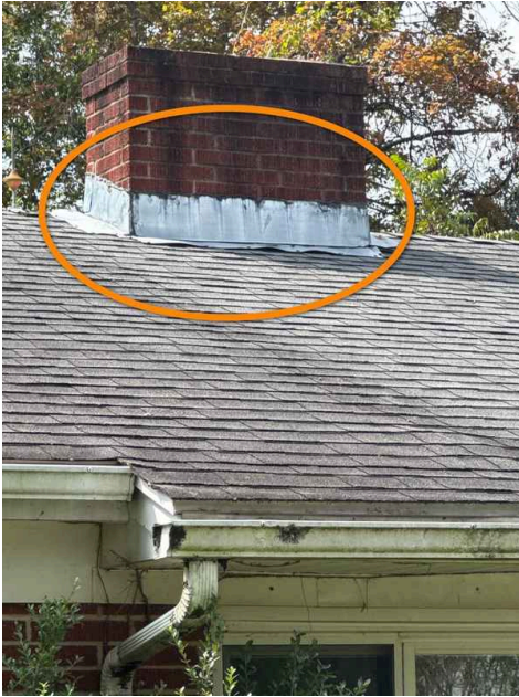
The flashing is not installed correctly and is loose in all areas around the chimney.
