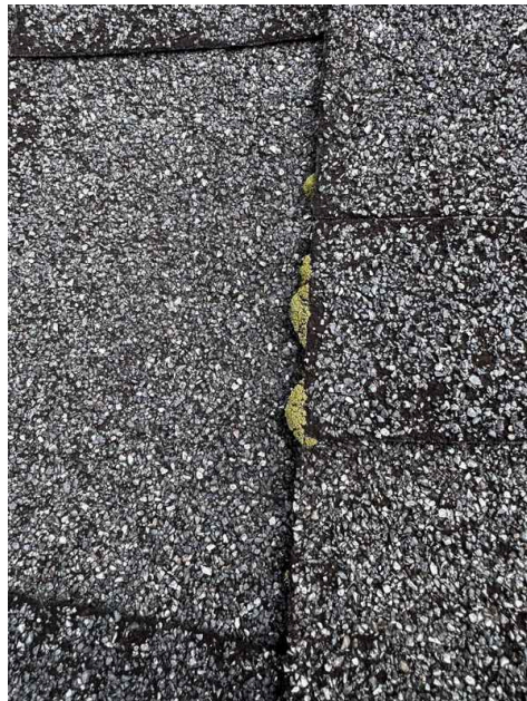
Moss was growing in many areas caused by excessive heat in the attic.
