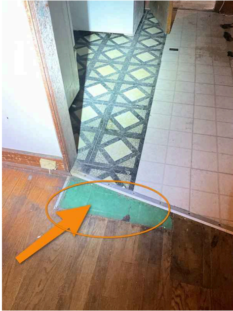
The smaller 7 inch tile are typically asbestos tile.
