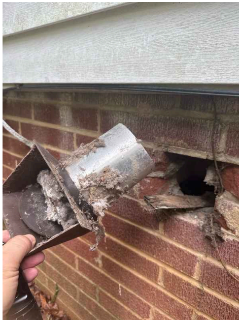
The duct is completely disconnected.
