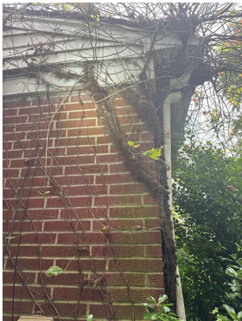
Large plants are growing into the structure of the home and coming out of the roof. Hidden damage throughout his present.
