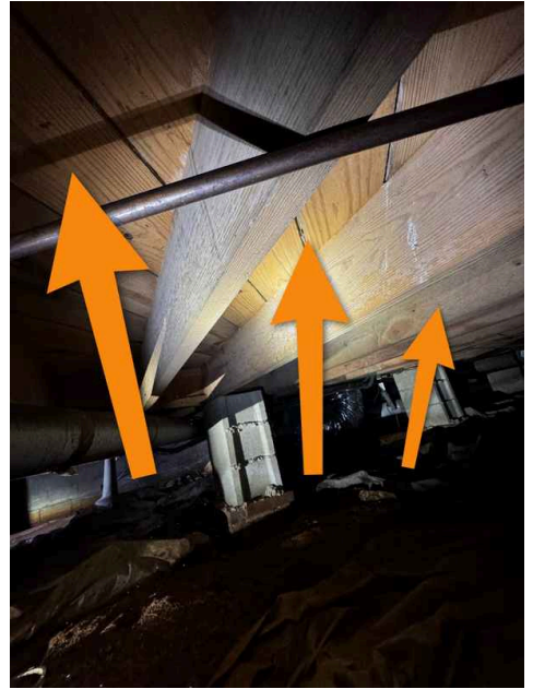
Additional photo of this finding.
