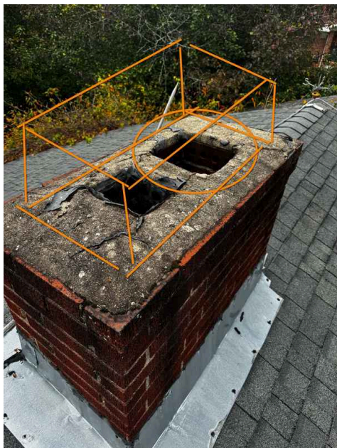
Additional photo of this finding. Also the box that prevents water entry is missing.
