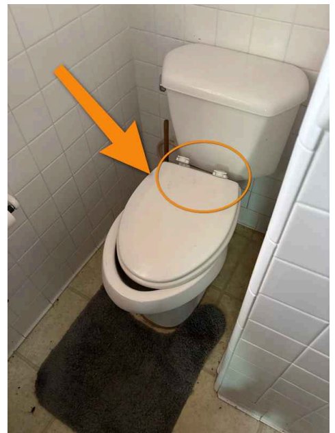
The toilet seat is not installed.
