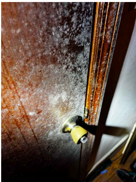
See description and following photos. Mold was found on surfaces throughout the home caused by long-term leakage
