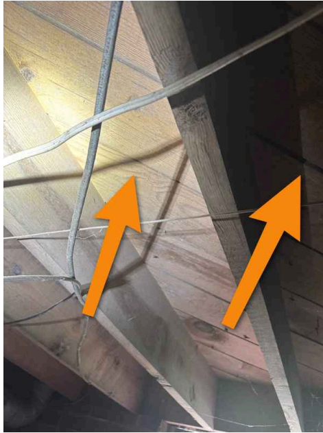
Additional photo of this finding. there is no insulation under any part of the home.
