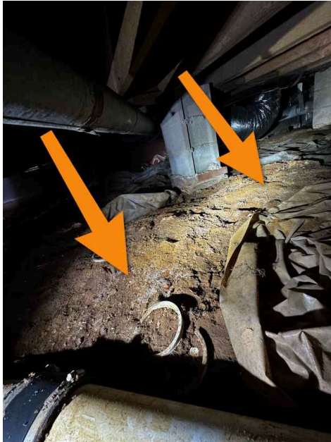
The vapor bar was missing in the majority of areas of the crawlspace.
