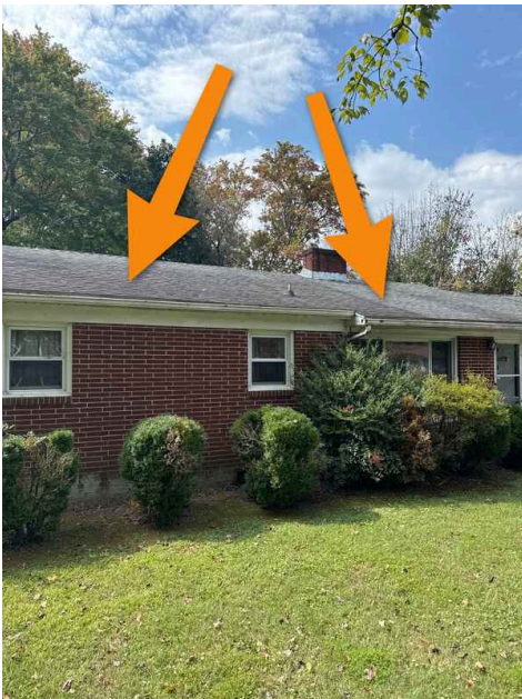
The roof is showing signs of heat damage caused by a lack of ventilation.
