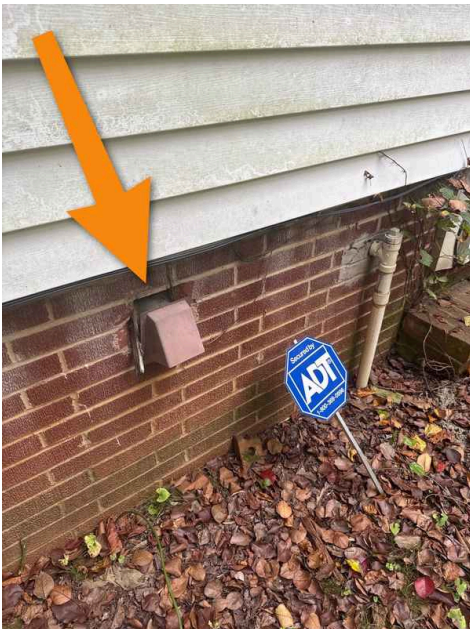
The dryer duct is loose and damaged.
