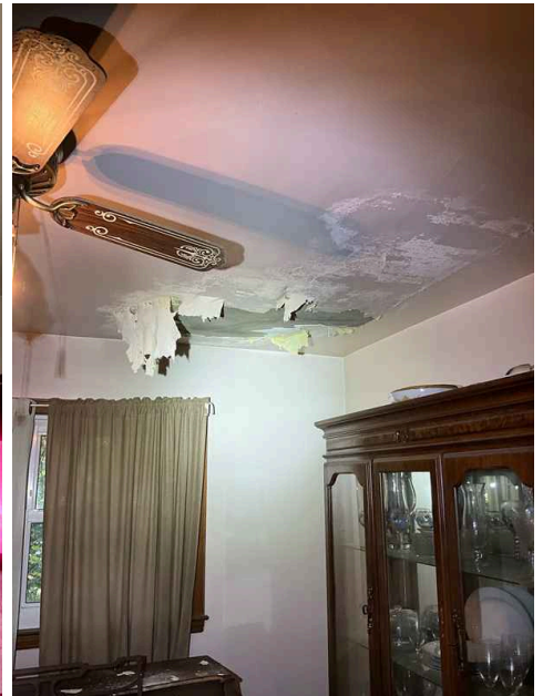
Similar findings were found here. This was a long term leak with significant damage.
