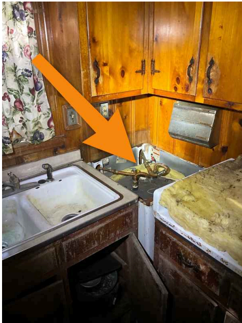
See description for this finding located is in the kitchen.
