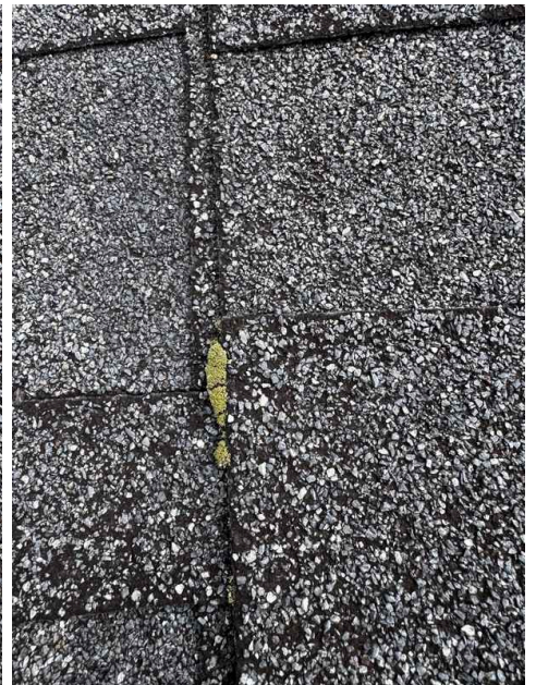
Additional photo of this finding.
