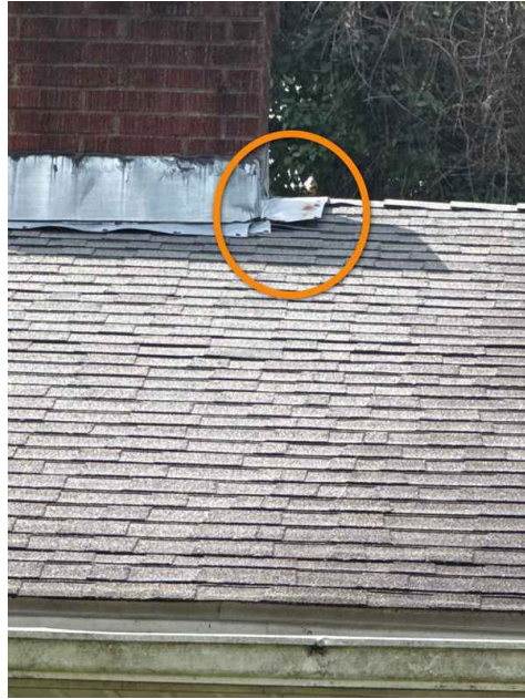
Loose and improper installation creates active roof leaks.
