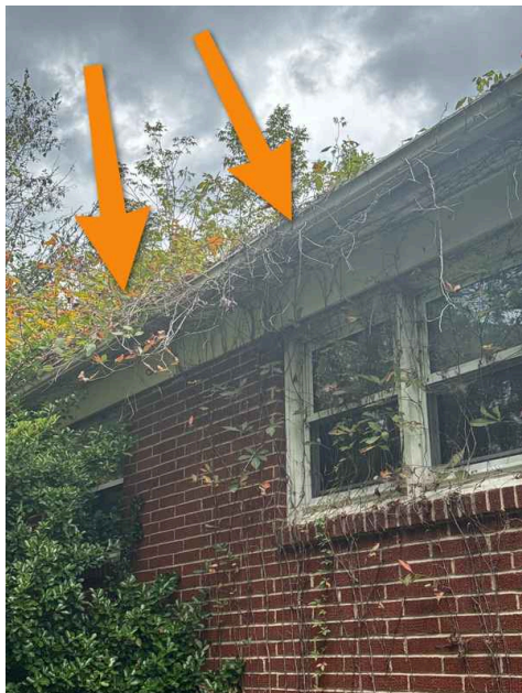
Hidden damage through all areas of the roof structure is expected.
