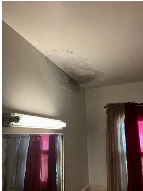
Additional photo of this finding from the bathroom. Mold is present and also likely inside the wall.
