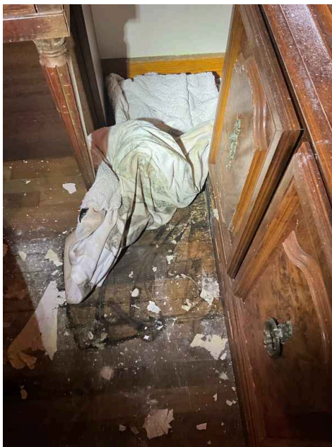
Additional photo of this finding below showing mold and damage.
