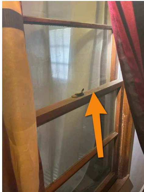
This window does not align properly and shut properly.
