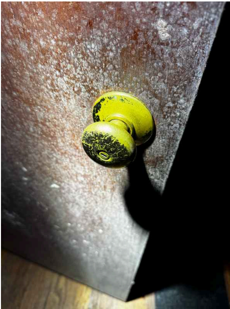
Additional photo of this finding.
