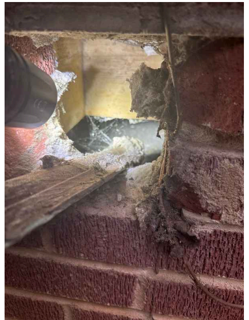
This means the hot humid air from the dryer is being directed under the carport addition.
