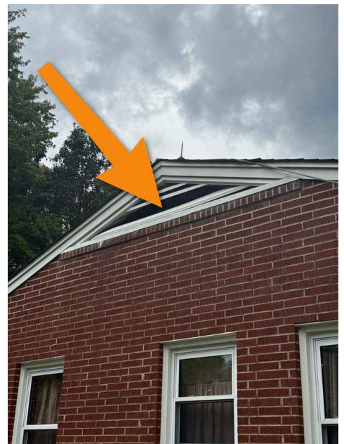
The damaged gable allows animals to enter the structure of the home.
