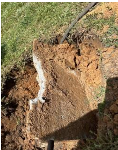
DAMAGED OUTLET LID
