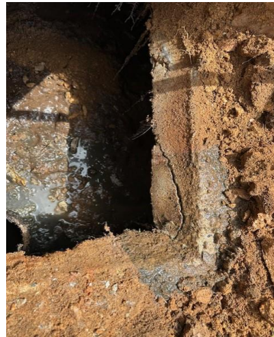
CRACK ON OUTLET TANK
