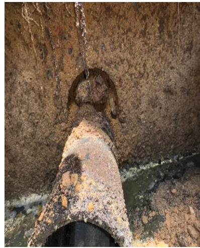
2" HOLE AROUND INLET PIPE
