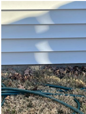
Picture 3 – Foundation crack
