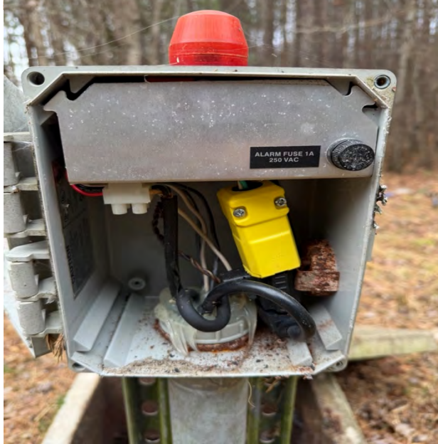
Inside of pump tank
