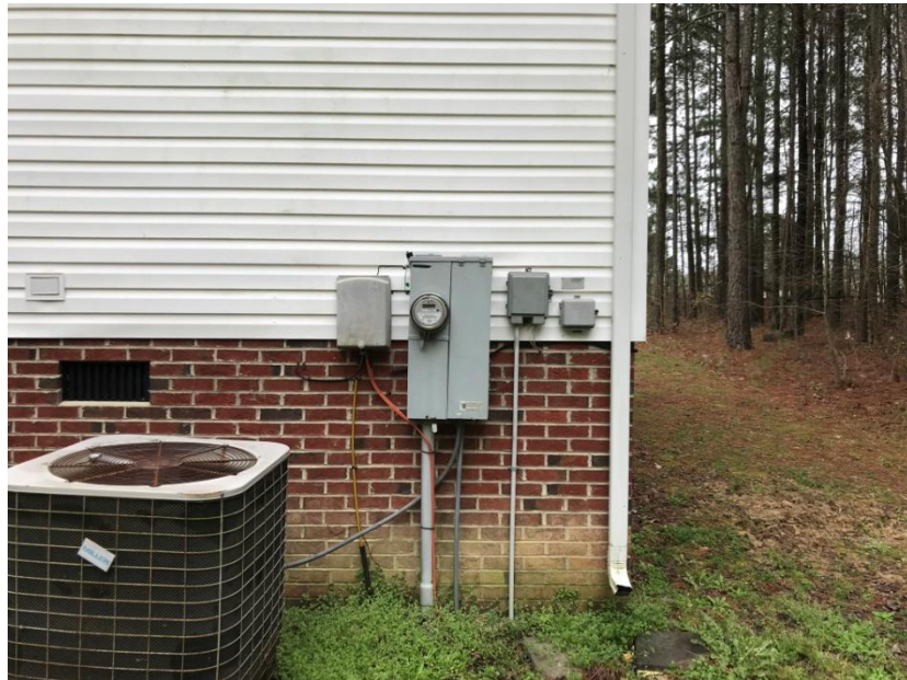
Utility service panel (rear wall left side)
