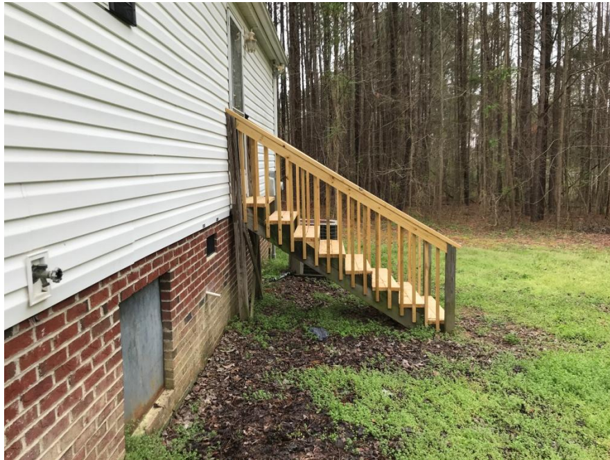
View of rear free standing detached steps.
