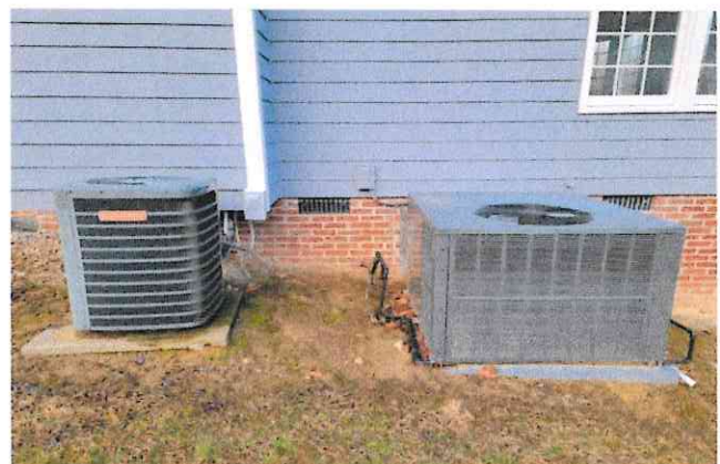
Package HVAC unit and 2nd floor A/C shown where installed outside
