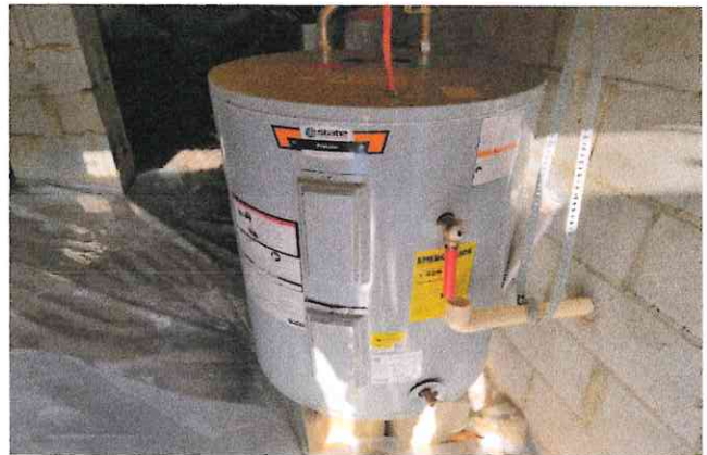
Water heater shown where installed in the crawlspace
