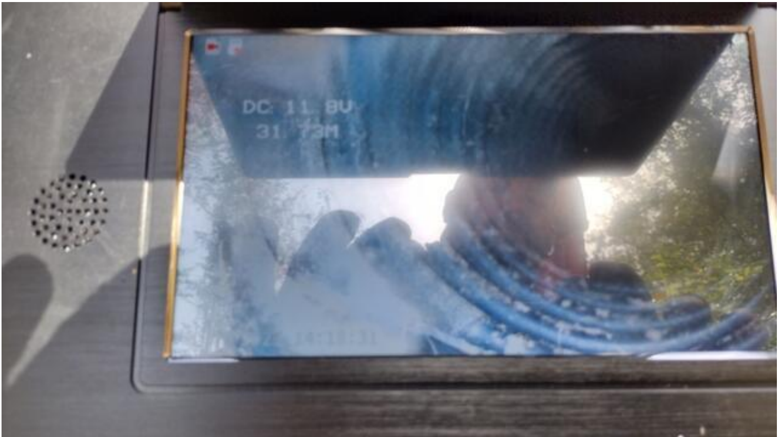
TANK DRAIN LINES – SOME ROOTS
