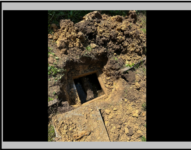
Inlet side of tank
